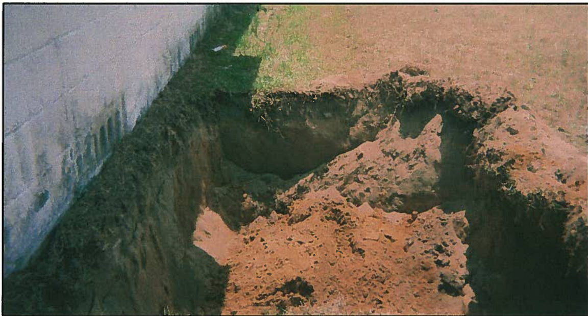
July 6, 2011 – Looking south along western side of building and suspected UST location following excavation investigation.
