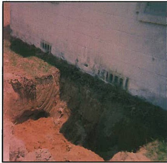
July 6, 2011 – Looking northeast at northwest corner of building and suspected UST location following excavation investigation.
