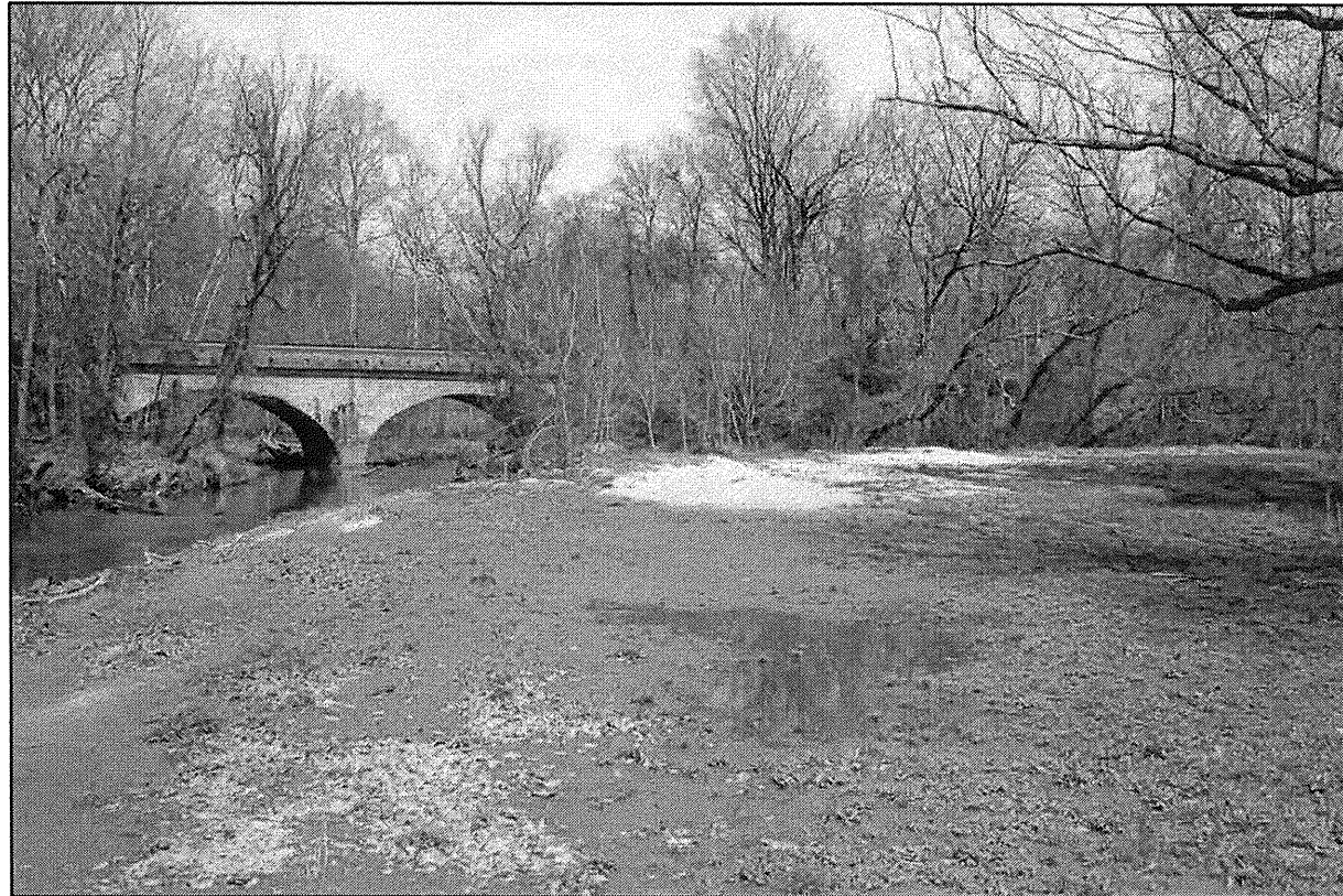
PHOTO 3: LOOKING NORTHEAST (LEFT) FROM NEAR BENT 4. EXISTING CONCRETE ARCH RAILROAD BRIDGE VISIBLE IN BACKGROUND
