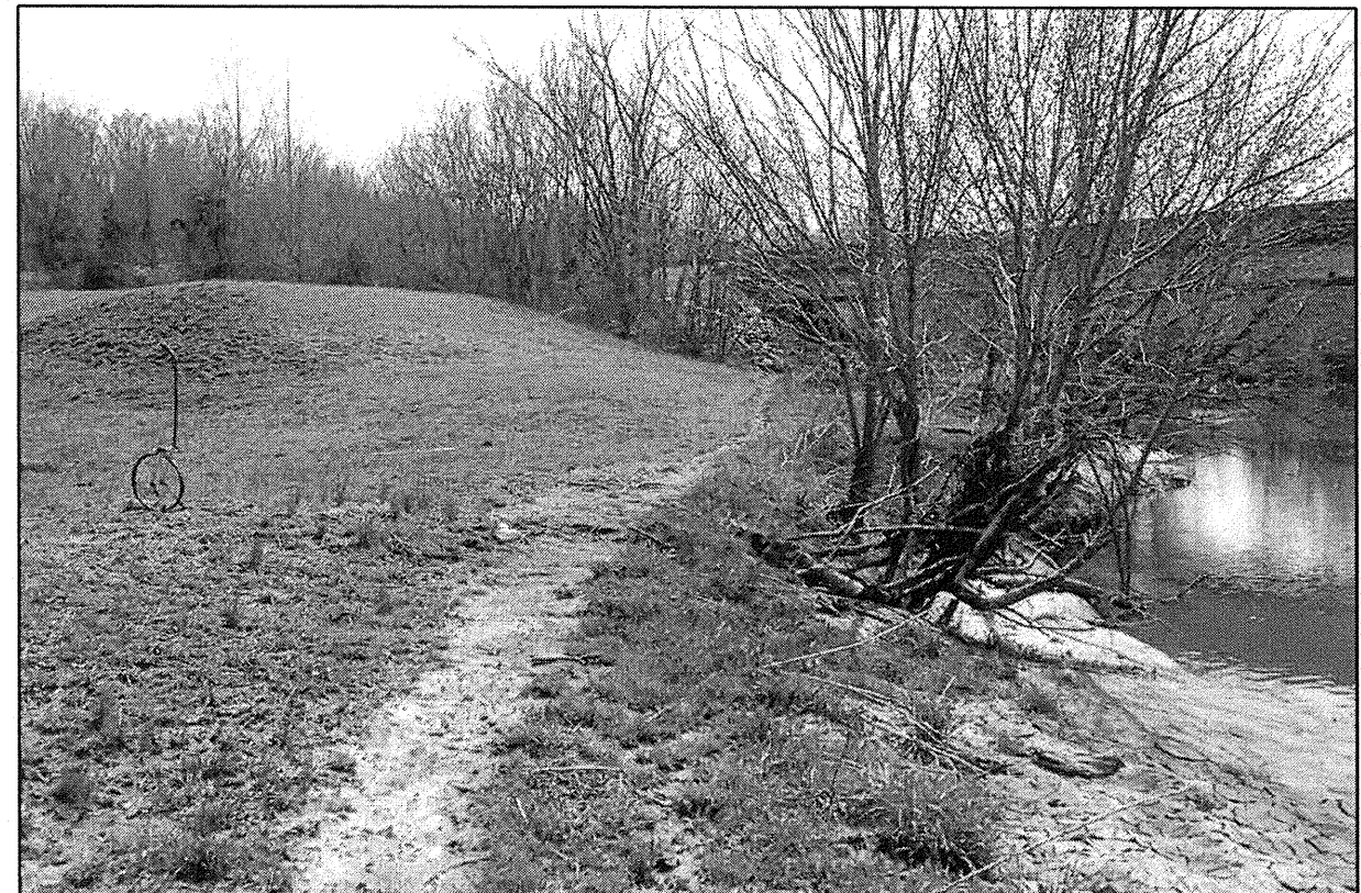
LOOKING WEST (RIGHT) FROM NEAR BENT 4. EXISTING PREVIOUS ROADWAY EMBANKMENT VISIBLE TO LEFT. EXISTING BRIDGE OVER HAMBY CREEK VISIBLE TO RIGHT IN BACKGROUND.
