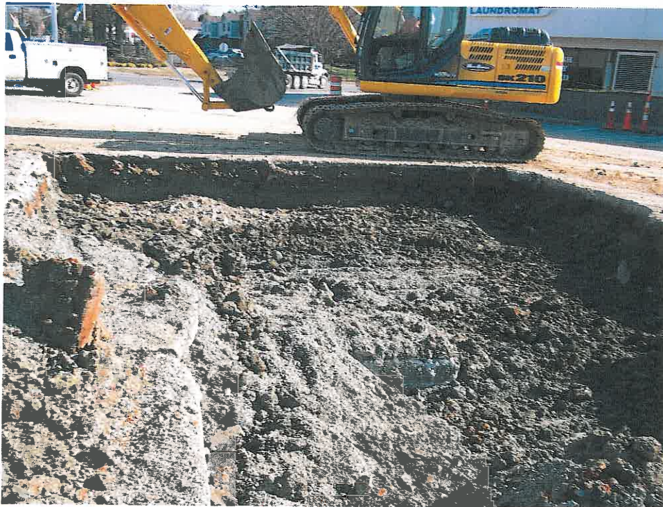
Photograph 10– View of dispenser island area.
