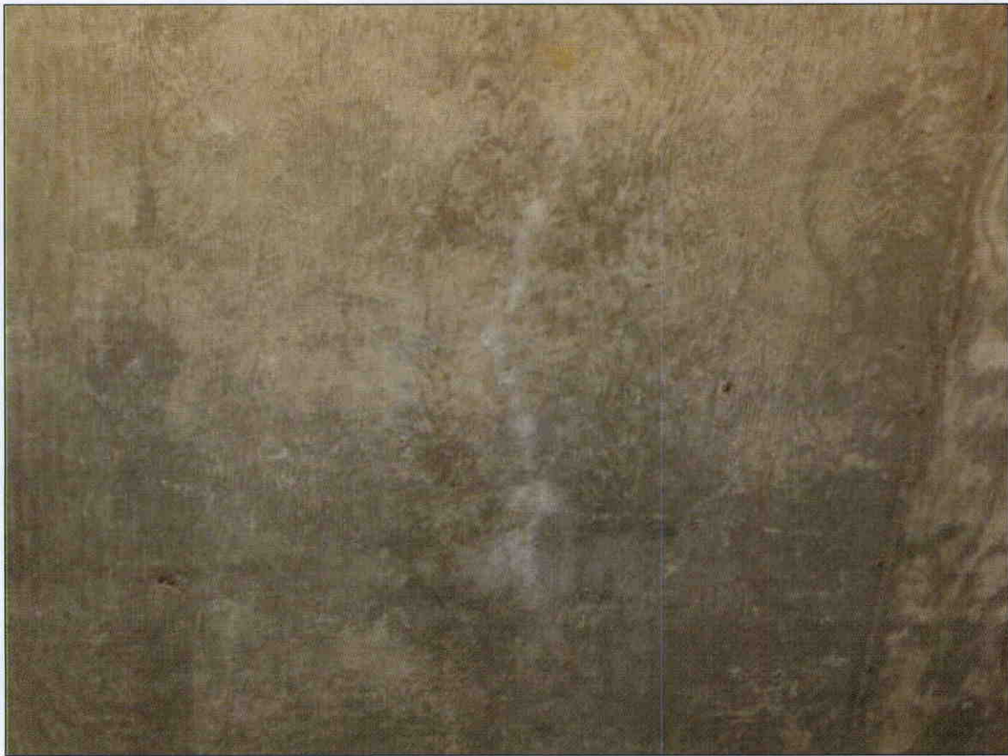
CRACKS IN THE BOTTOM OF THE DECK IN ALL SPANS
