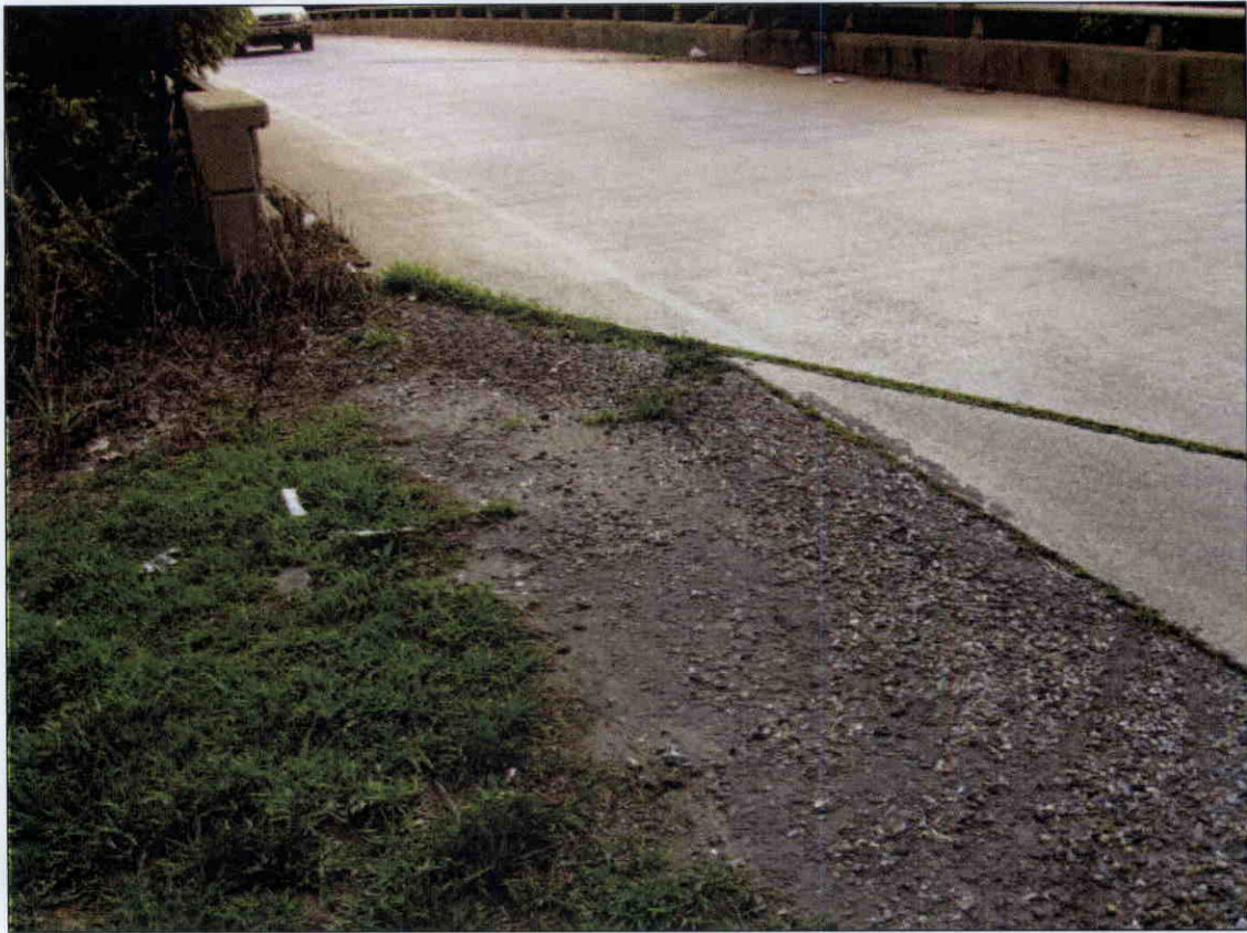
SETTLEMENT AT ALL CORNERS OF THE BRIDGE
