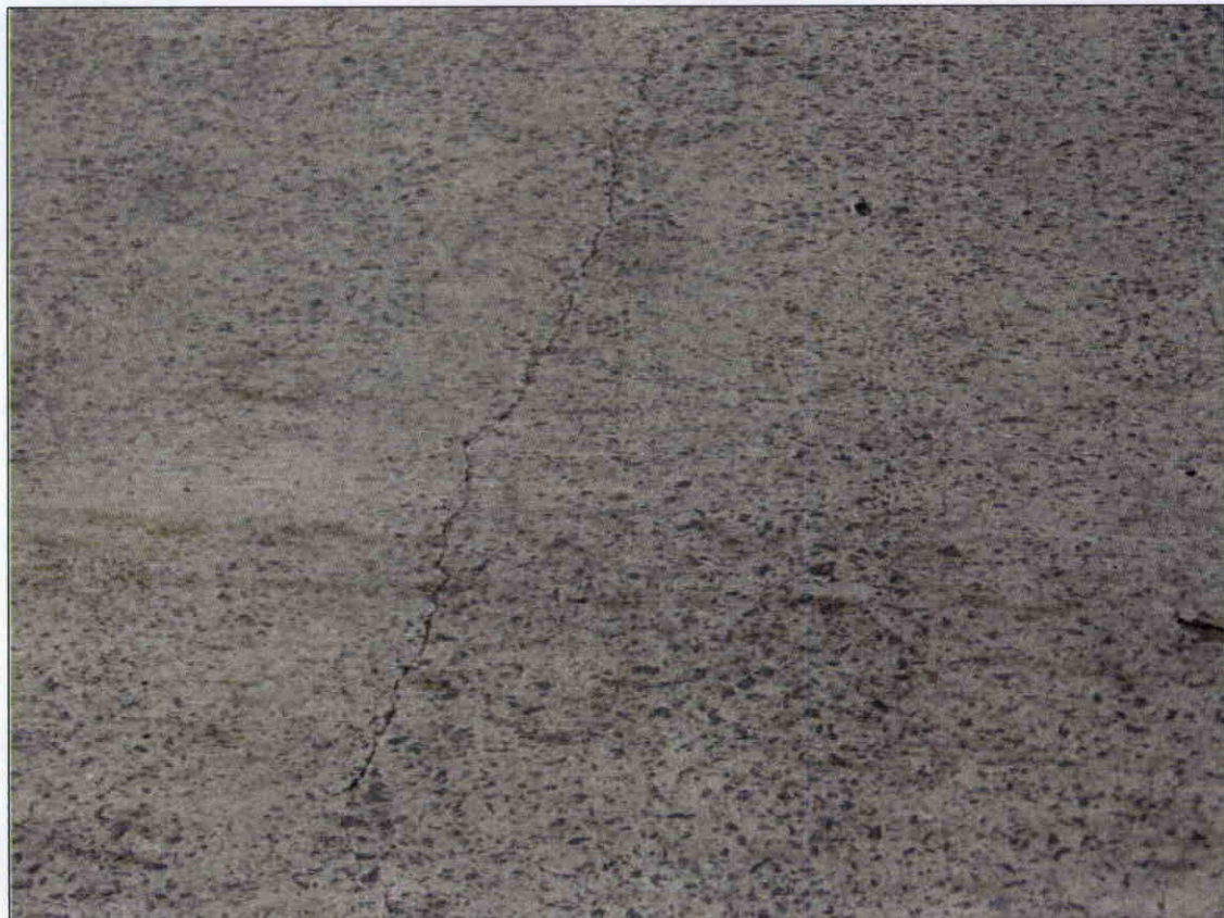
TRANSVERSE CRACKS IN ALL SPANS
