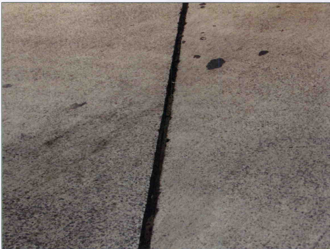
ALL EXPANSION JOINTS LOW AND LEAKING
