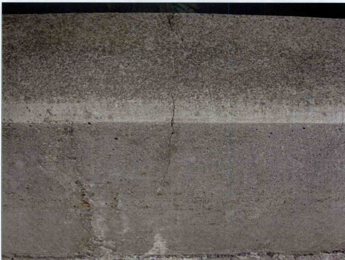
VERTICAL CRACKS IN BOTH PARAPET WALLS
