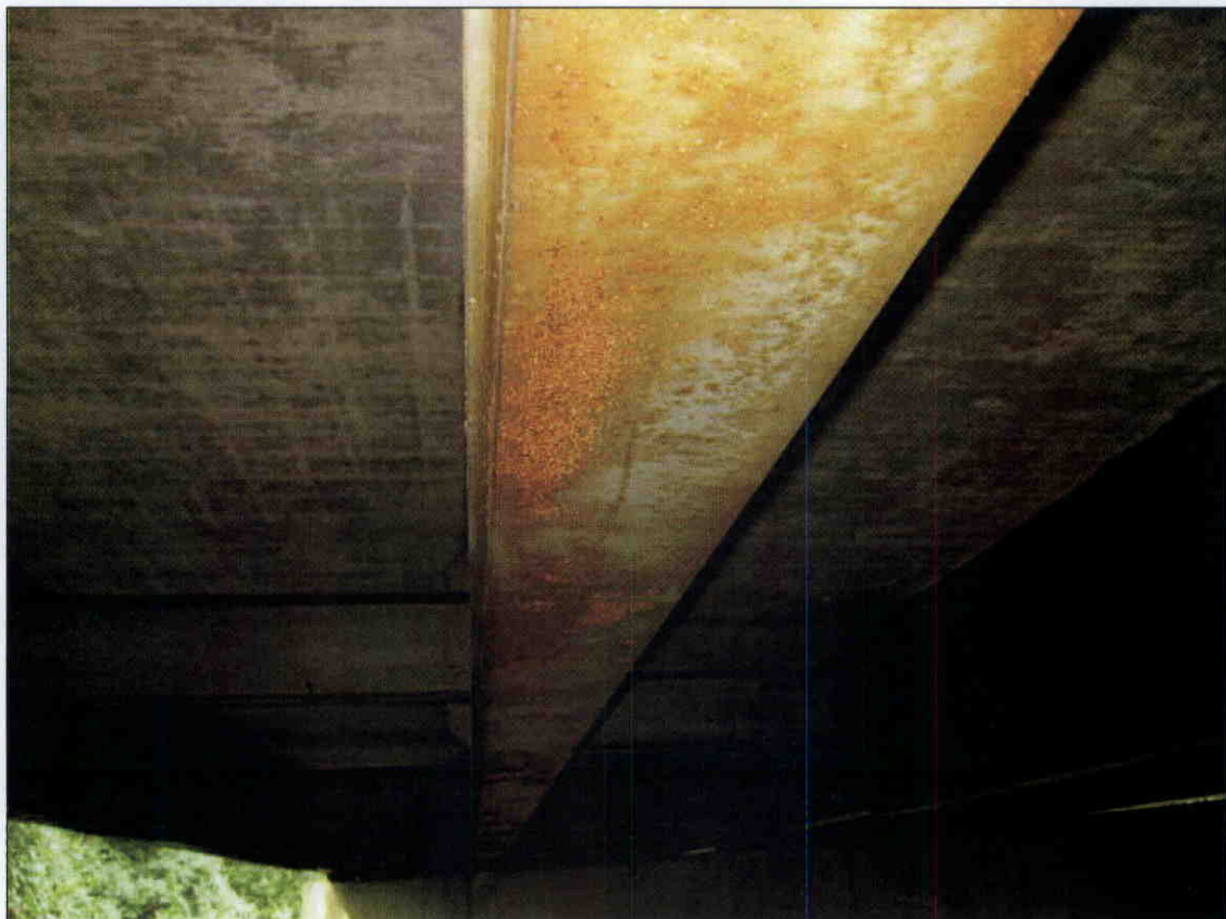
SURFACE RUST ON BOTTOM FLANGES IN ALL SPANS
