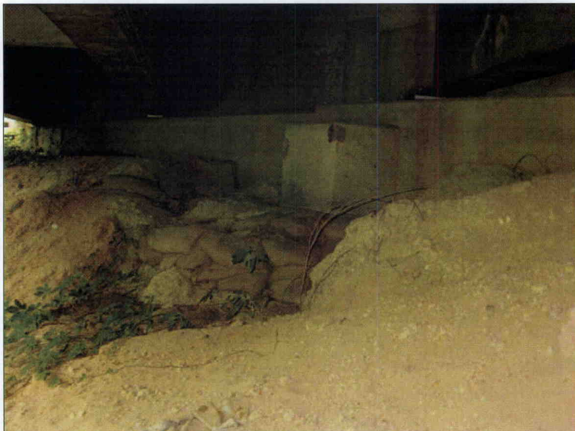
WASH ON ABUT 2 EARTH SLOPE
