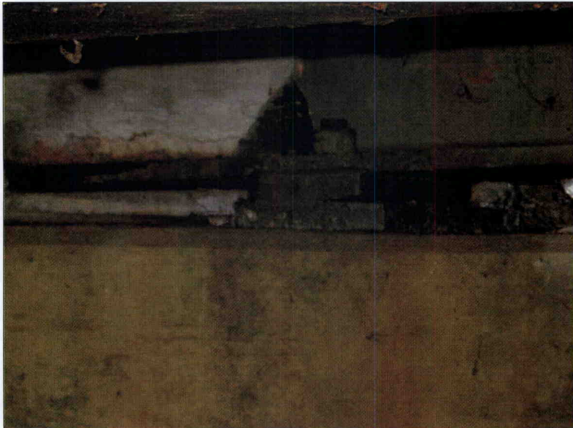
RUST ON THE BEARINGS AND BEAM ENDS AT THE ABUTMENTS
