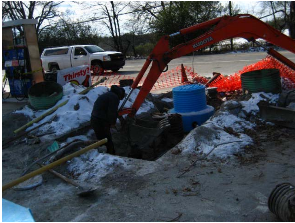
Parcel 199 – S.L. Jarvis & M.C. Jarvis Property, looking northwest. Photo shows location of known UST on north side of building during repairs by others.
