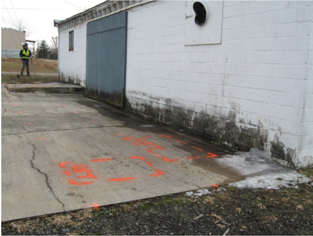
Parcel 98 – Steven Joseph Whitley Property, looking south. Photo shows approximate marked location of the probable USTs on the east side of the property.
