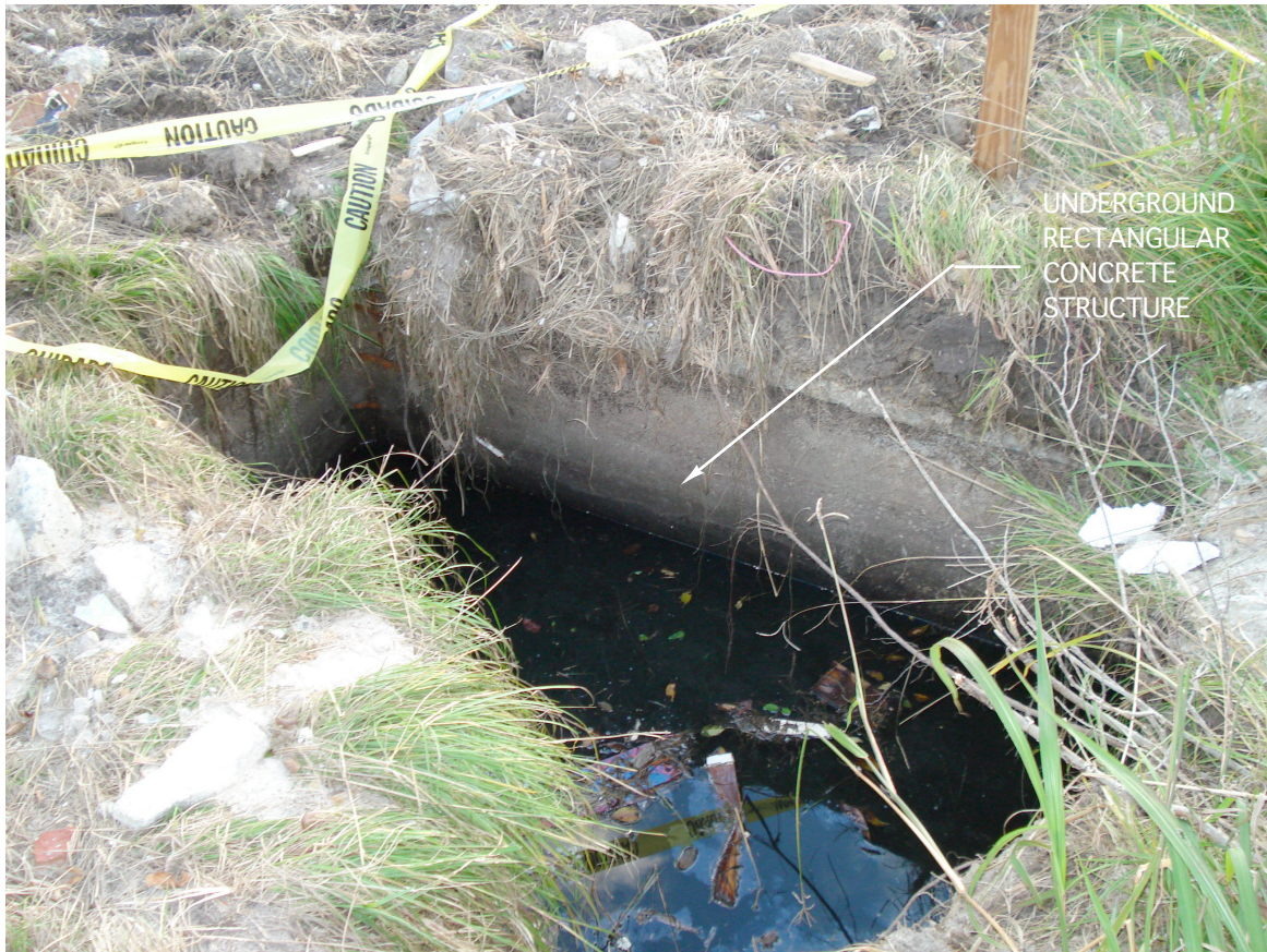
Photograph 3: View looking south at underground rectangular concrete structure encountered by NCDOT demolition contractor. Two pipes, oriented northwest-southeast, extend from each end of structure. Apparent sheen shown on water surface is believed to be due to naturally occurring bacteria, not petroleum.
