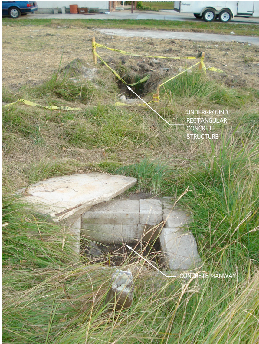
Photograph 2: View looking southeast at underground concrete structure encountered by NCDOT demolition contractor.
