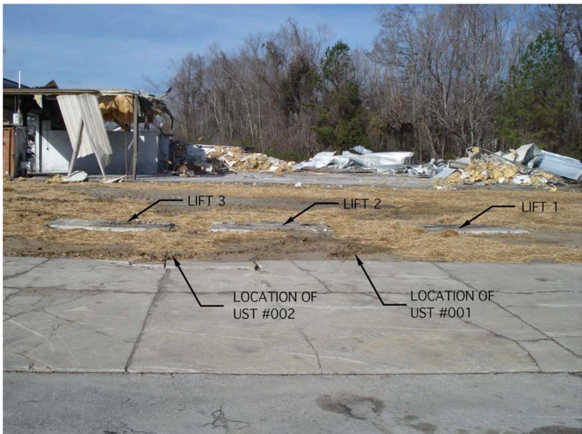
Photograph 2: View looking west at hydraulic Lift 1, Lift 2, and Lift 3, and locations of hydraulic fluid USTs #001 and #002 prior to removal and after demolition of Piney Green Tire & Auto building.
