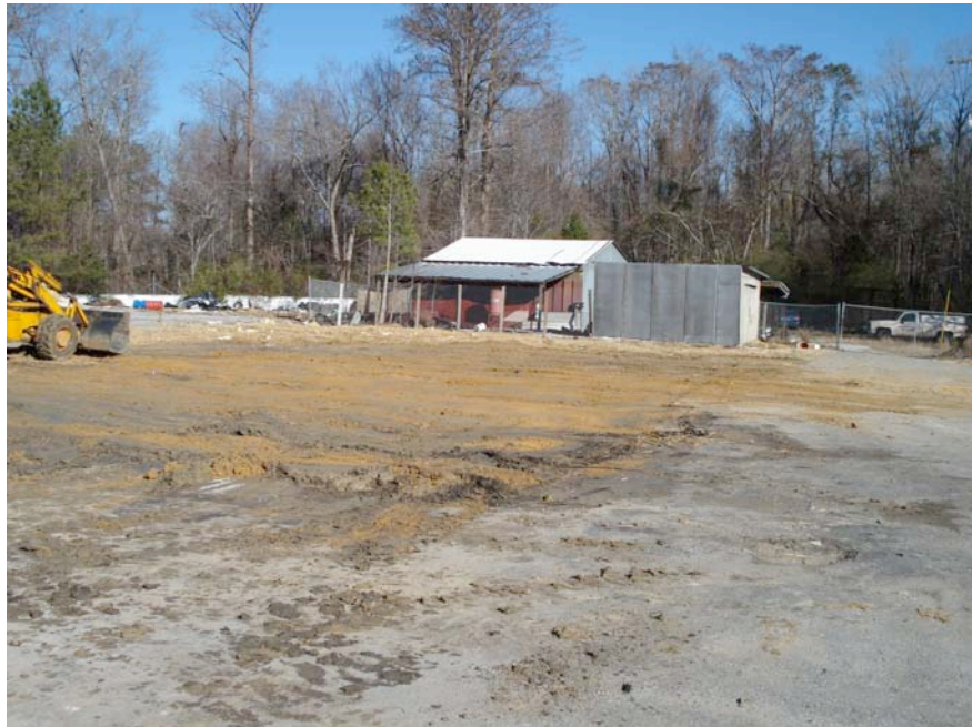
Photograph 8: View looking north at backfilled and compacted hydraulic lift and hydraulic fluid UST removal area.
