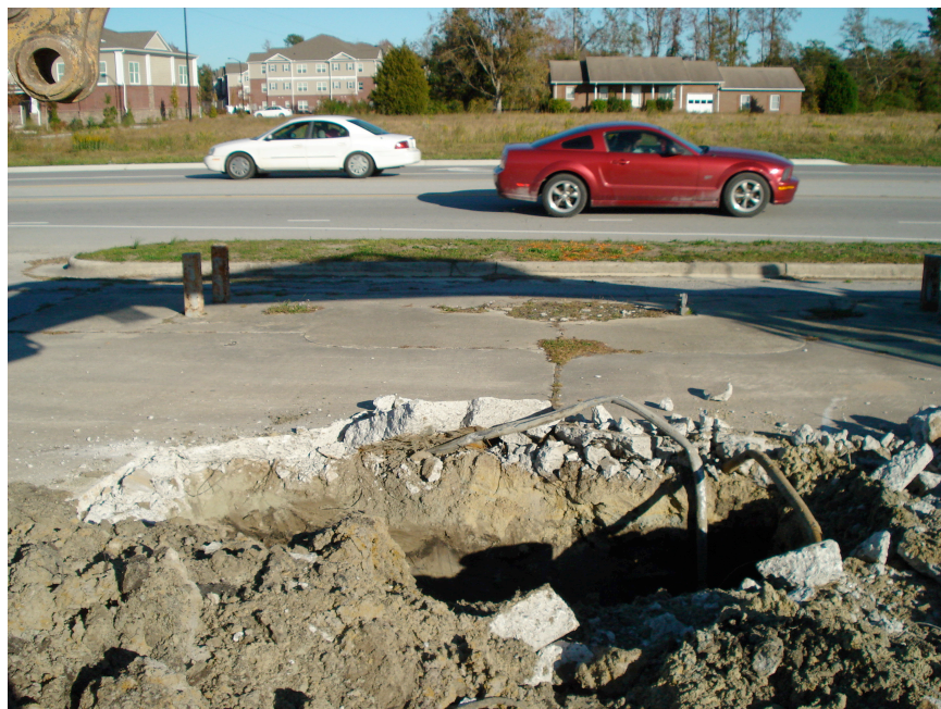
Photograph 2: View looking east at excavation, showing some of piping encountered beneath concrete.
