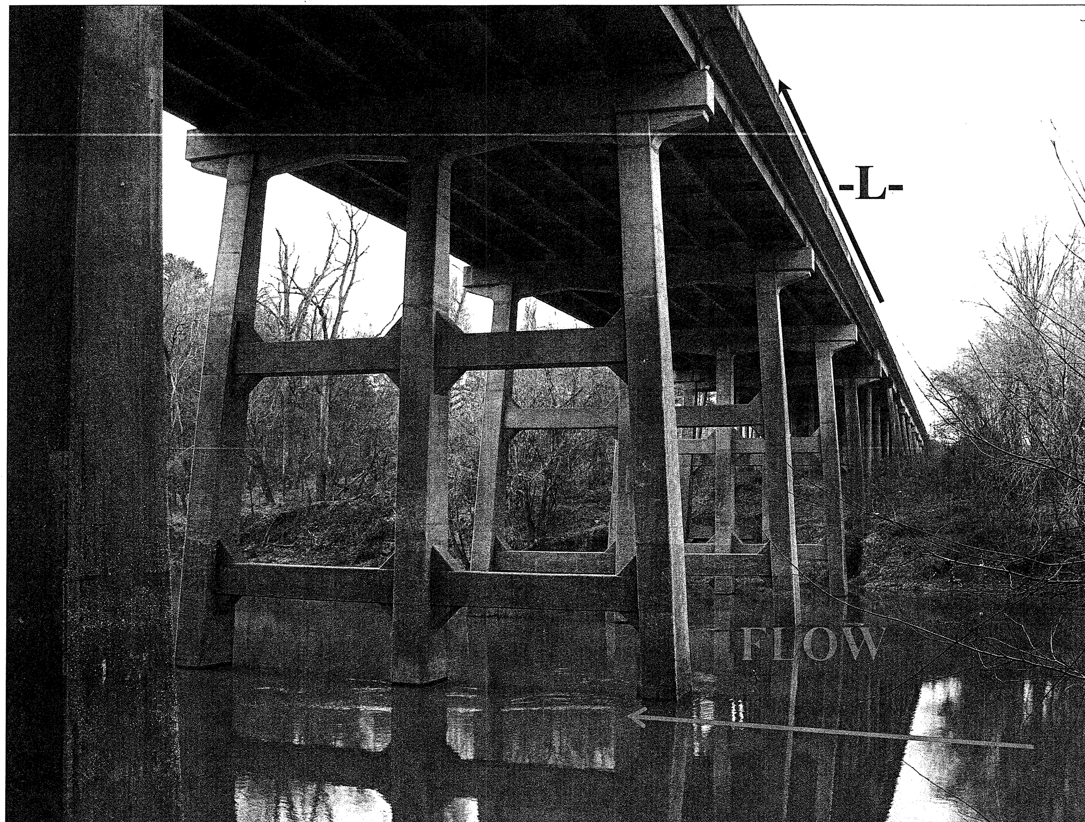
Bridge No. 85 on -L- (US 301/I-95 Bus. Loop) over -Y1- (SR 1738), -Y2- (SR 1741) and Cape Fear River
