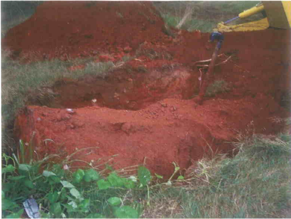
Photograph 1: Removal of UST at Parcel 9, 121 Hibriten Drive (view is to the east).
