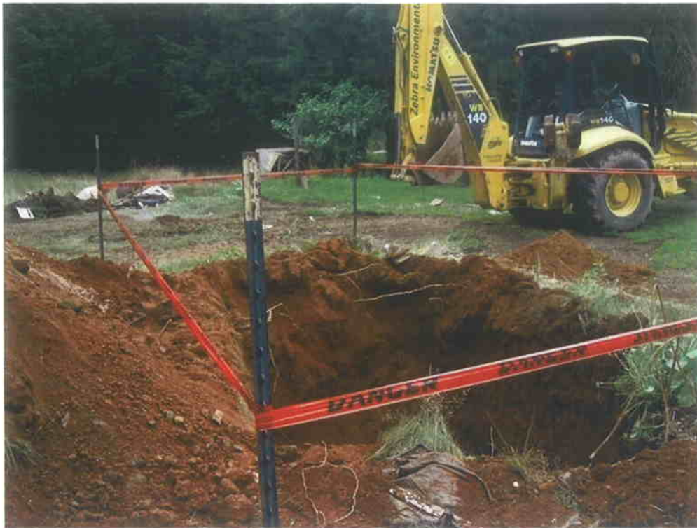
Photograph 3: View of over-excavation at Parcel 9, 121 Hibriten Drive, (view is to the southwest).
