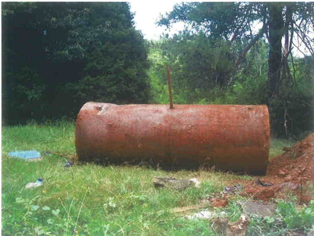
Photograph 2: Removal of UST at Parcel 9, 121 Hibriten Drive (view is to the east).
