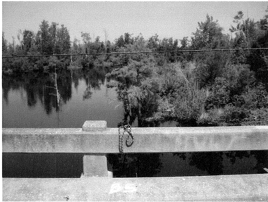
Photograph No. 10: This photograph was taken from the right side of the -L- alignment, looking west, across proposed Interior Bent No. 5.
