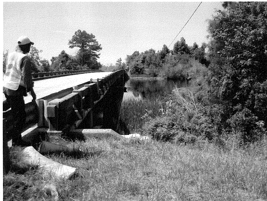
Photograph No. 14: This photograph was taken at proposed End Bent No. 2, along the -L- alignment, looking south.
