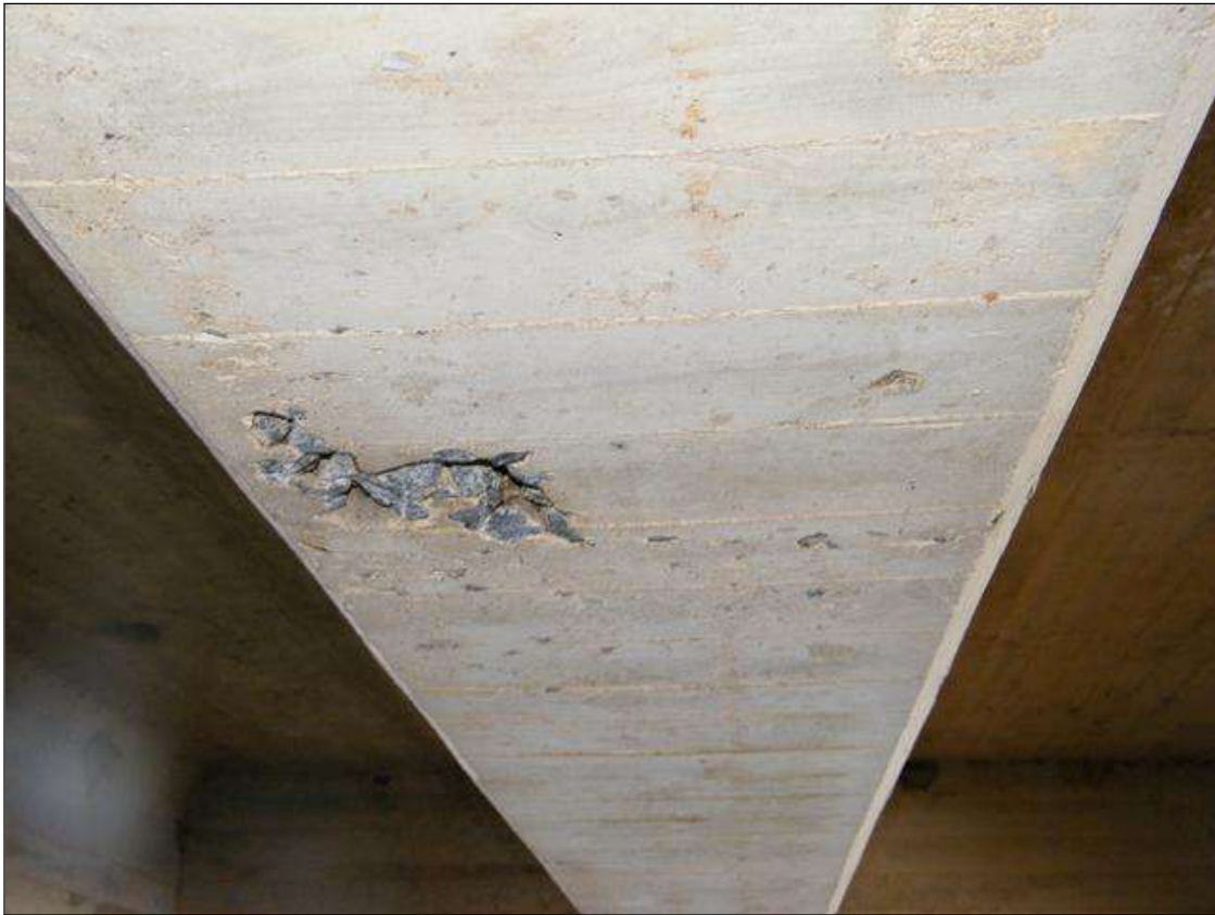
GIRDER 2 IN SPAN 1 HAS 2 INCH DEEP AREA OF HONEYCOMBING NEAR MID-SPAN .
