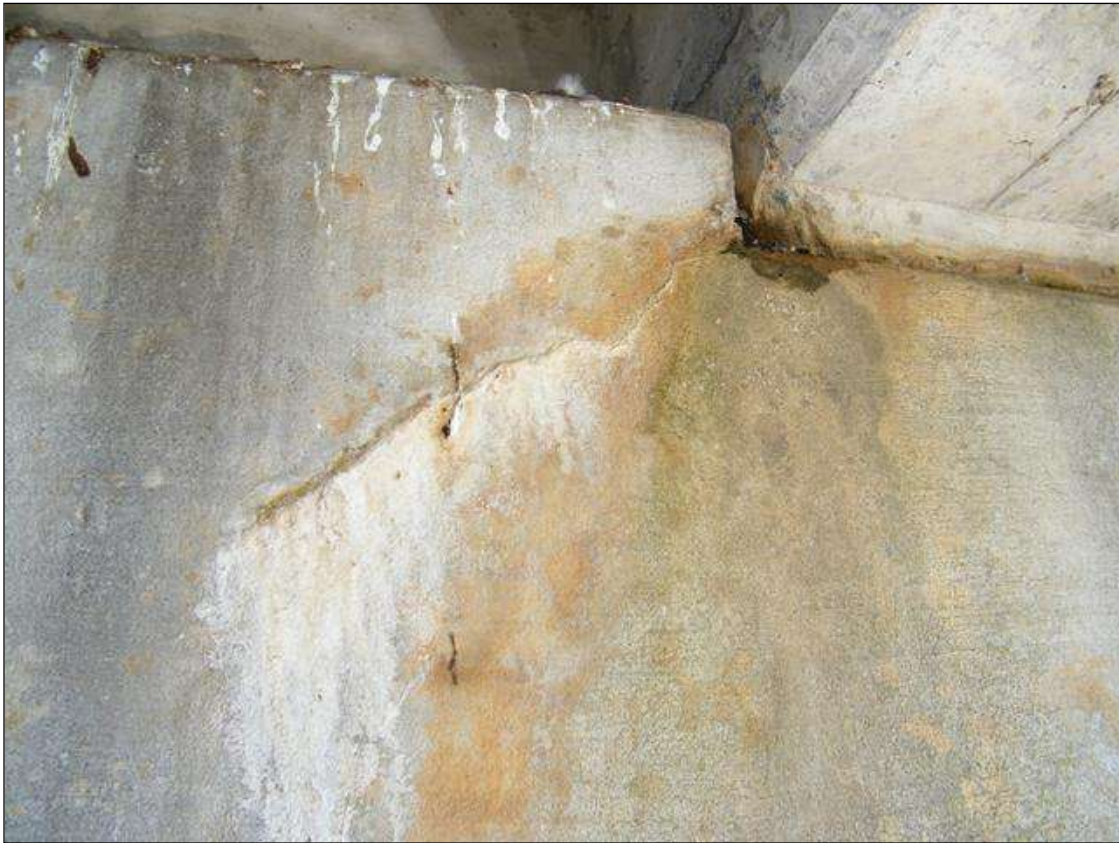
PIER 1 CAP ON SOUTH FACE HAS DIAGONAL EFFLORESCENCE CRACKS AT STEP-UP LEFT OF GIRDER 4
