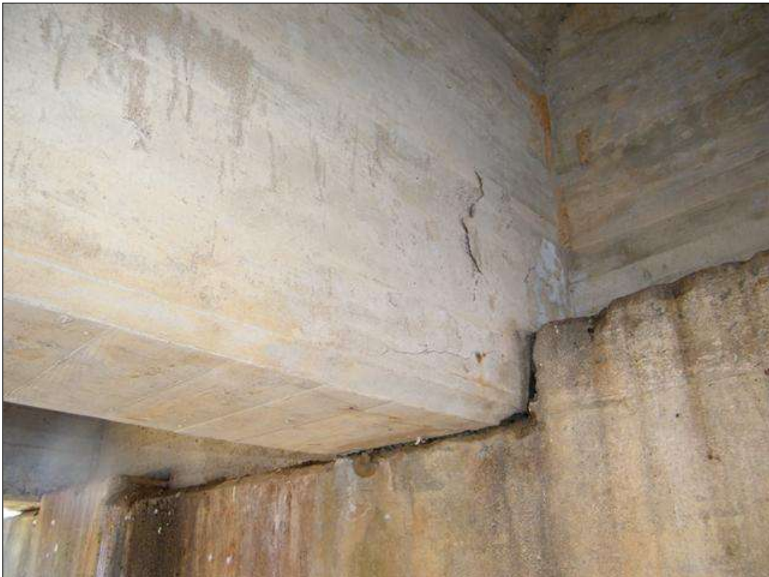
GIRDER 3 IN SPAN 2 IS DELAMINATED ON LEFT SIDE AT PIER 1 .
