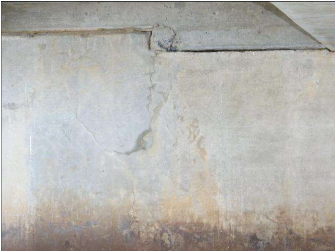
ABUTMENT 1 CAP MAP CRACKING ON FACE AT BAY 3
