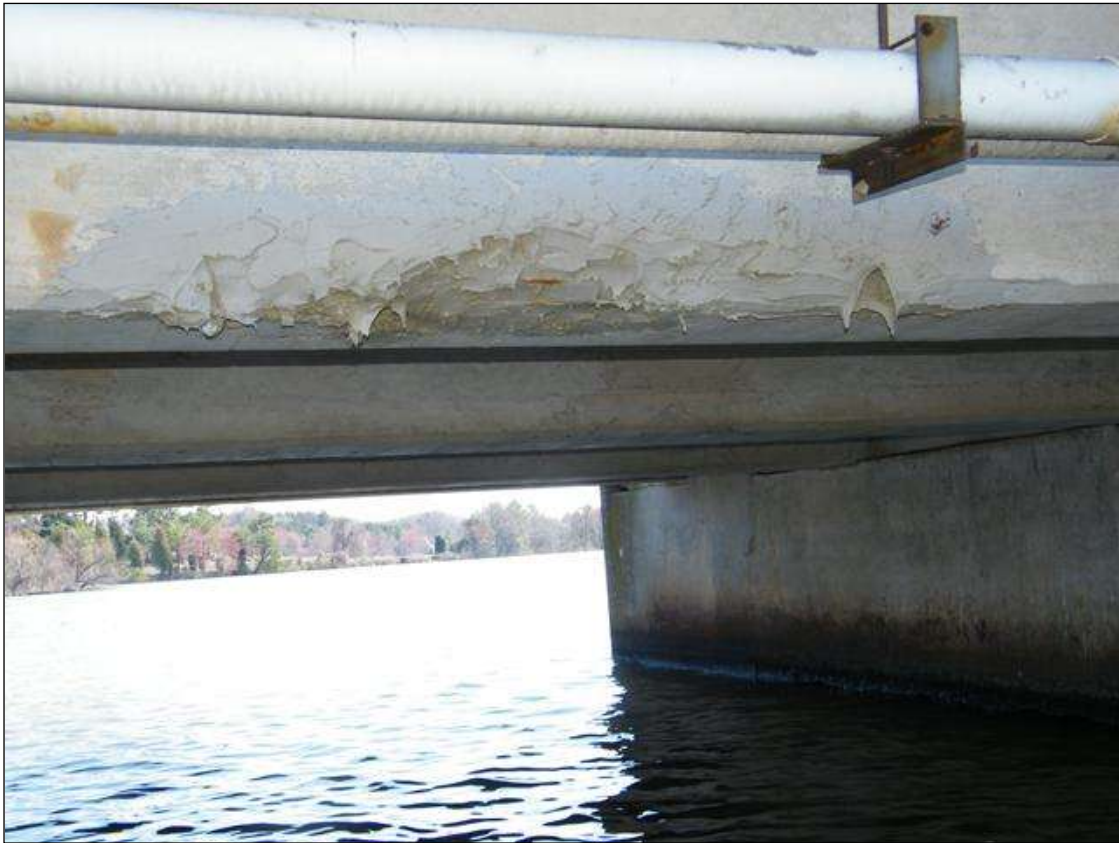
GIRDER 1 IN SPAN 1 HAS A CONCRETE REPAIR, 10 FEET FROM ABUTMENT 1.
