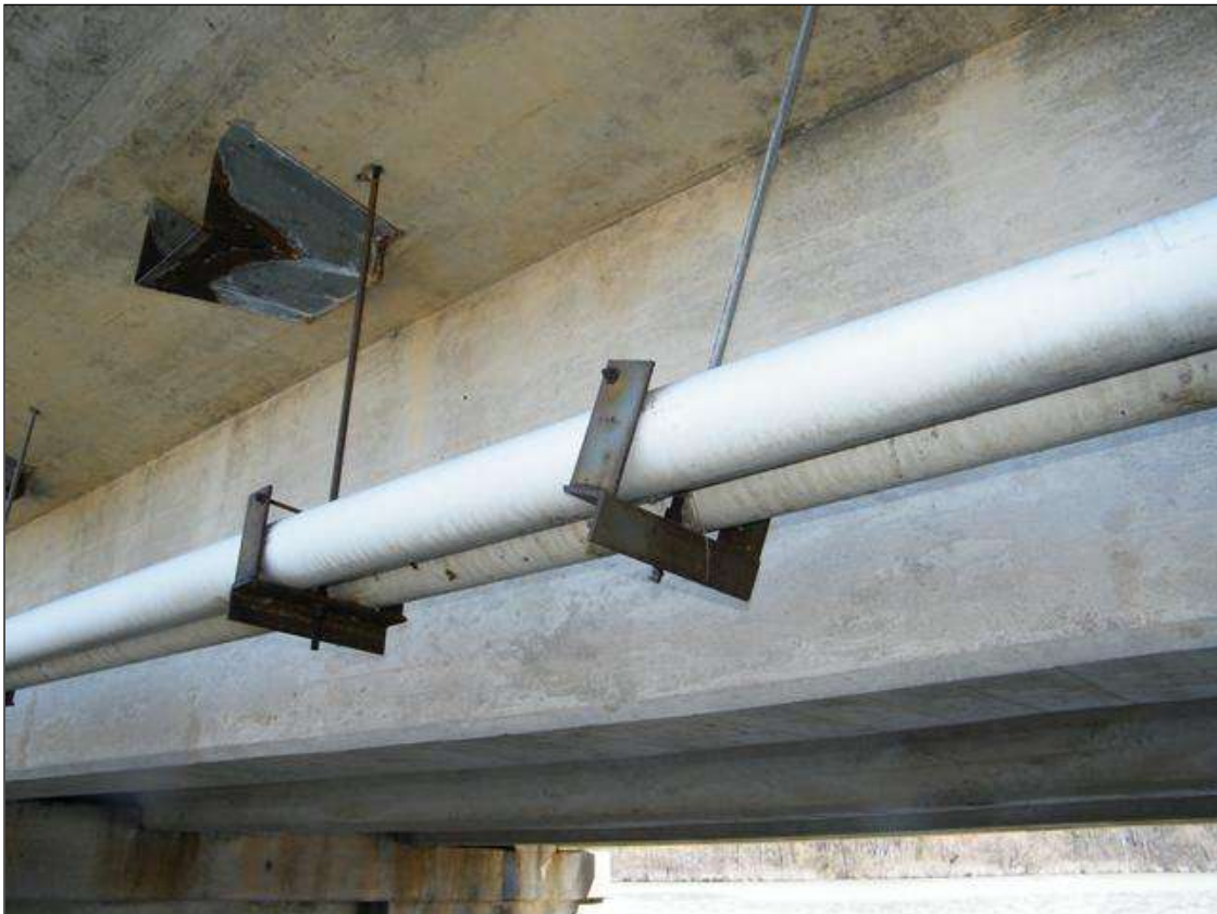
UTILITY, 2 LINES OF 5" DIAM. PVC ALONG THE LEFT OVERHANG.
