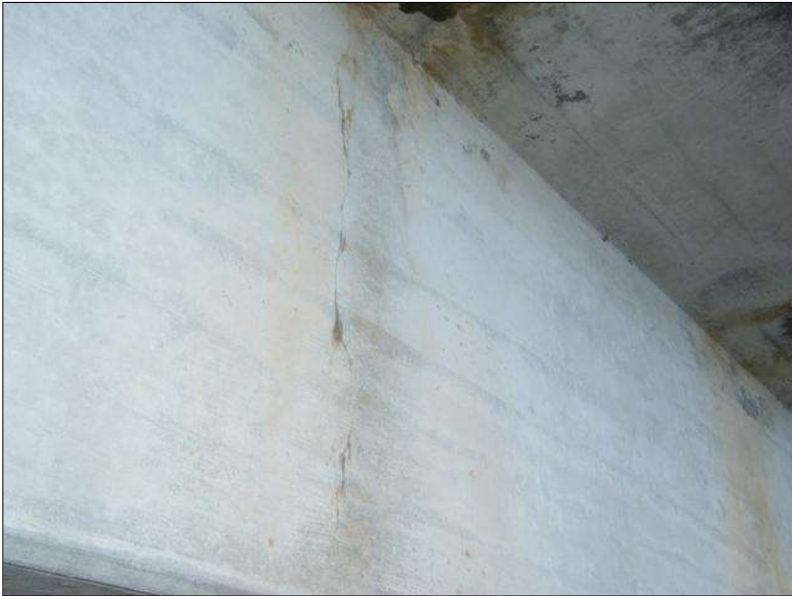
GIRDER 4 IN SPAN 3 HAS VERTICAL H/L CRACK ON RIGHT SIDE FROM TOP TO BOTTOM NEAR MID-SPAN AT 10 FEET FROM ABUTMENT 2 .
