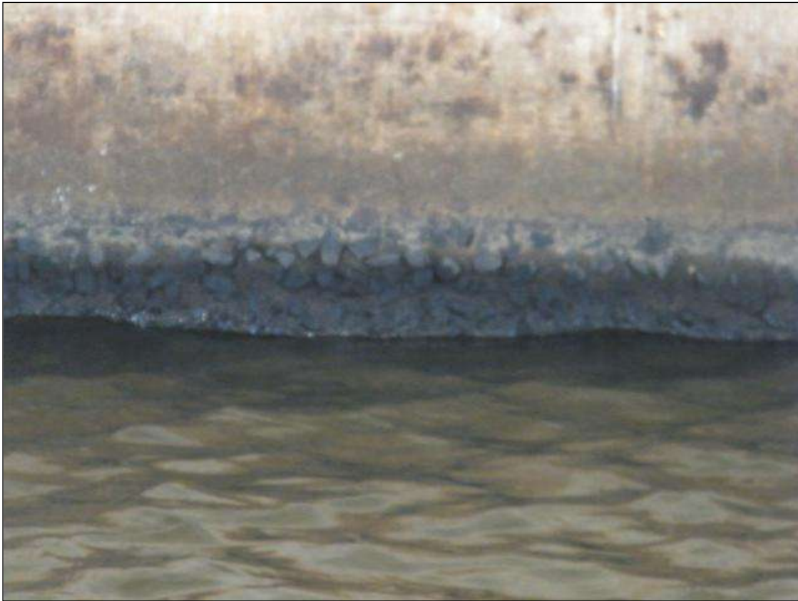
ABUTMENT 1 BREASTWALL AND COLUMNS ARE PITTING UP TO 1" DEEP ALONG THE WATERLINE.
