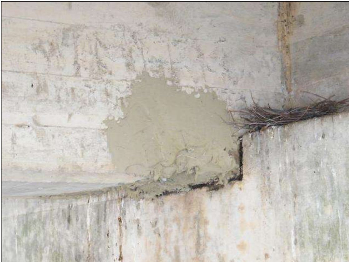
GIRDER 2, SPAN 3 HAS A CONCRETE REPAIR ALONG BOTTOM AT PIER 2
