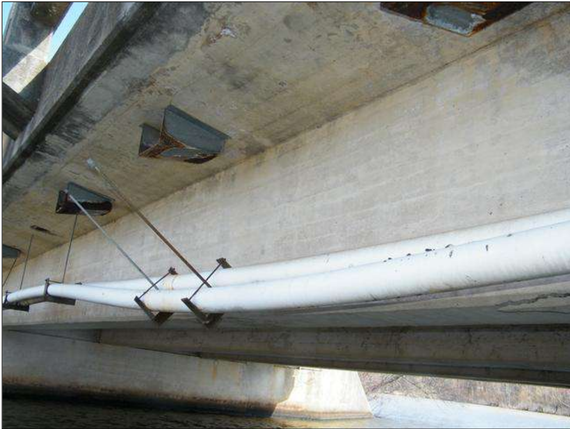
UTILITY BRACKETS BROKEN IN SPAN 3, UTILITY LINES SAGGING .
