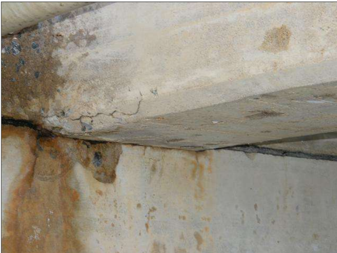
GIRDER 1, SPAN 3 HAS A 1/8" LONGITUDINAL CRACK FROM ABUTMENT 2 BACK 6" ALONG BOTTOM.
