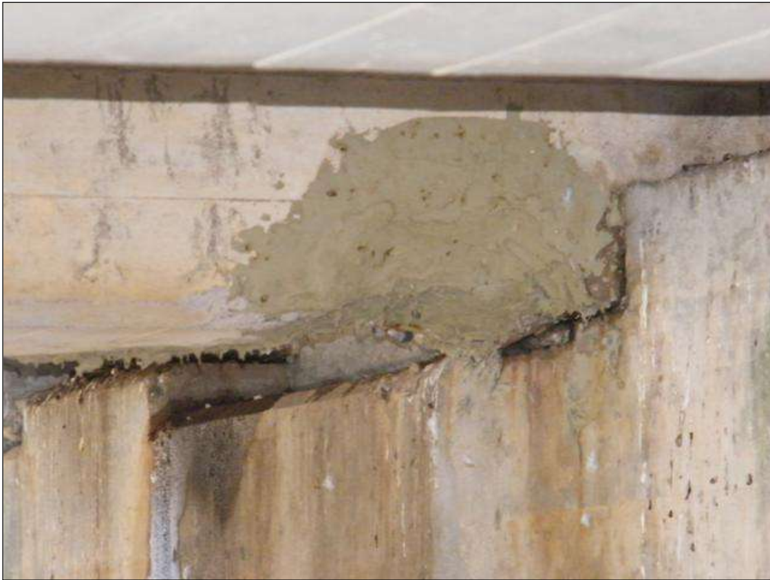
GIRDER 3, SPAN 3 HAS A CONCRETE REPAIR ALONG BOTTOM AT PIER 2
