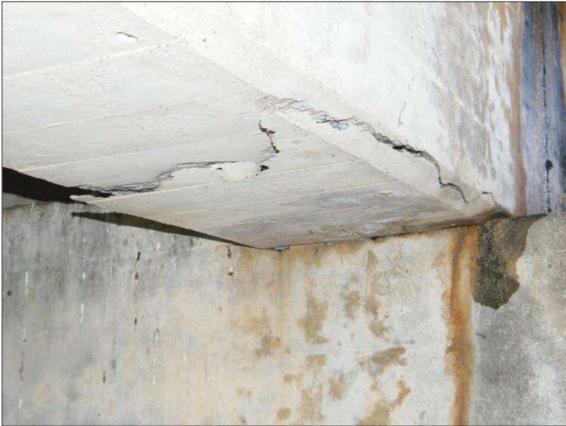
GIRDER 1, SPAN 3 IS DELAMINATED 1" DEEP ALONG BOTTOM FROM PIER 2 BACK 1' LONG X WIDTH.
