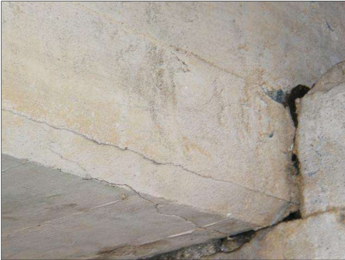
GIRDER 2 IN SPAN 2 DELAMINATED ON LEFT SIDE AT PIER 1 .
