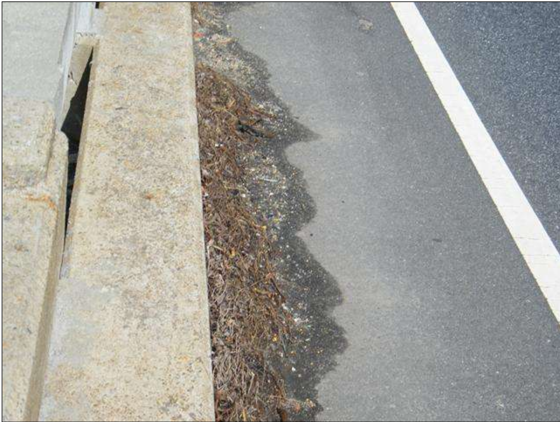
DIRT ALONG CURBS PARTIALLY BLOCKING DRAIN HOLES
