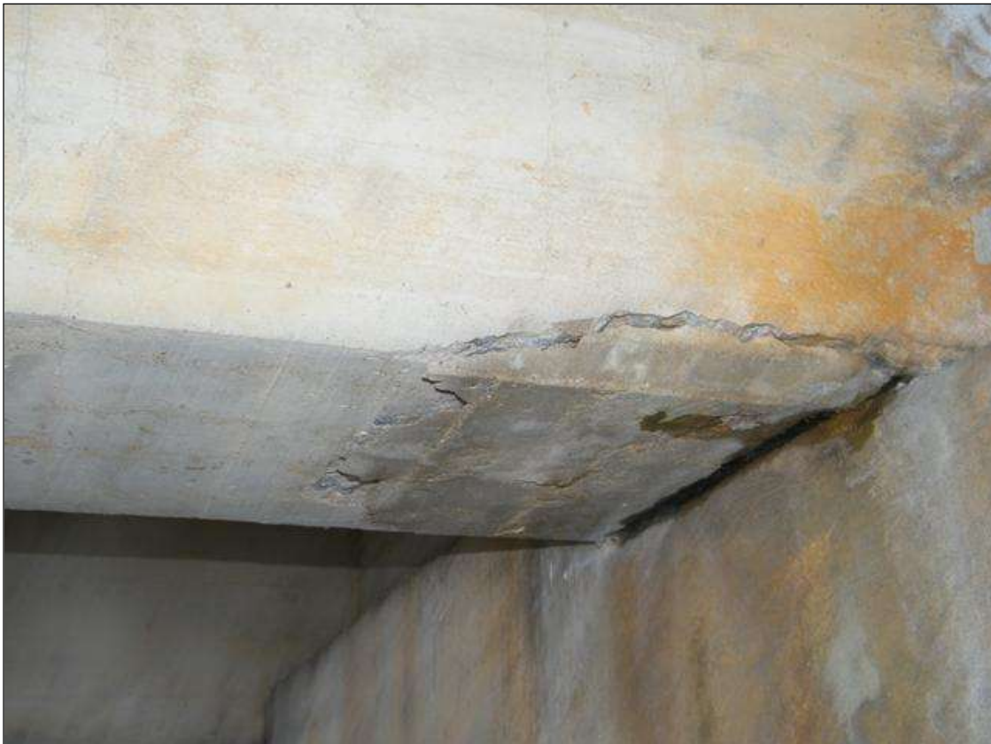
GIRDER 3 IN SPAN 1 HAS DELAMINATED AREA ALONG BOTTOM AT PIER 1 .
