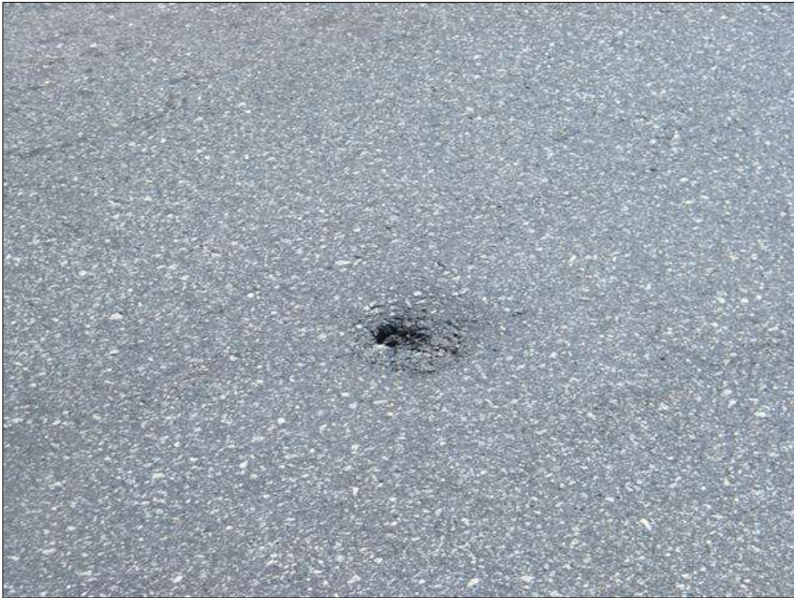
DECK WAS CORED IN SPAN 3, HOLE IN WEARING SURFACE.
