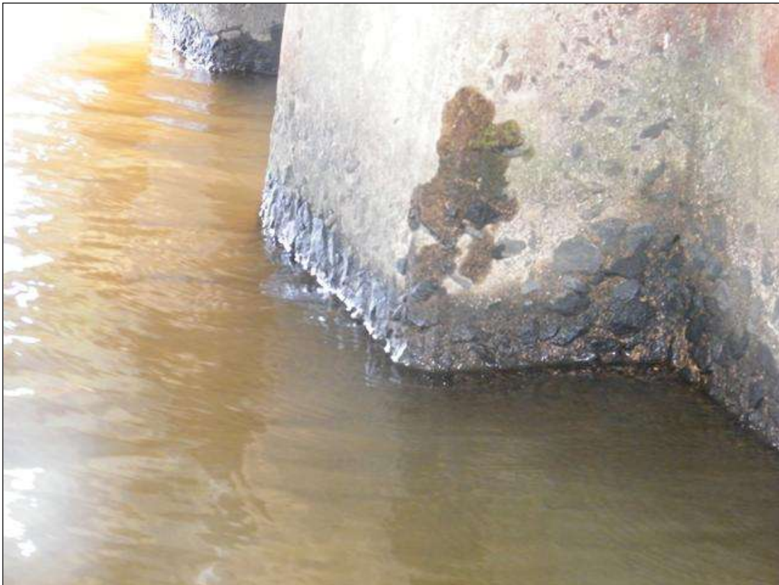
COLUMNS AT PIER 1 ARE PITTING UP TO 1" DEEP AT THE WATERLINE
