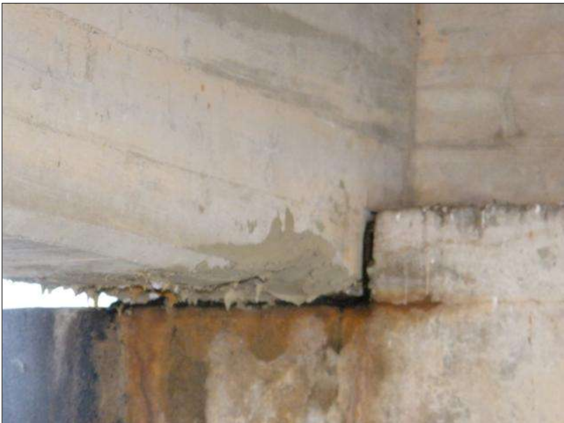
GIRDER 1, SPAN 1 HAS A CONCRETE REPAIR AT PIER 1.
