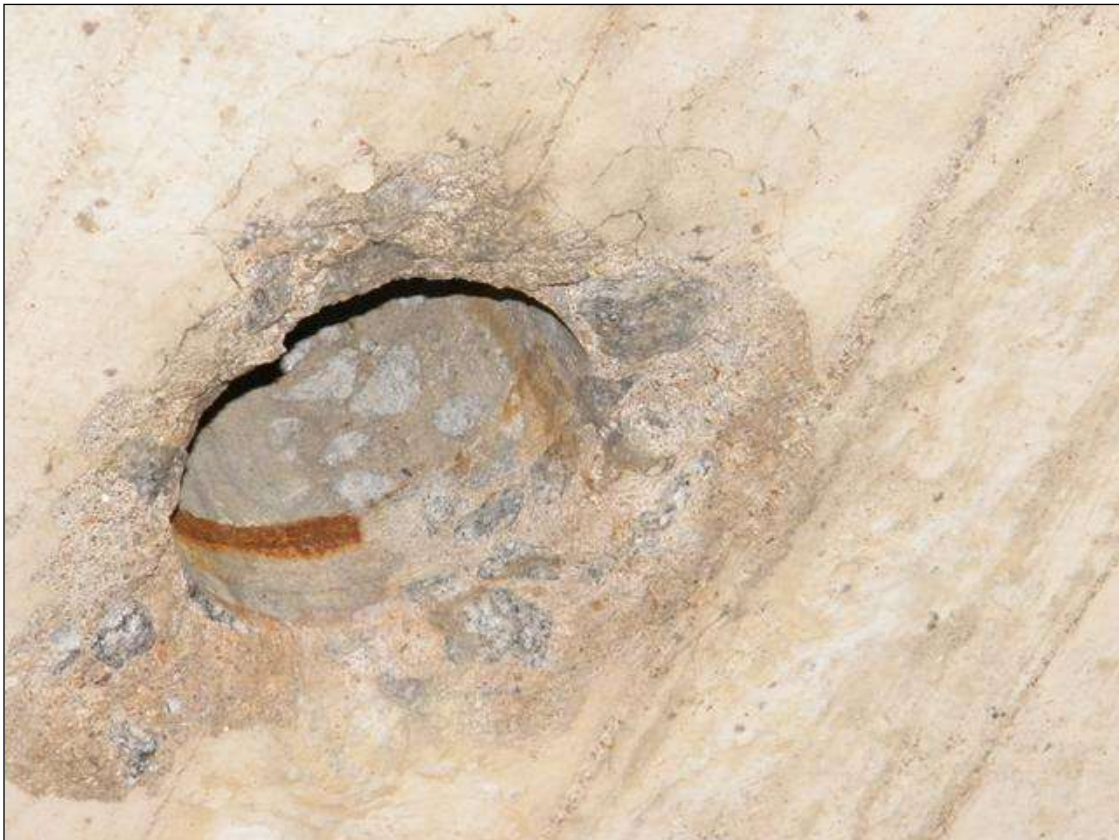
DECK HAS BEEN CORED IN SPAN 3, BAY 1
