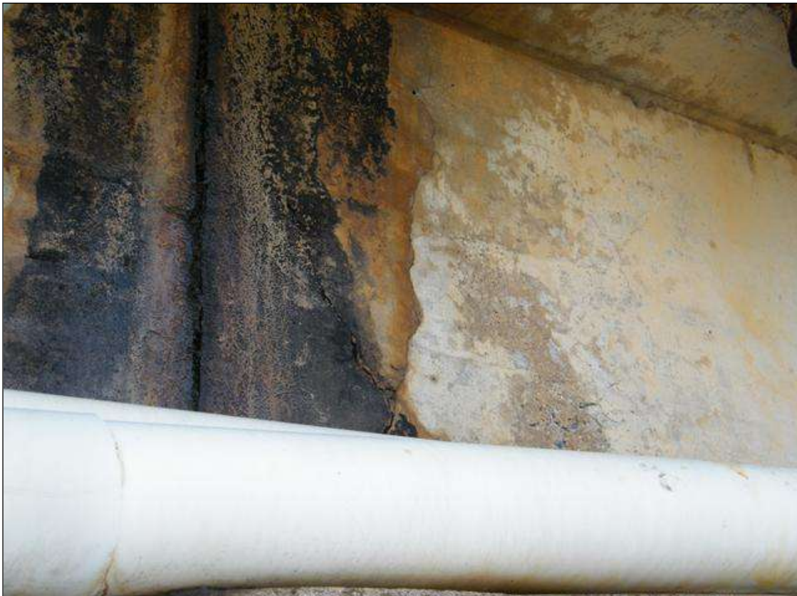
GIRDER 1 IN SPAN 2 HAS 1/2 CRACK ON RIGHT SIDE AT PIER 2 .
