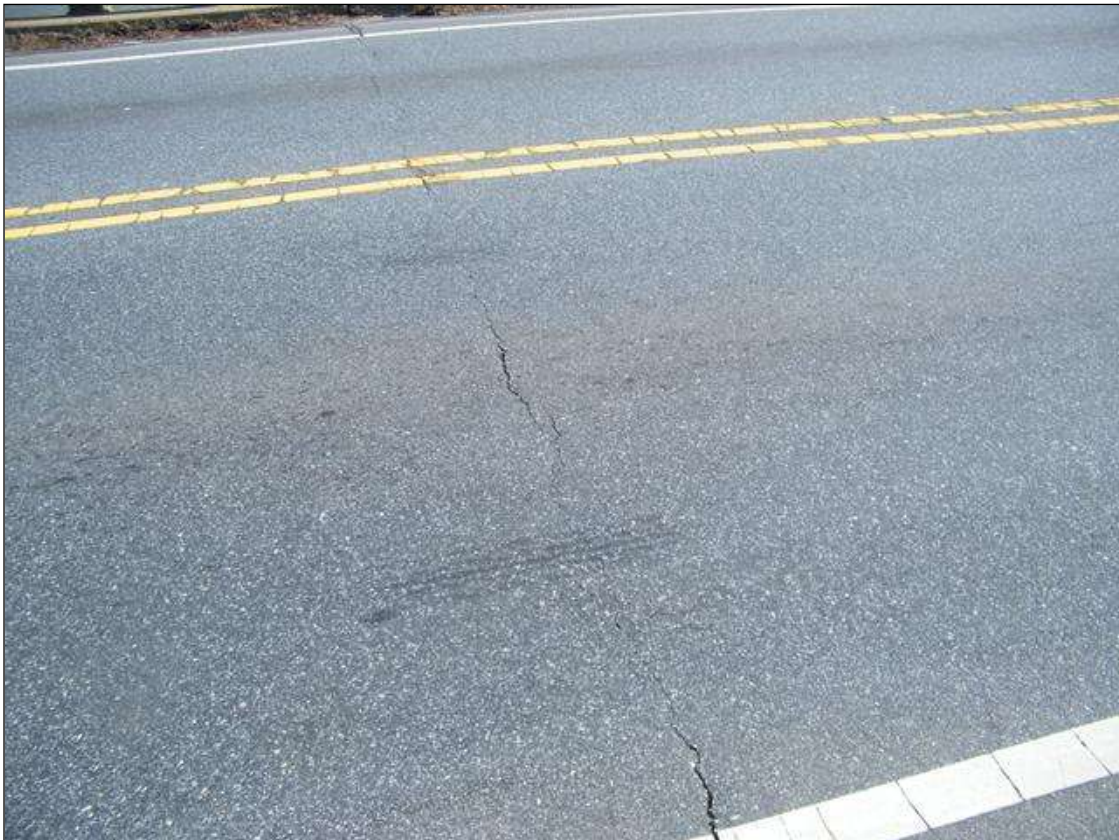
WEARING SURFACE CRACKED AT PIERS AND ABUTMENTS.
