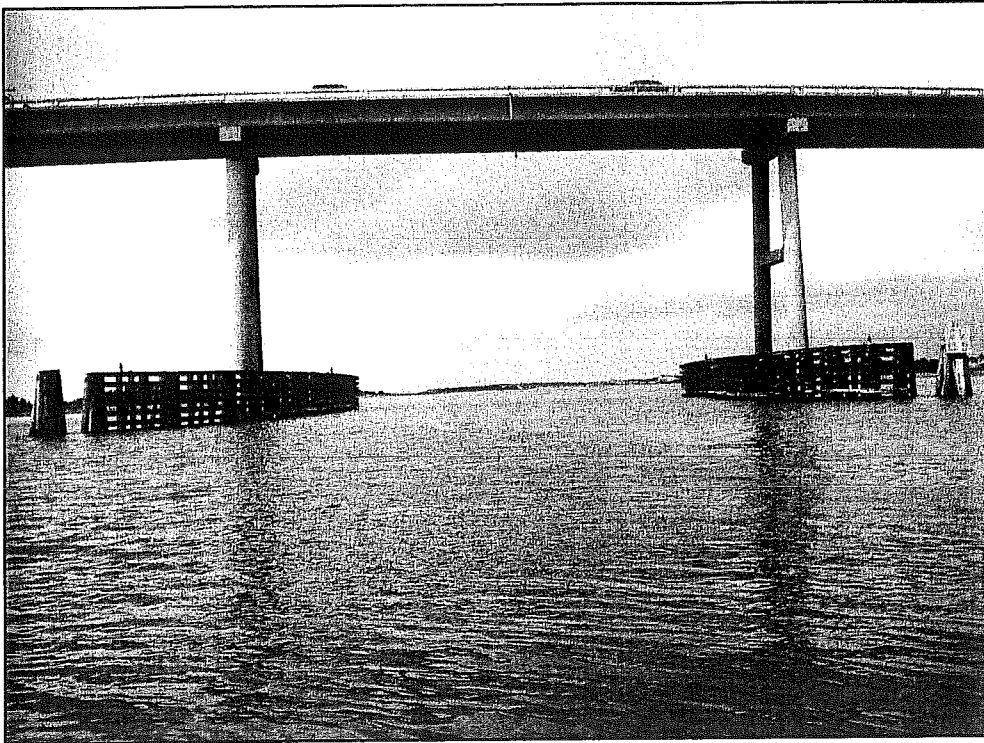
EAST OF BRIDGE #6 FACING WEST NORTH FENDER ON RIGHT SOUTH FENDER ON LEFT
