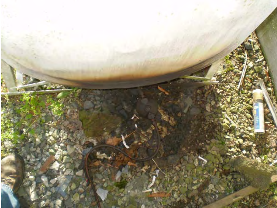
Photograph 7 – View of surface staining beneath AST supply line and filter adjacent to commercial building.
