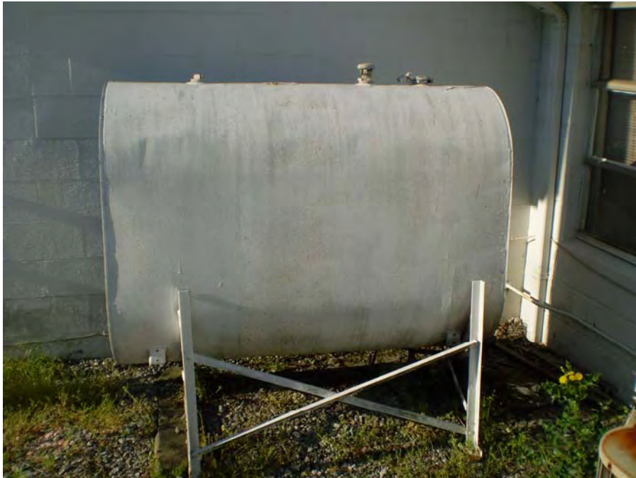
Photograph 6 – View of AST located on the east side of the commercial building at Parcel #16.
