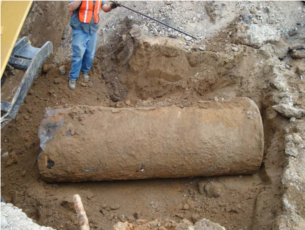
Photograph 3: View looking east at removal of UST #002. UST #001 product piping is shown in lower left.
