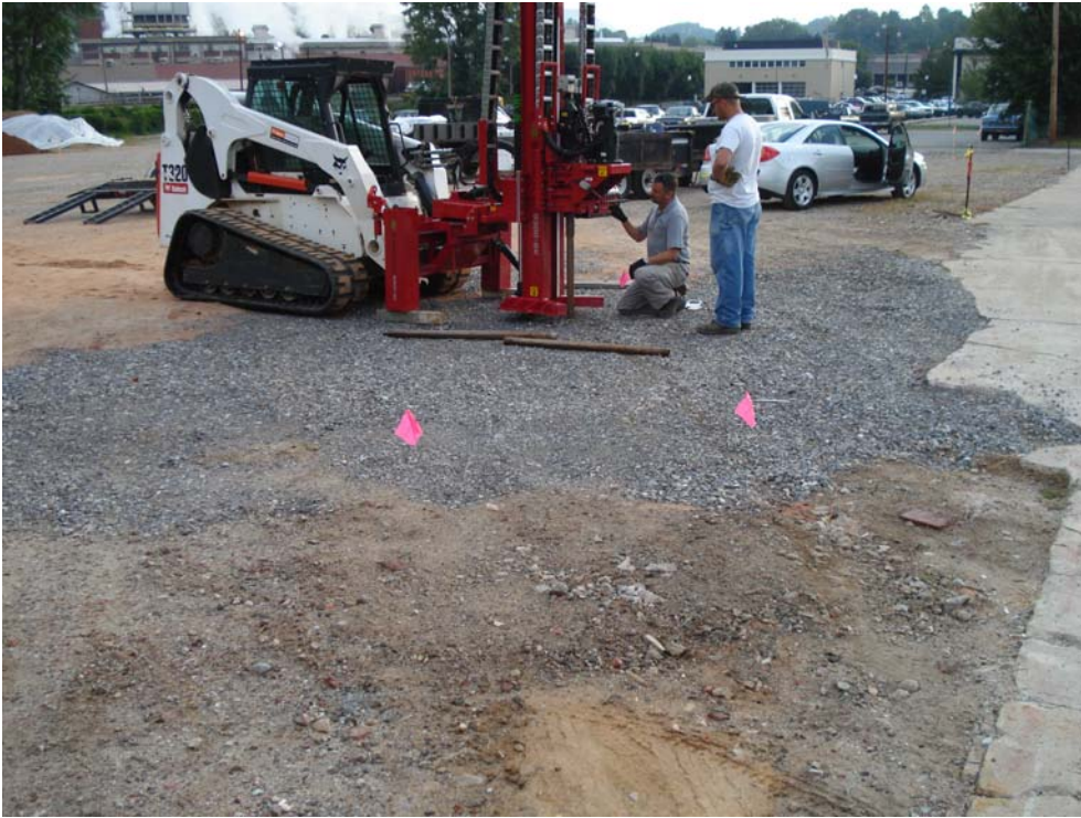
Photograph 5: View looking east at collection of confirmation soil sample SB7-4A. Confirmation soil sample locations SB7-7A and SB7-8 are marked by pink flags in foreground.
