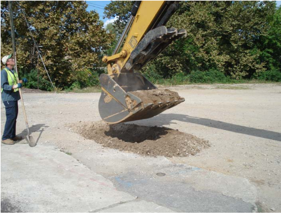
Photograph 1: View looking northwest at initial excavation of USTs at Parcel #7. Fill pipe cover for UST #003 is shown in center foreground.
