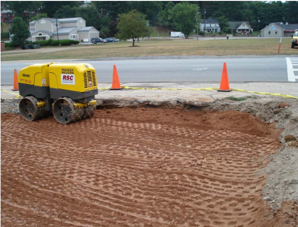
Photograph 4: View looking south at compaction of backfill material in UST pit using remote-controlled vibratory roller.
