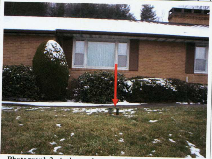
Photograph 2: A closer view, note fill port and vent pipe.
