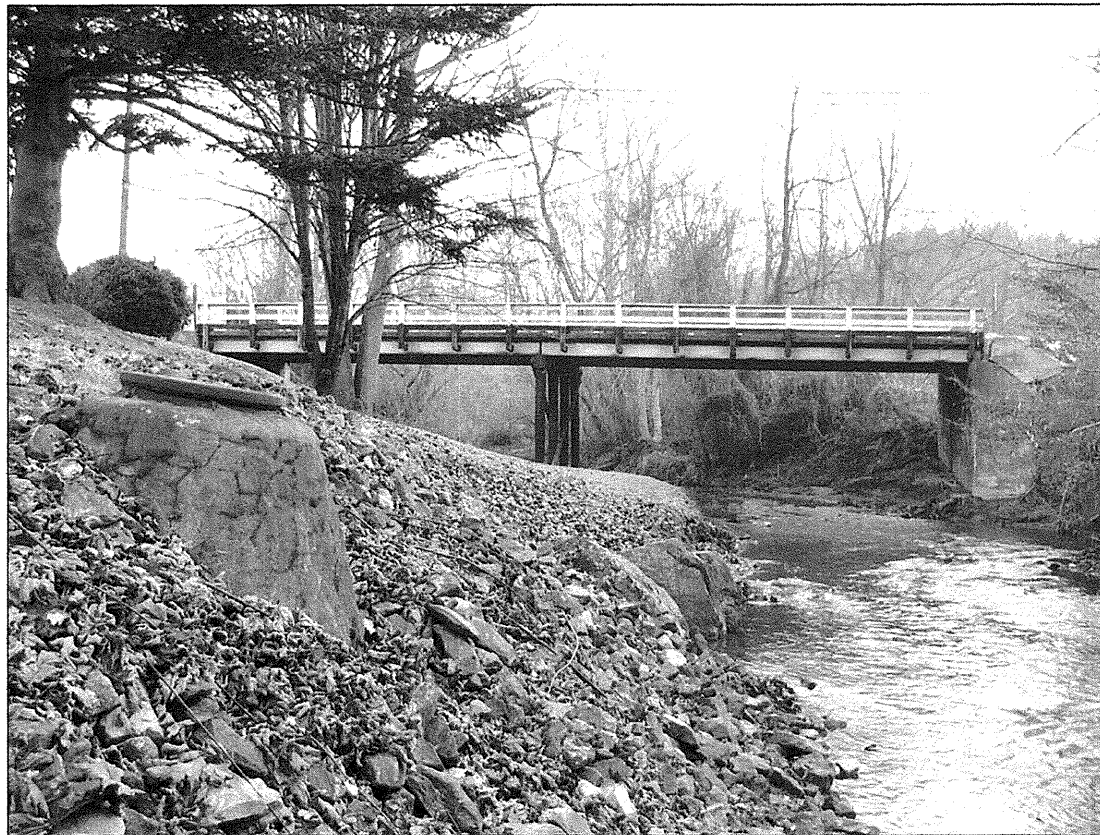
Photo 1: Looking upstream (East) at existing bridge. Line -L- is running from left to right. Note sewer manhole in foreground
