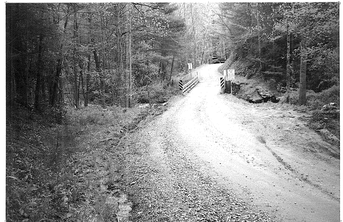
Figure 4. Looking back from Station 17+00. Note water in ditch.
