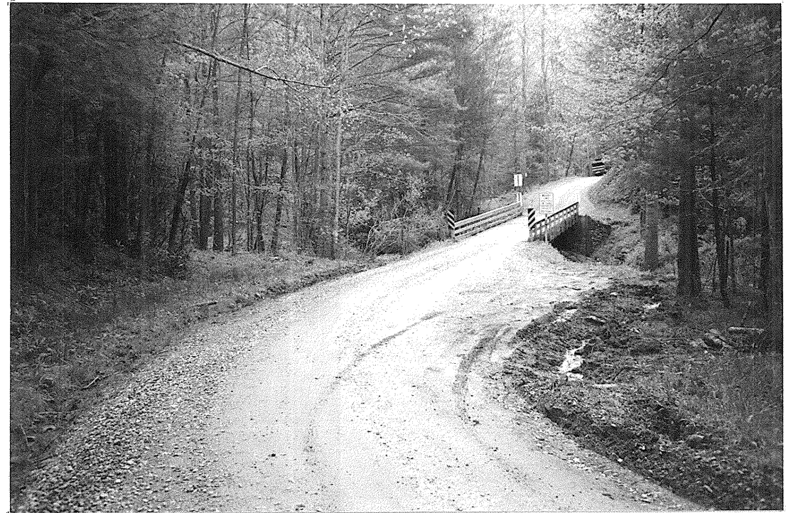
Figure 3. Looking back from Station 16+50. Note water in ruts on right.
