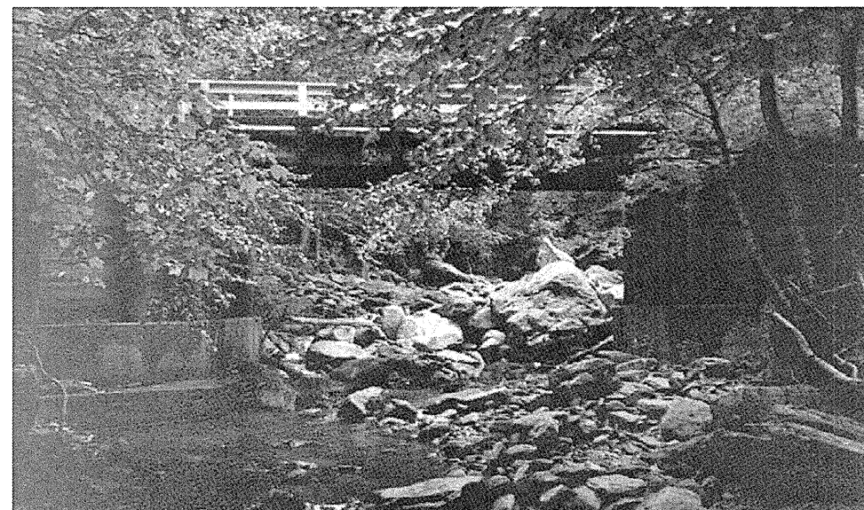
Photograph No. 2: This photograph was taken from the center of the new bridge location looking south at old bridge.
