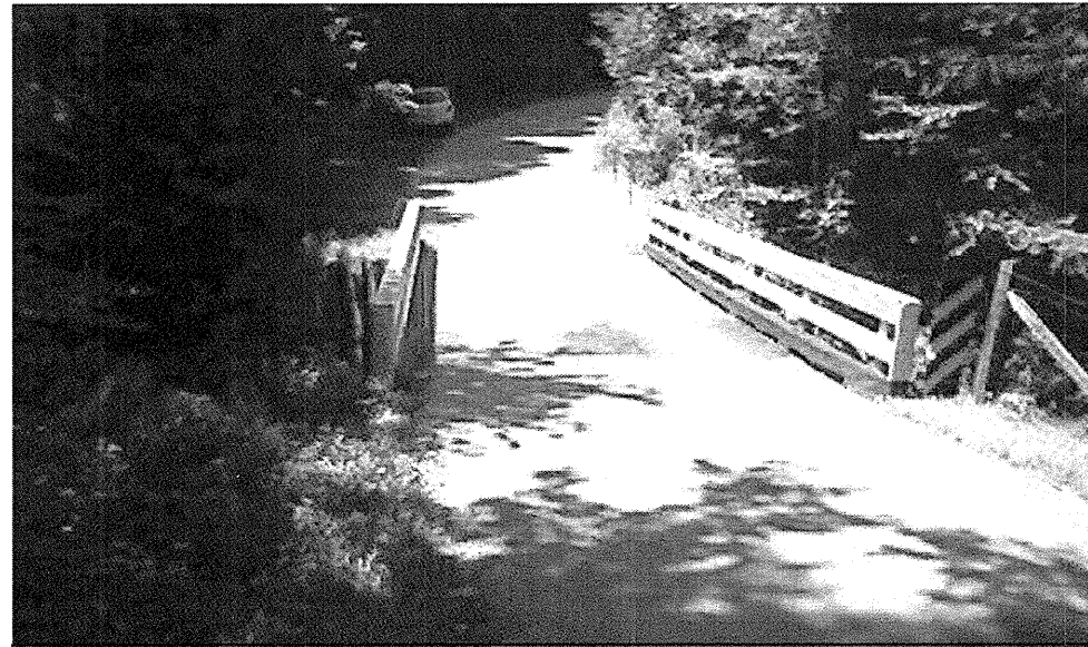
Photograph No. 1: This photograph was taken standing on the south end of the existing bridge looking north.
