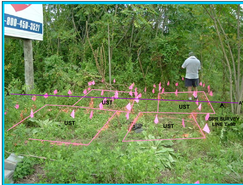
The photograph shows the location of four probable USTs buried 1.75 to 2.0 feet below surface, as suggested by the geophysical results at Parcel 21.
