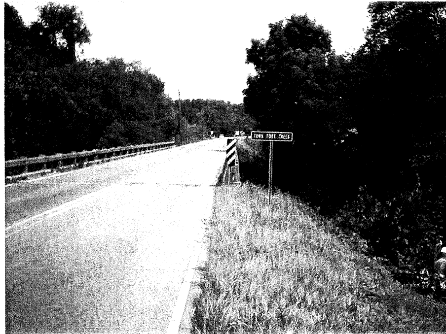
Photograph No. 1: This photograph was taken from the right side of the existing bridge, looking north.
