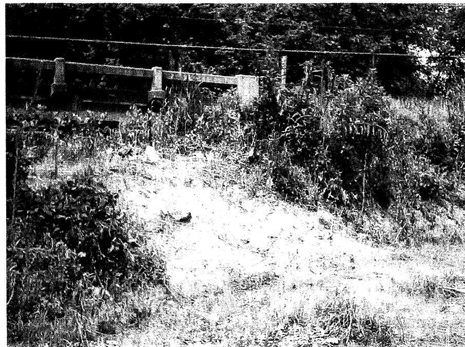
Photograph No. 6: This photograph was taken from the right side of the -L- alignment, looking west, across proposed End Bent No. 2.
