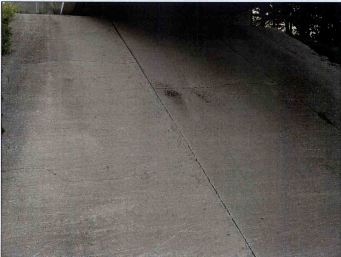
CRACKING IN SLOPE PROTECTION - SPAN 1
