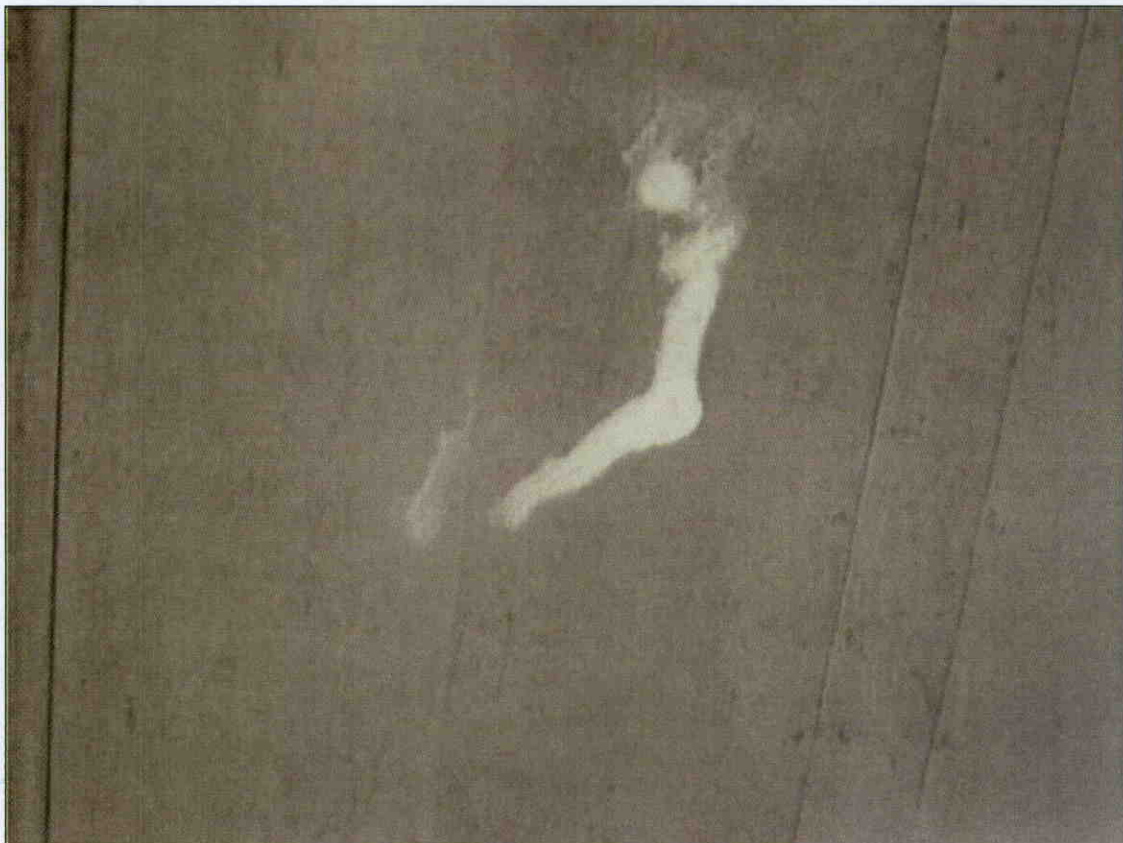
EFFLORESCENCE LEAKAGE IN SPAN 3 - 1/4 POINT
