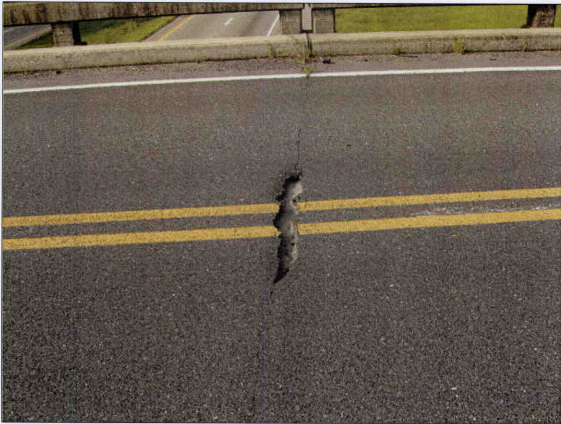
POTHOLE IN JOINT MEASURING 4 INCHES WIDE X 2 INCHES DEEP X 4 FOOT LONG AT INTERIOR BENT 3
