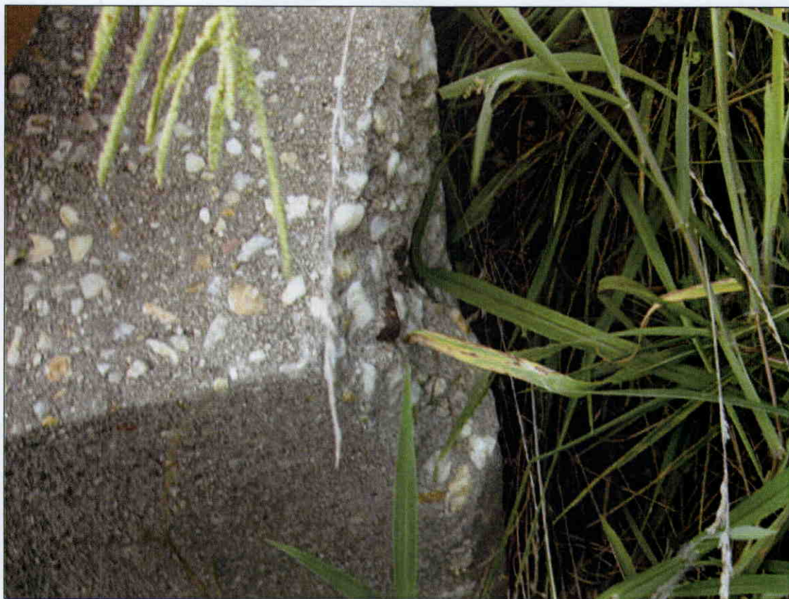
CHIP ON SOUTHEAST WINGWALL
