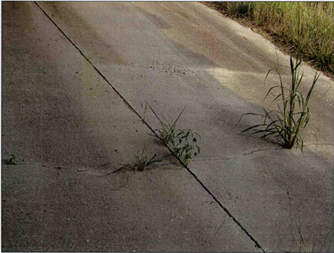
VEGETATION GROWING OUT OF CRACK IN SLOPE BANK
