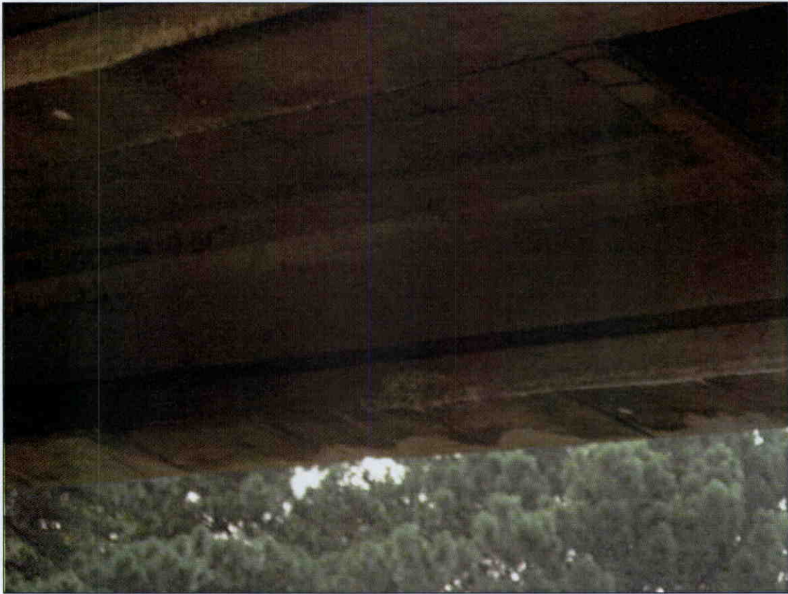
SPALL ON UNDERSIDE - BEAM 1, SPAN 3
