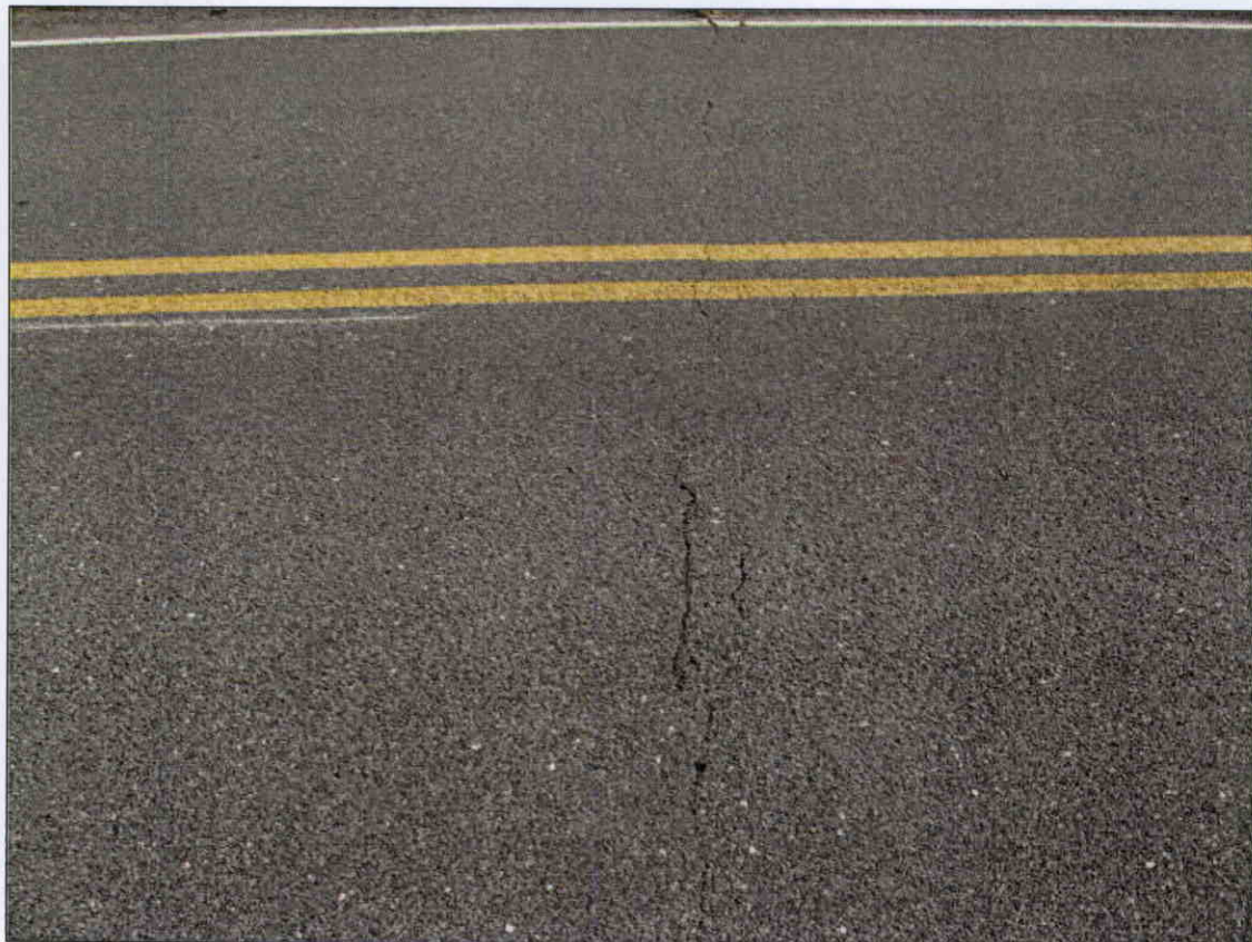
TYPICAL HAIRLINE CRACK OVER INTERIOR BENT 2 JOINT
