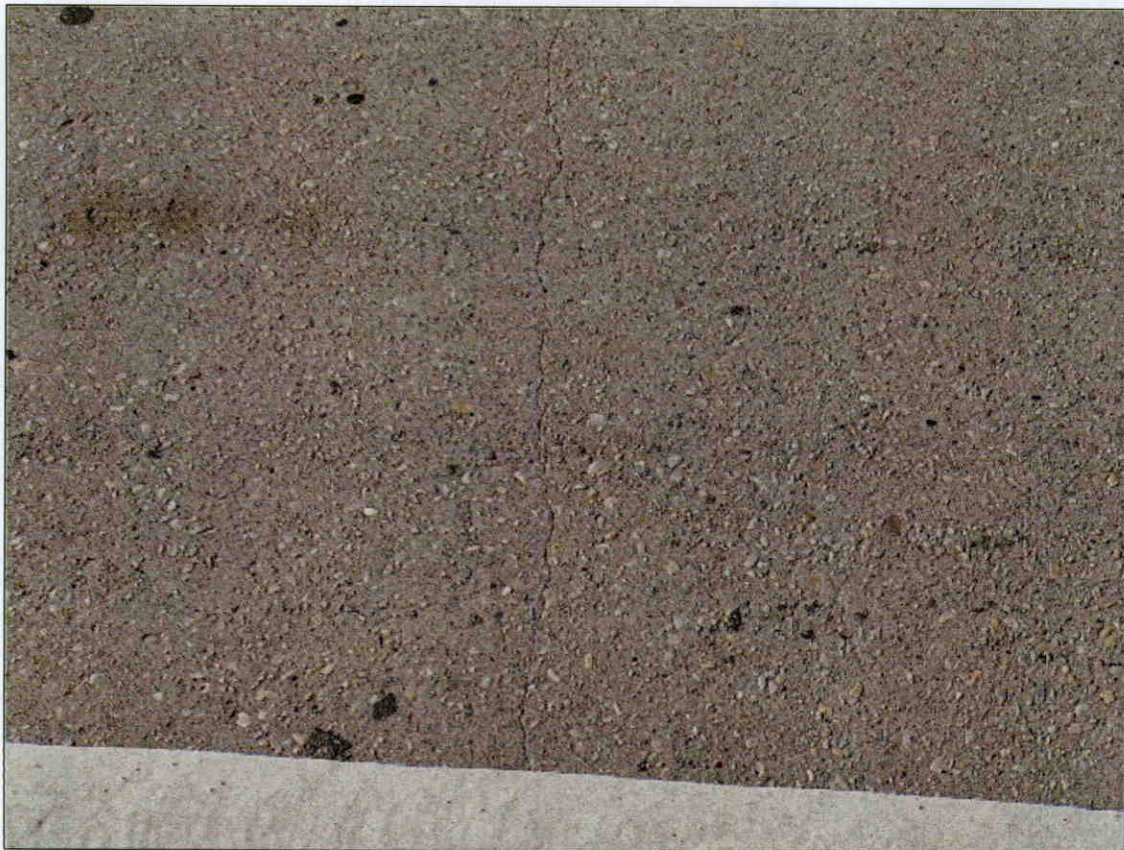
TRANSVERSE HAIRLINE CRACKS IN TOP OF DECK THROUGHOUT SPANS 1 AND 2, SPAN 2 SHOWN
