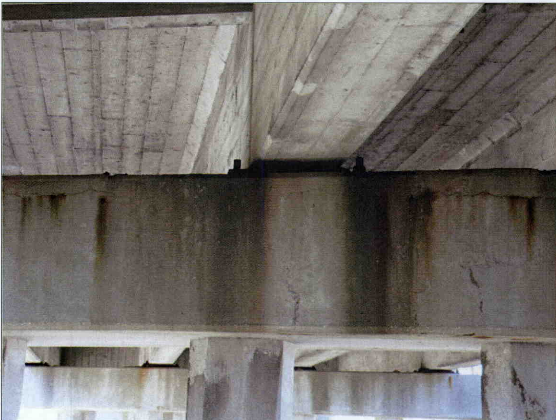
HAIRLINE TO 1/16 IN HORIZONTAL CRACK IN FACE OF BENT 3 CAP BETWEEN PILES 4 AND 6, SPAN 4 SIDE
