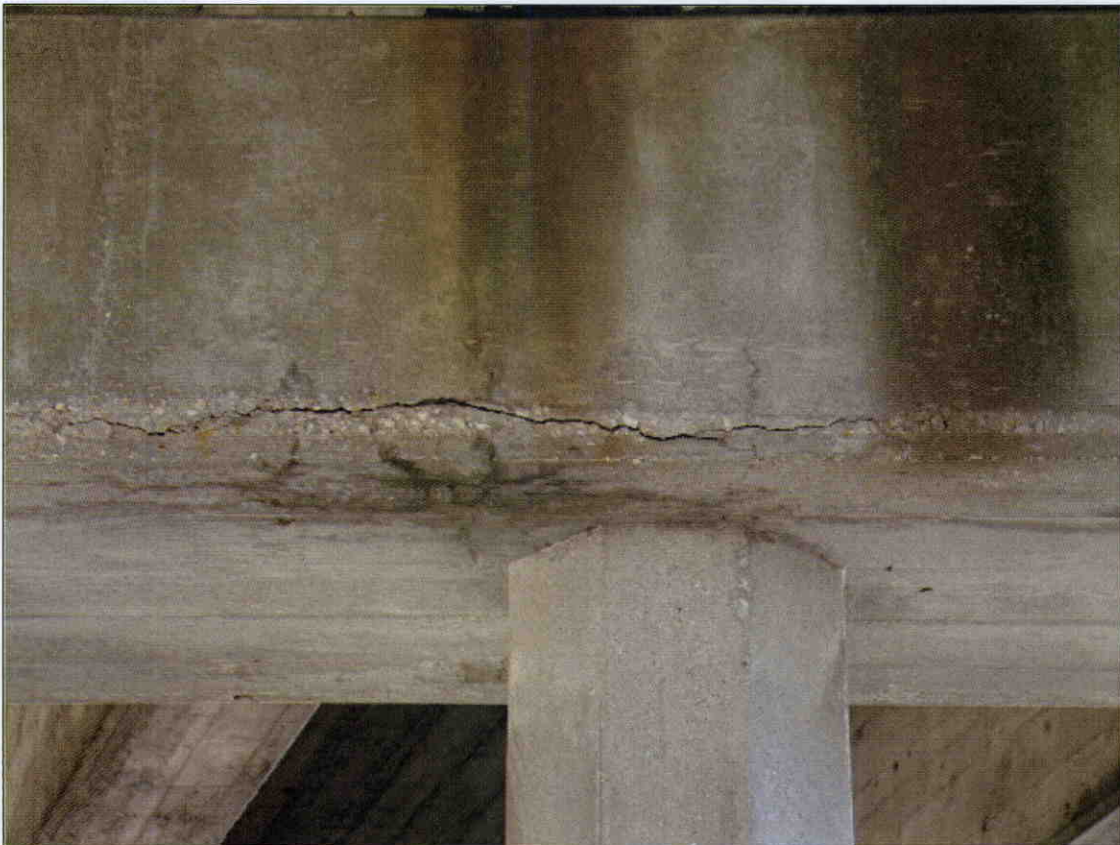
HAIRLINE TO 1/4 IN HORIZONTAL CRACK IN FACE OF BENT 2 CAP BETWEEN PILES 3 AND 4, SPAN 3 SIDE
