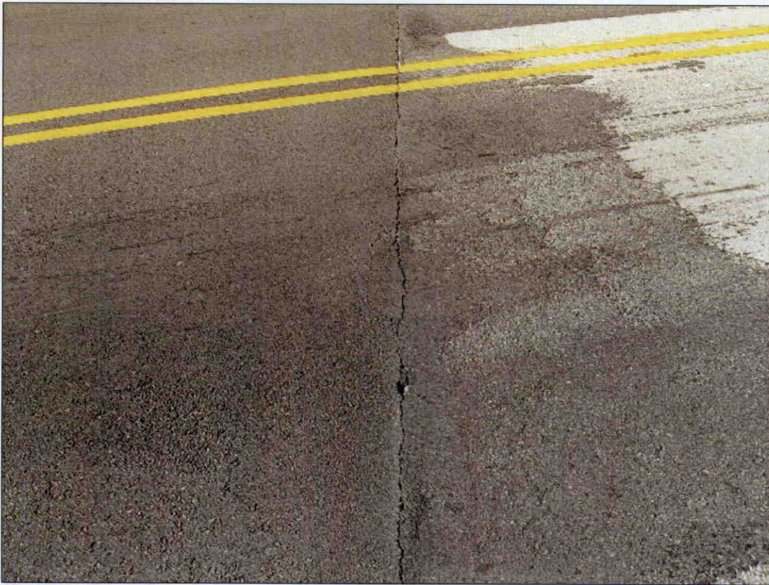
TRANSVERSE CRACK IN ASPHALT WEARING SURFACE ALONG END BENT 2 FILL FACE WITH 1/4 IN OF SETTLEMENT
