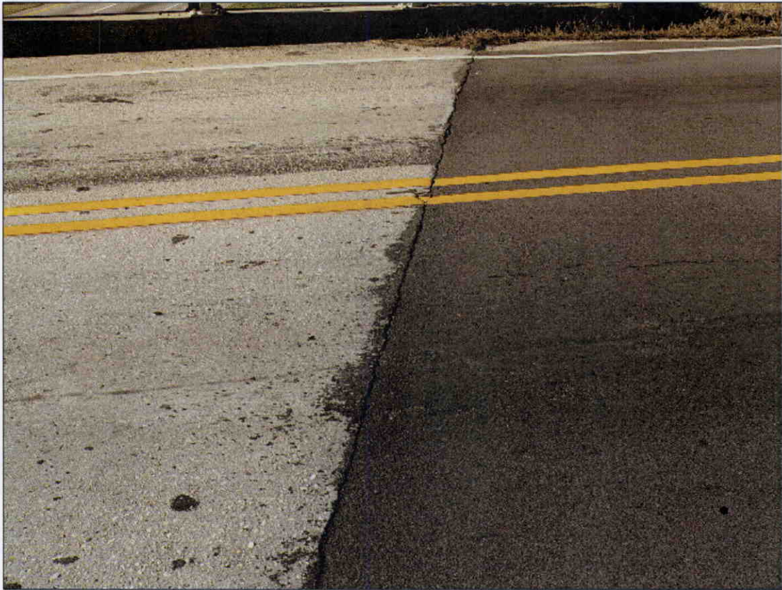
TRANSVERSE CRACK IN ASPHALT WEARING SURFACE ALONG END BENT 1 FILL FACE WITH 1/4 IN OF SETTLEMENT
