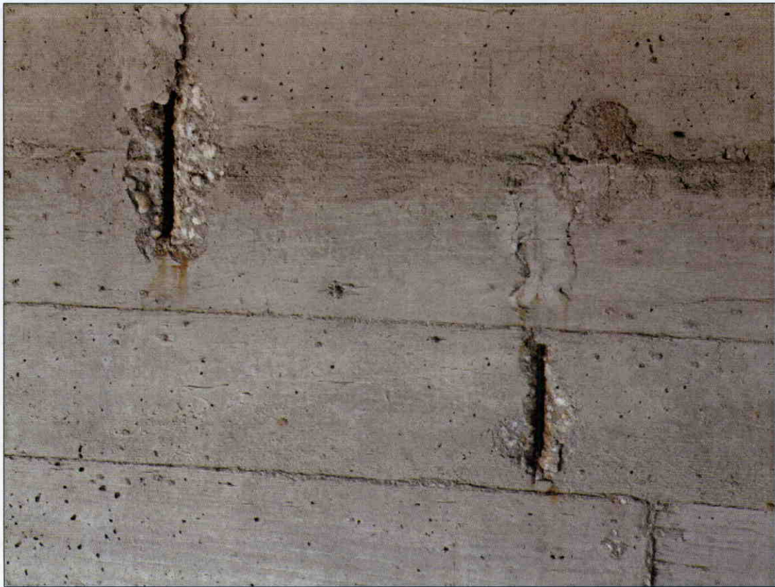
4 IN X 12 IN X 1/2 IN DEEP AND 2 IN X 5 IN X 1/2 IN DEEP SPALLS WITH EXPOSED REBAR IN FACE OF GIRDER 1, SPAN 4 NEAR END BENT 2
