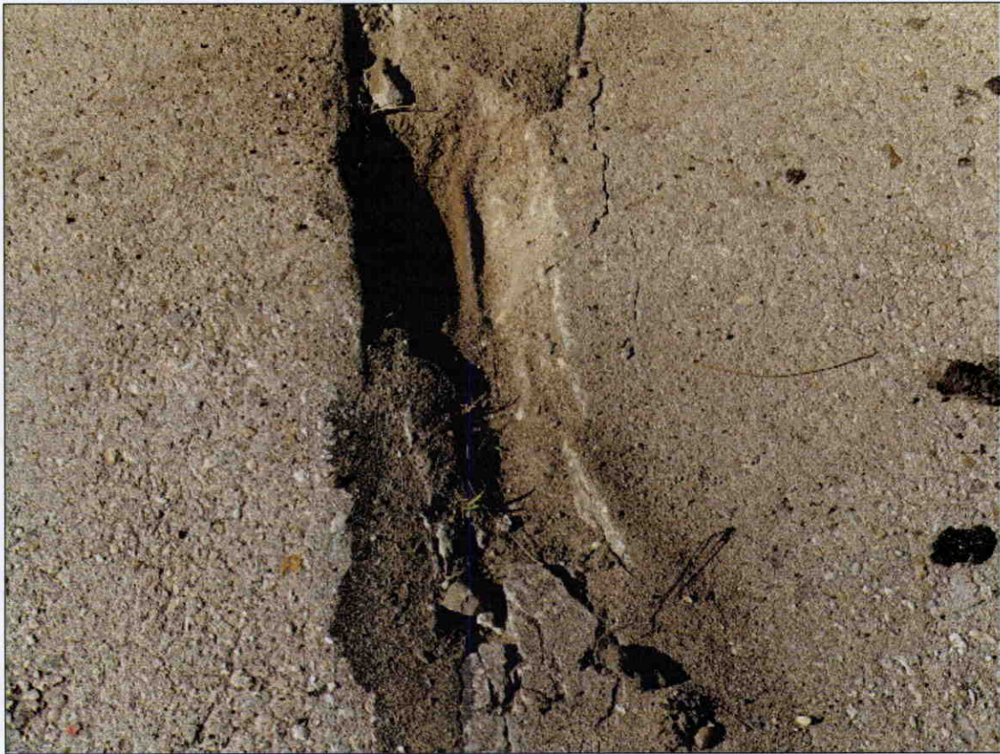
6 IN X 24 IN X 3 IN DEEP SPALL WITH EXPOSED REBAR IN TOP OF DECK AT DECK EXPANSION JOINT AT BENT 2
