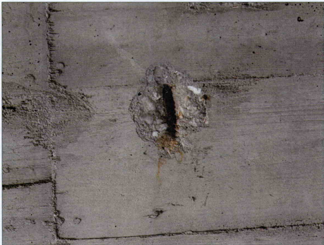
4 IN X 4 IN X 1/2 IN DEEP SPALL WITH EXPOSED REBAR IN FACE OF GIRDER 1, SPAN 4 NEAR END BENT 2
