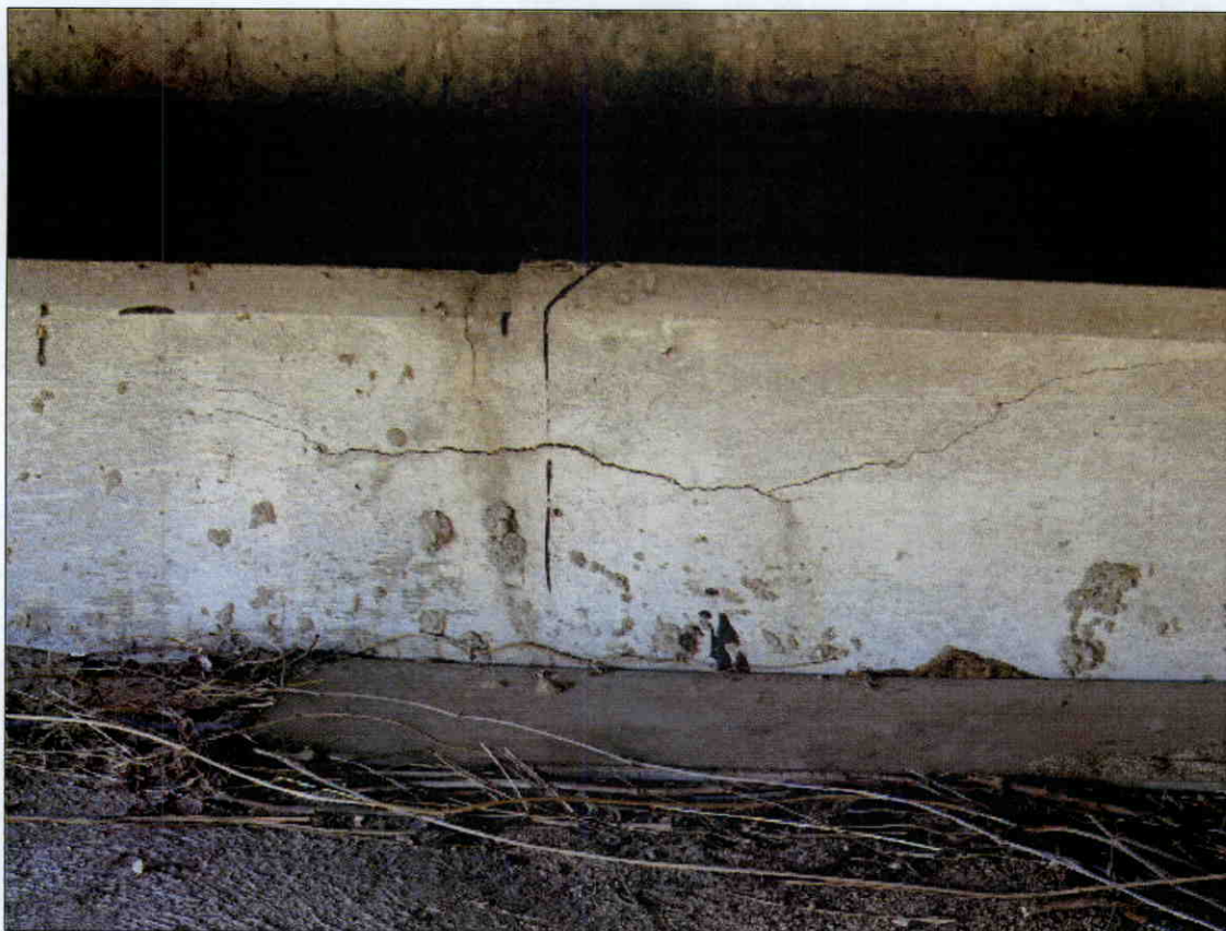
HAIRLINE TO 1/16 IN HORIZONTAL CRACK IN FACE OF END BENT 2 CAP BAY 1
