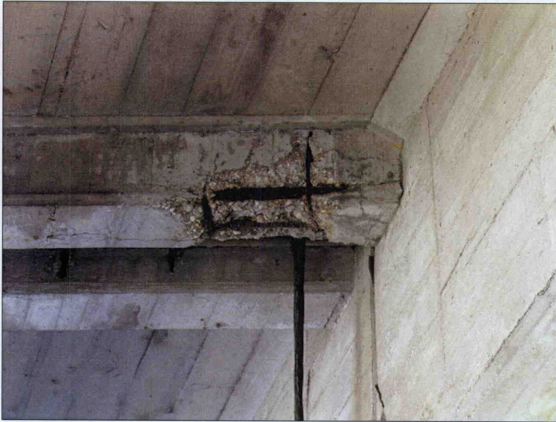
9 IN X 20 IN X 2 IN DEEP SPALL WITH EXPOSED REBAR IN BOTTOM OF END DIAPHRAGM AT BENT 1, BAY 1, SPAN 1
