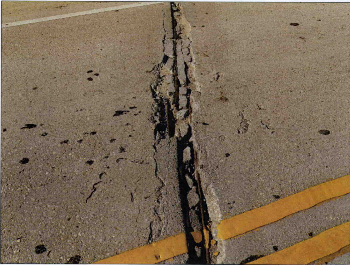
9 IN X 12 FT X 3 IN DEEP SPALL WITH EXPOSED REBAR IN TOP OF DECK WITH ADDITIONAL AREAS OF BROKEN CONCRETE AT DECK EXPANSION JOINT AT BENT 2
