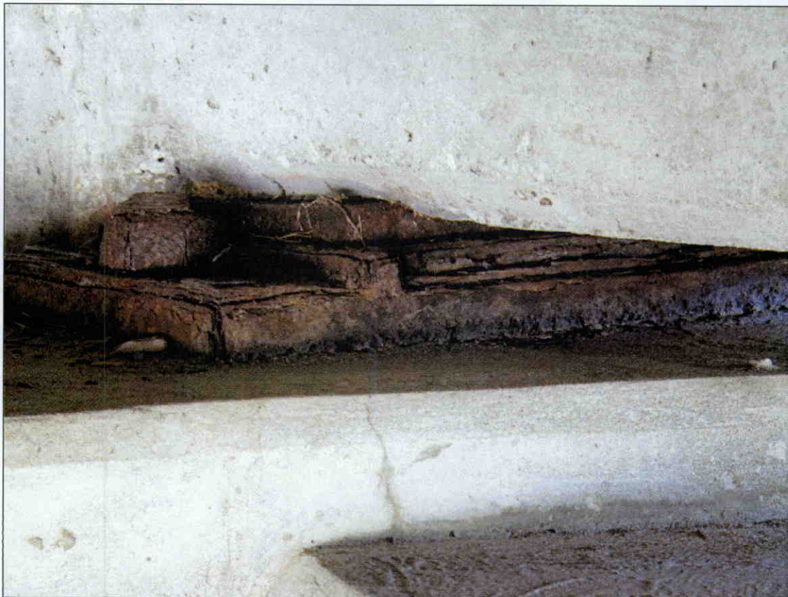
RUST AND DELAMINATION OF BEARING AT GIRDER 4, END BENT 2, SIMILAR CONDITION AT GIRDER 1
