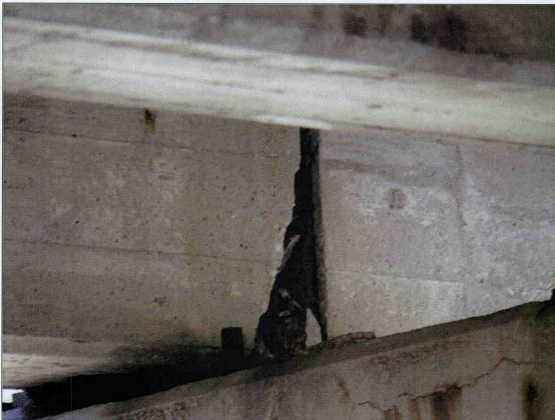
19 IN X 5 IN X 3 IN DEEP SPALL IN FACE OF GIRDER 4, SPAN 4 AT BENT 3, SIMILAR SPALL AT GIRDER 1, SPAN 2 AT BENT 2 AND GIRDER 1, SPAN 3 AT BENT 3
