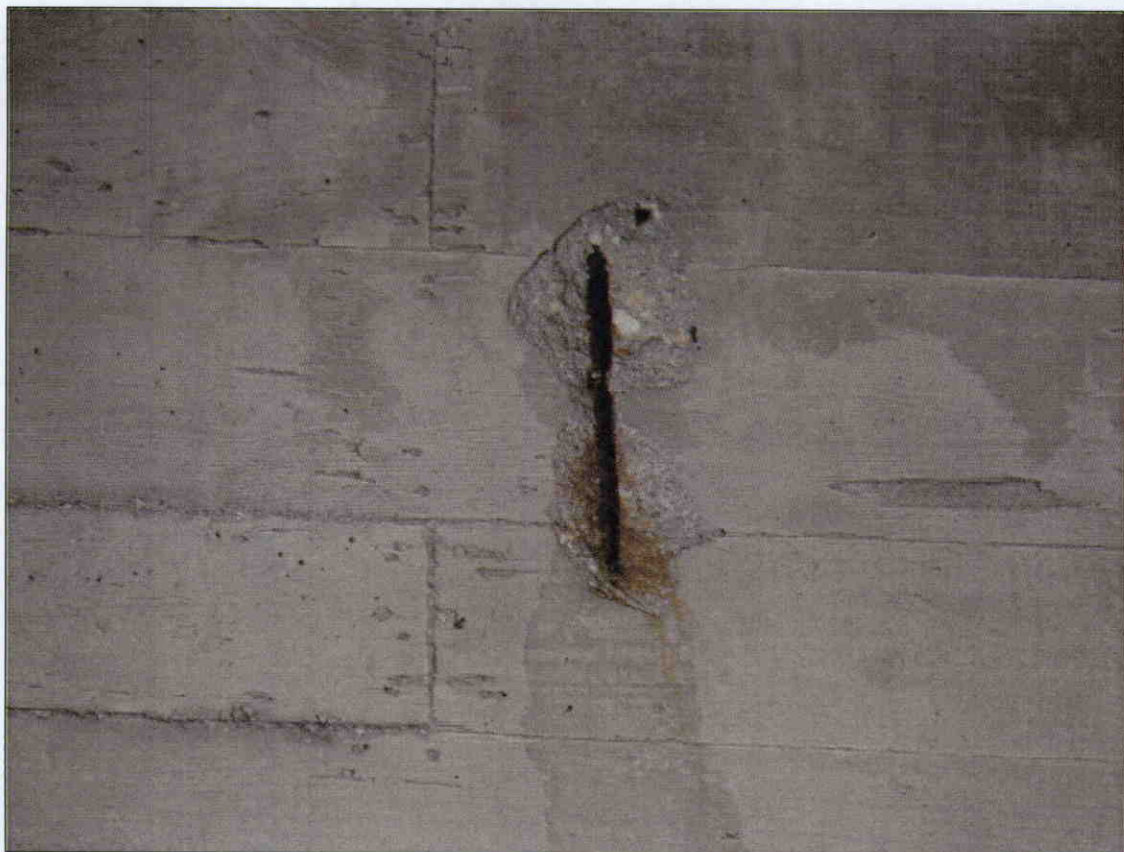
4 IN X 9 IN X 1/2 IN DEEP SPALL WITH EXPOSED REBAR IN RIGHT FACE OF GIRDER 1, SPAN 2 NEAR BENT 2
