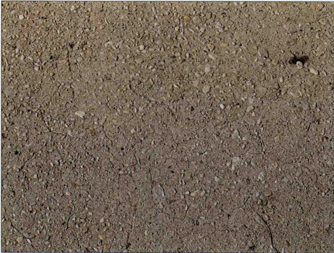
ROUGH AND WORN SURFACE WITH EXPOSED AGGREGATE AND HAIRLINE MAP CRACKING IN TOP OF DECK, SPAN 1 SHOWN, SIMILAR CONDITION THROUGHOUT
