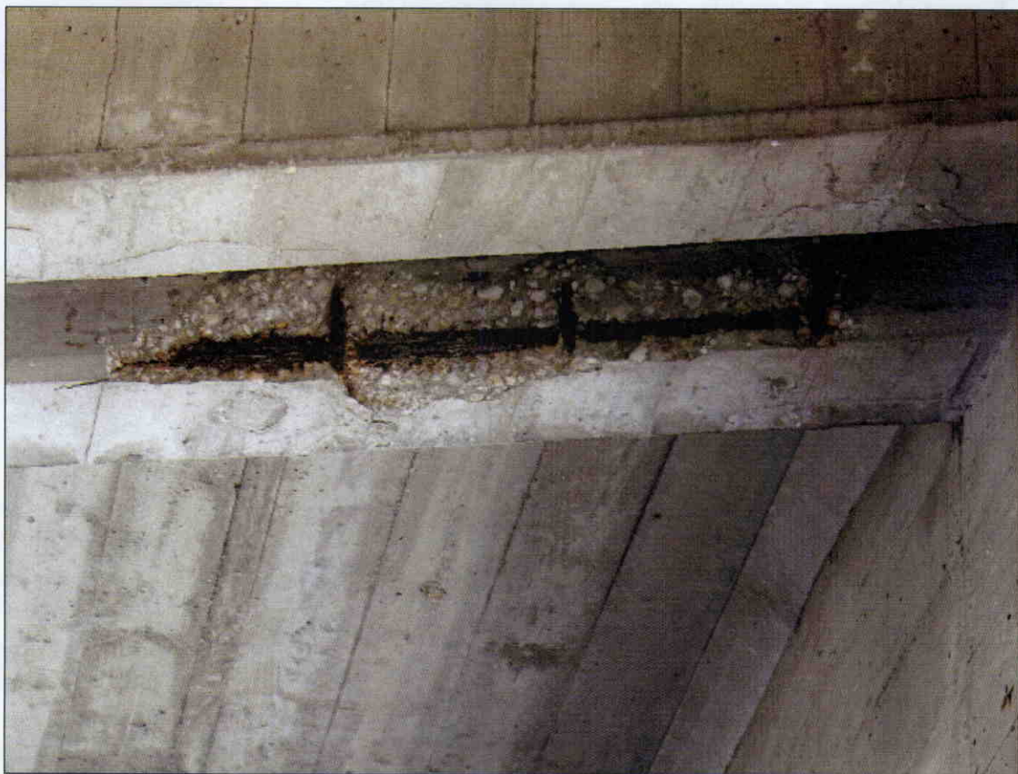
10 IN X 40 IN X 2 IN DEEP SPALL WITH EXPOSED REBAR IN BOTTOM OF END DIAPHRAGM AT BENT 1, BAY 2, SPAN 2
