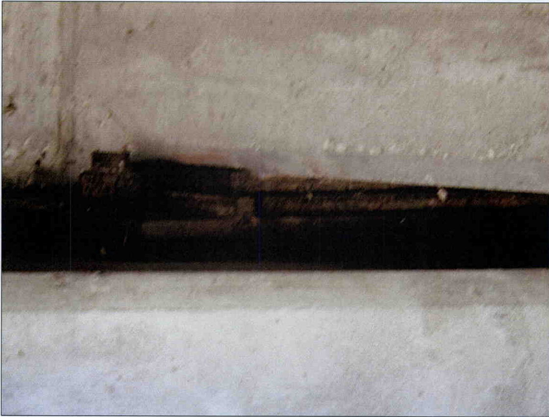
RUSTED BEARING AT GIRDER 2, END BENT 2, SIMILAR CONDITION AT GIRDER 3
