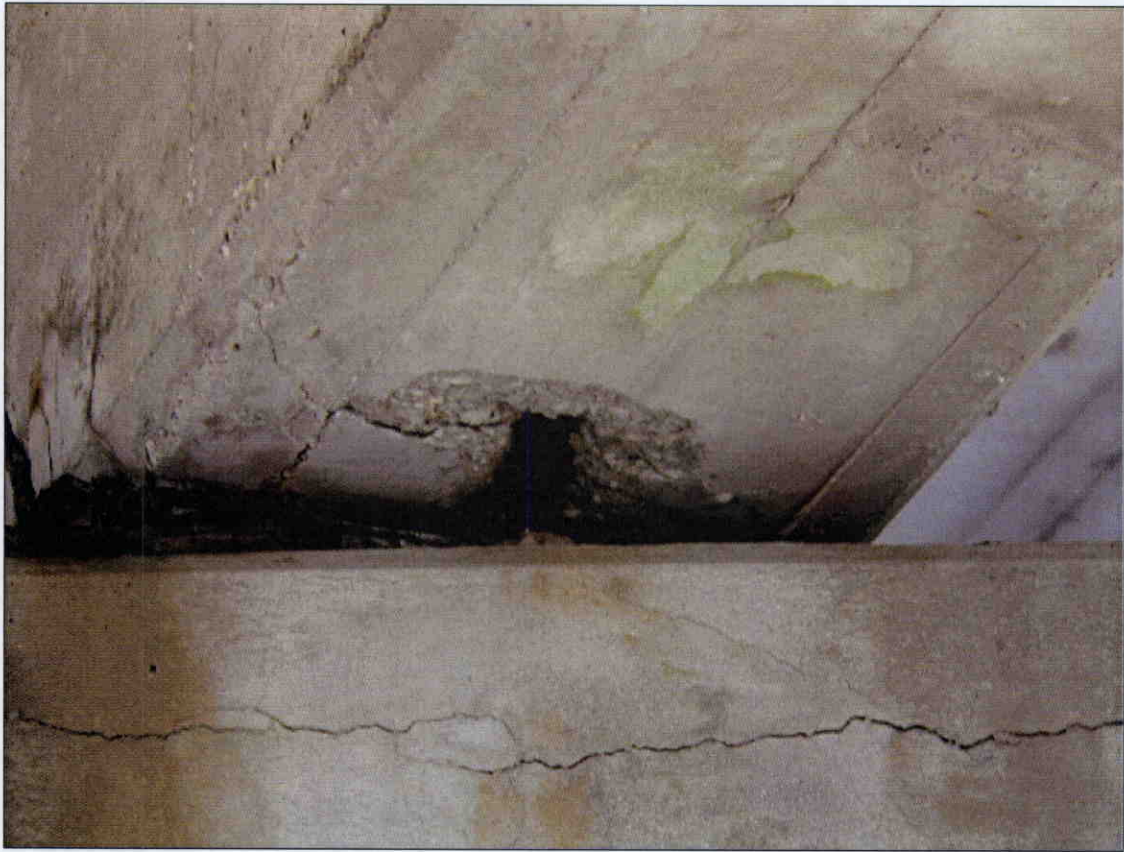
9 IN X 9 IN X 1 IN DEEP SPALL WITH EXPOSED REBAR IN BOTTOM OF GIRDER 2, SPAN 1 AT BENT 1, SIMILAR SPALLS GIRDERS 3 AND 4
