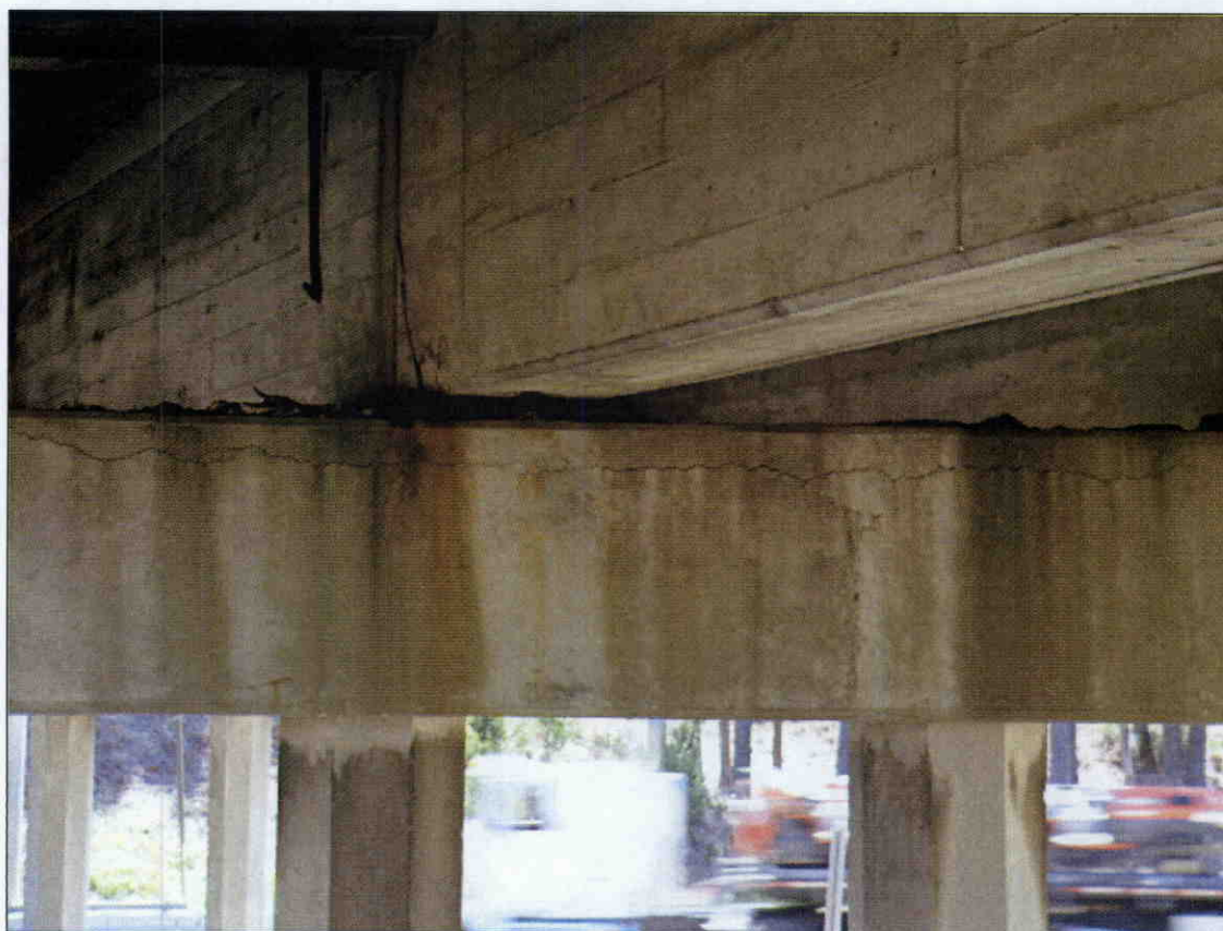
HAIRLINE TO 1/8 IN HORIZONTAL CRACK IN FACE OF BENT 1 CAP BETWEEN PILES 2 AND 6, SPAN 1 SIDE
