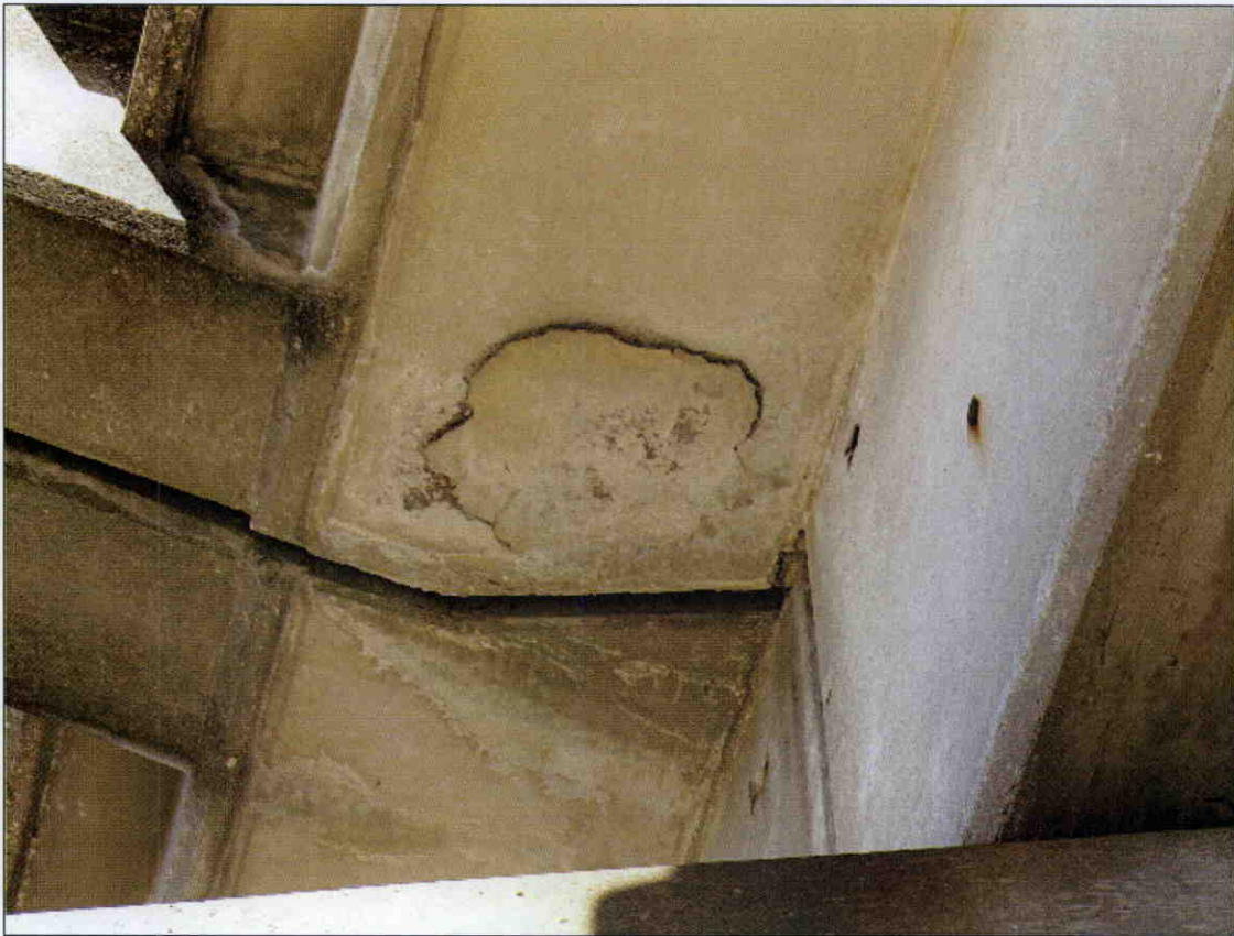
18 IN X 18 IN IMMINENT SPALL IN BOTTOM OF OUT SOUTH DECK OVERHANG AT BENT 2
