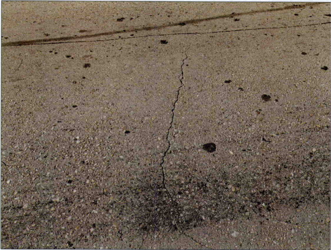
HAIRLINE TO 1/8 IN TRANSVERSE CRACKS IN TOP OF DECK THROUGHOUT SPAN 4
