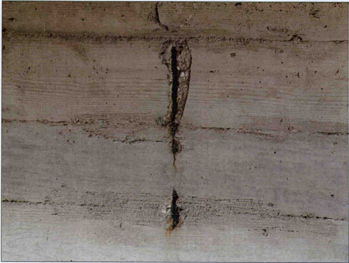
2 IN X 9 IN X 1/2 IN DEEP AND 2 IN X 3 IN X 1/2 IN DEEP SPALLS WITH EXPOSED REBAR IN FACE OF GIRDER 3, SPAN 4 NEAR END BENT 2
