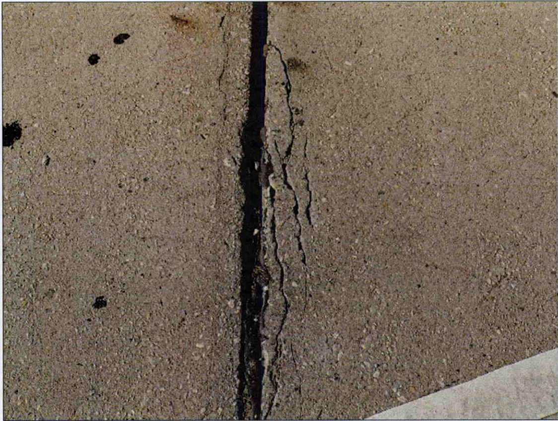
1/8 IN TRANSVERSE CRACKS WITH IMMINENT SPALL IN TOP OF DECK AT DECK EXPANSION JOINT AT BENT
