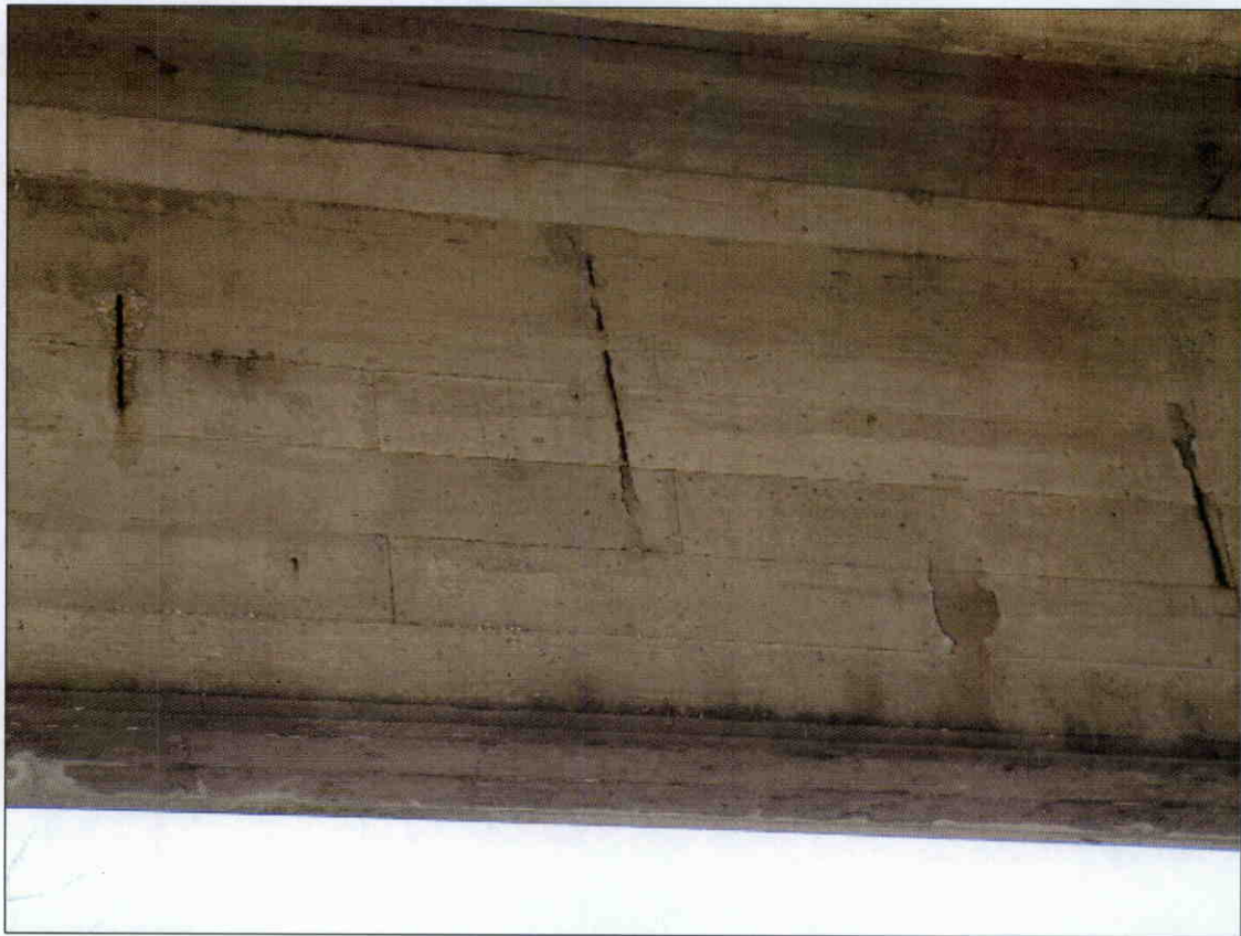
2 IN X 15 IN X 1/2 IN DEEP SPALL WITH EXPOSED REBAR IN RIGHT FACE OF GIRDER 1, SPAN 2 NEAR BENT 1, 3 TOTAL
