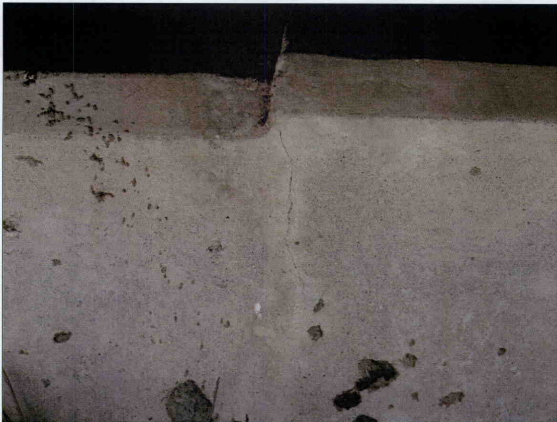
VERTICAL HAIRLINE CRACK IN FACE OF END BENT 2 CAP AT STEP, SIMILAR CONDITION AT END BENT 1
