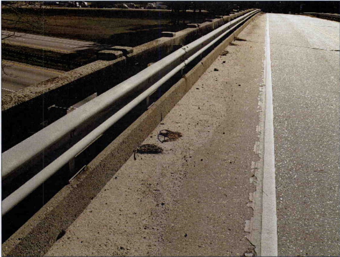
DIRT AND DEBRIS WITH VEGETATION GROWING ALONG NORTH CURB, SIMILAR CONDITION AT SOUTH CURB
