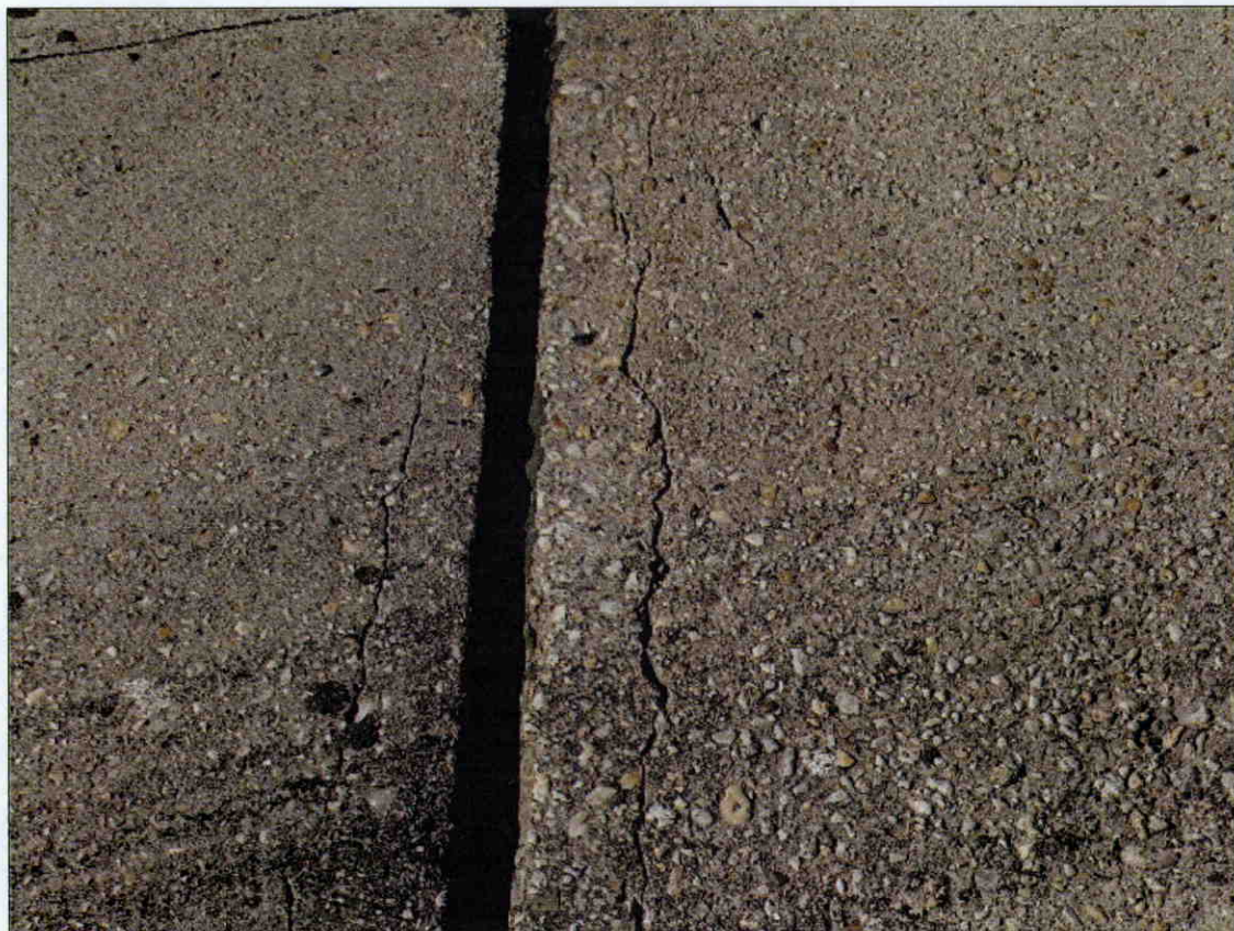
HAIRLINE TO 1/8 IN TRANSVERSE CRACKS IN TOP OF DECK AT DECK EXPANSION JOINT AT BENT 3
