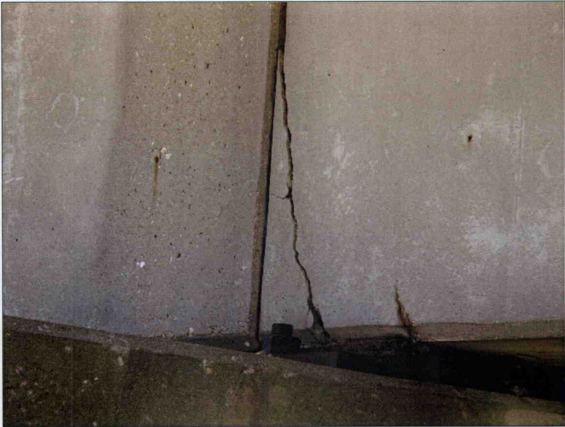
24 IN LONG X 1/4 IN VERTICAL CRACK IN END OF GIRDER 1 AT BENT 1, SPAN 1 SIDE, SIMILAR CRACKS AT ENDS OF GIRDERS AT OTHER BENTS
