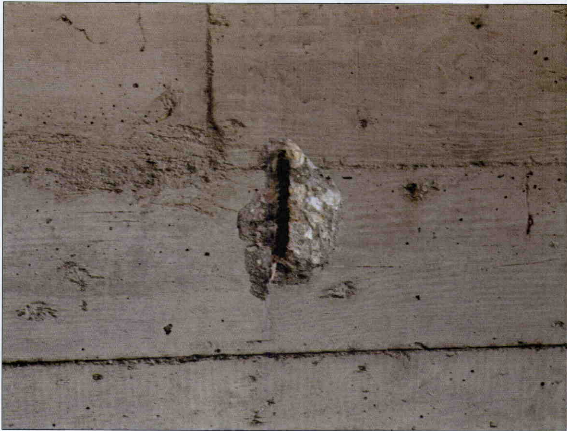
4 IN X 6 IN X 1/2 IN DEEP SPALL WITH EXPOSED REBAR IN FACE OF GIRDER 1, SPAN 4 NEAR END BENT 2
