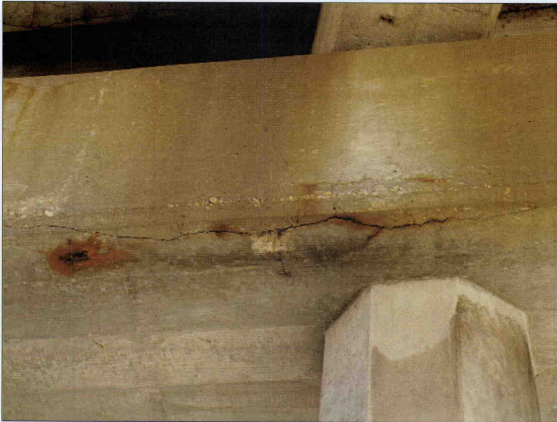
HAIRLINE TO 1/8 IN LONGITUDINAL CRACK IN BOTTOM OF BENT 2 CAP AT PILE 7, SIMILAR CRACKS IN BOTTOM OF ALL BENT CAPS
