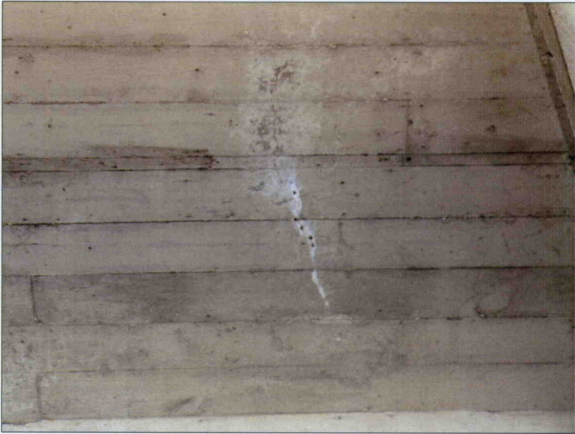
TRANSVERSE HAIRLINE CRACK WITH EFFLORESCENCE IN BOTTOM OF DECK THROUGHOUT SPAN 4
