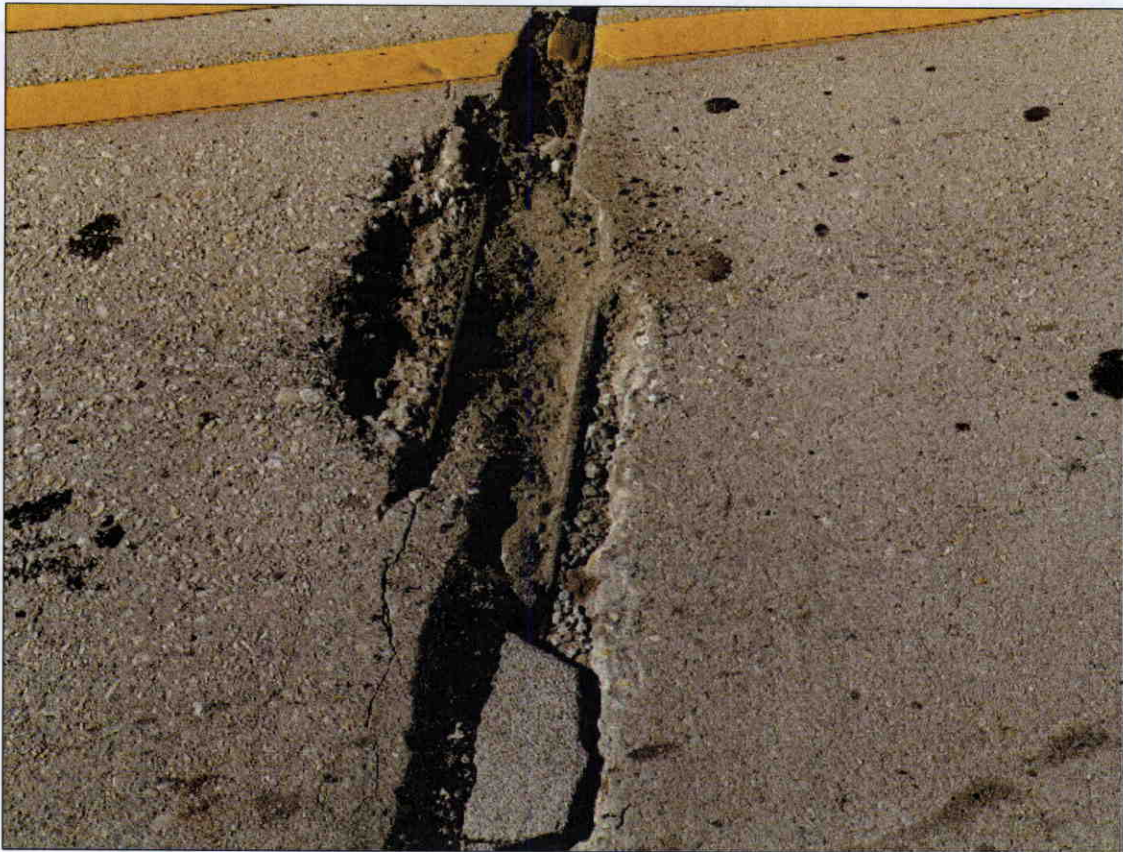
14 IN X 36 IN X 3 IN DEEP SPALL WITH EXPOSED REBAR IN TOP OF DECK AT DECK EXPANSION JOINT AT BENT 1
