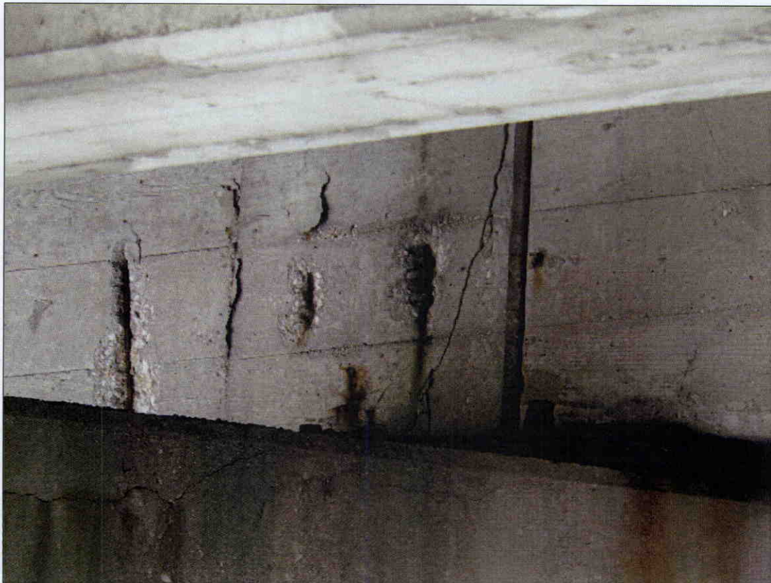
3 IN X 12 IN X 1/2 IN DEEP SPALL WITH EXPOSED REBAR IN FACE OF GIRDER 1, SPAN 3 AT BENT 3, 3 TOTAL
