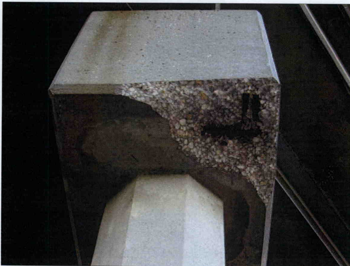
BOTTOM SOUTH END OF BENT 1 CAP SPALLED 18 IN. X 20 IN. WITH EXPOSED REBAR
