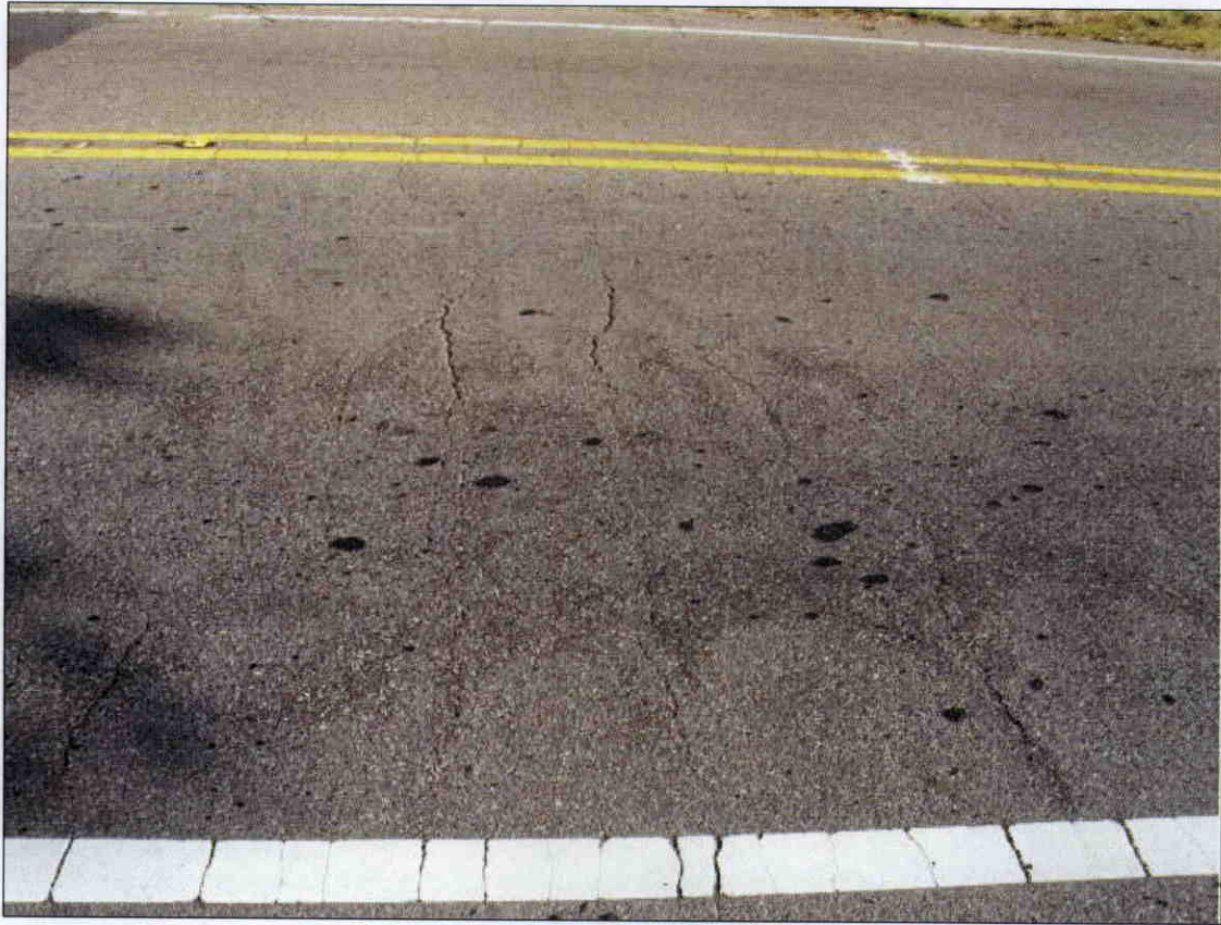
TRANSVERSE CRACK IN ASPHALT WEARING SURFACE AT SOUTH APPROACH
