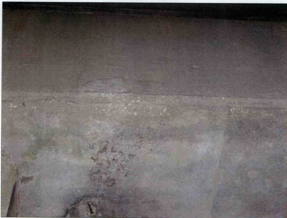
1/16 IN. HORIZONTAL CRACK ON BOTTOM SOUTH CORNER OF BENT 4 CAP BETWEEN PILES 6 AND 7
