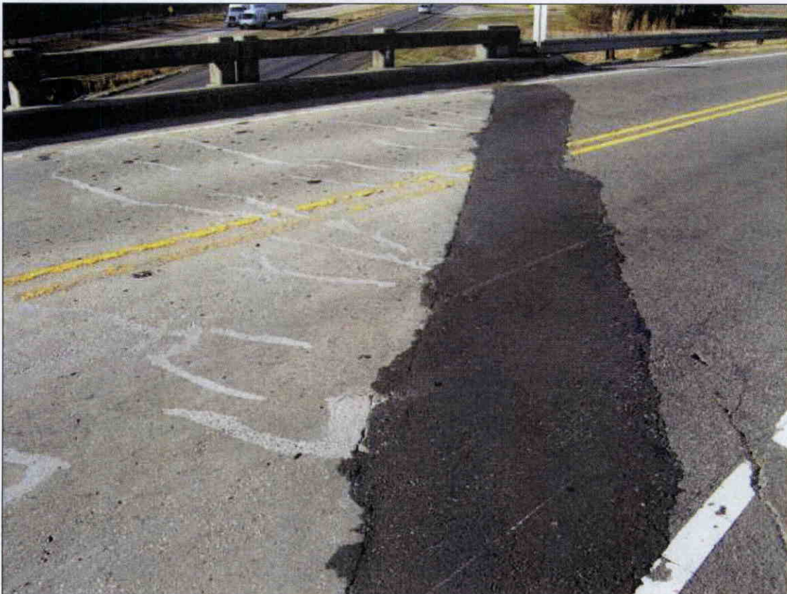
PATCHED ASPHALT WEARING SURFACE AT NORTH APPROACH
