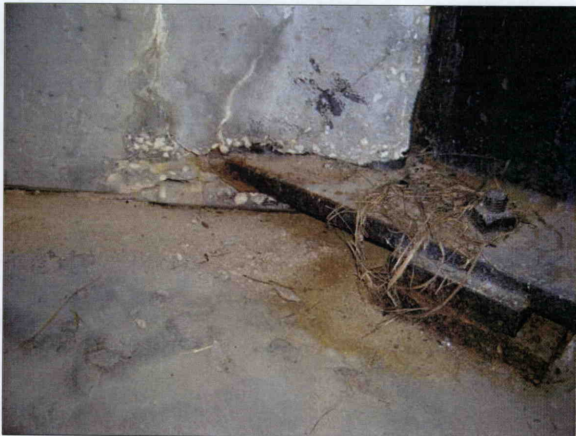
CURTAIN WALL SPALLING AT END OF BEAM 3 END BENT 1
