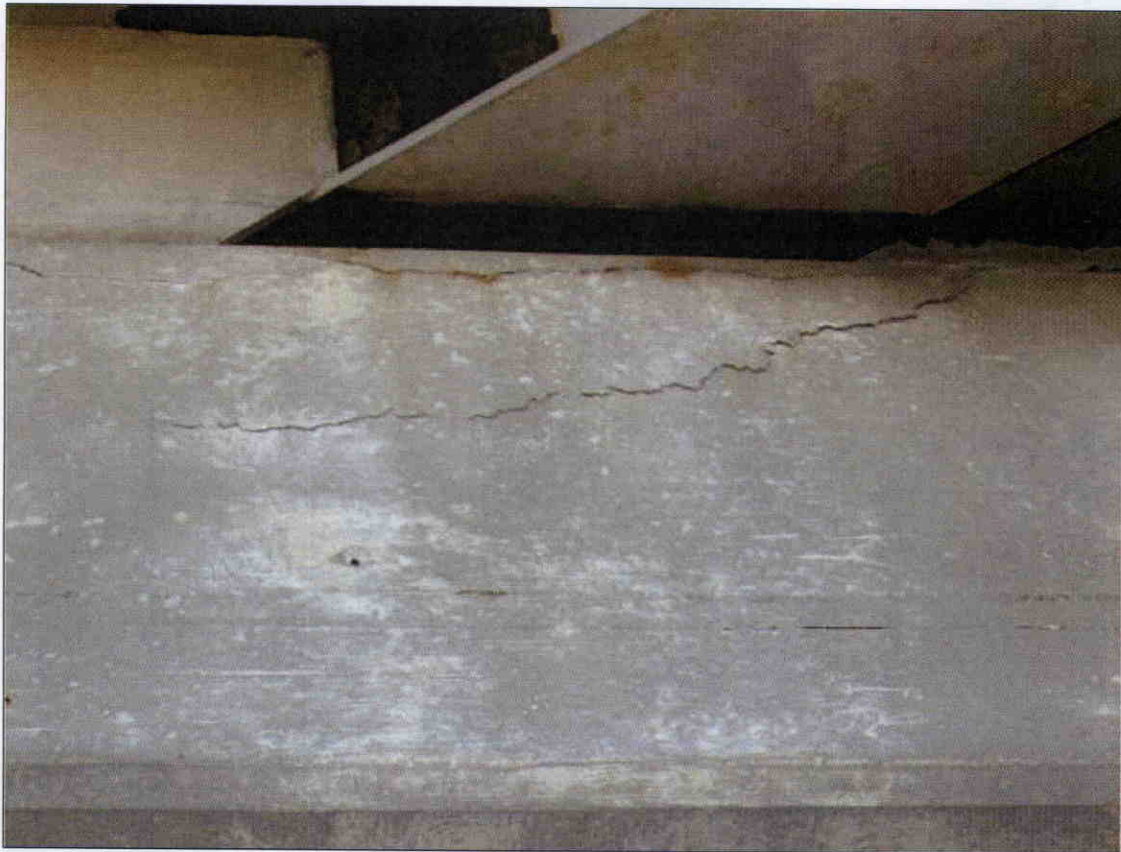
NORTH FACE OF BENT 1 CAP DELAMINATED 3 FT. X 1 FT. UNDER BEAM 4 SPAN 2 . DELAMINATION EXTEND ON TOP OF CAP FOR 8 IN. AND TO BEARING PLATE 3.5 IN.FROM
