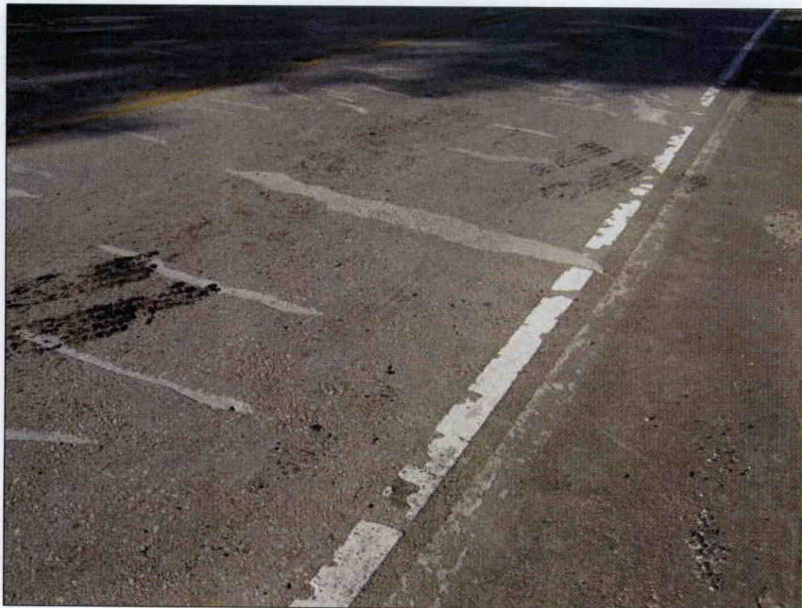
RANDOM CONCRETE PATCHED AREAS ON DECK AT SPAN 1
