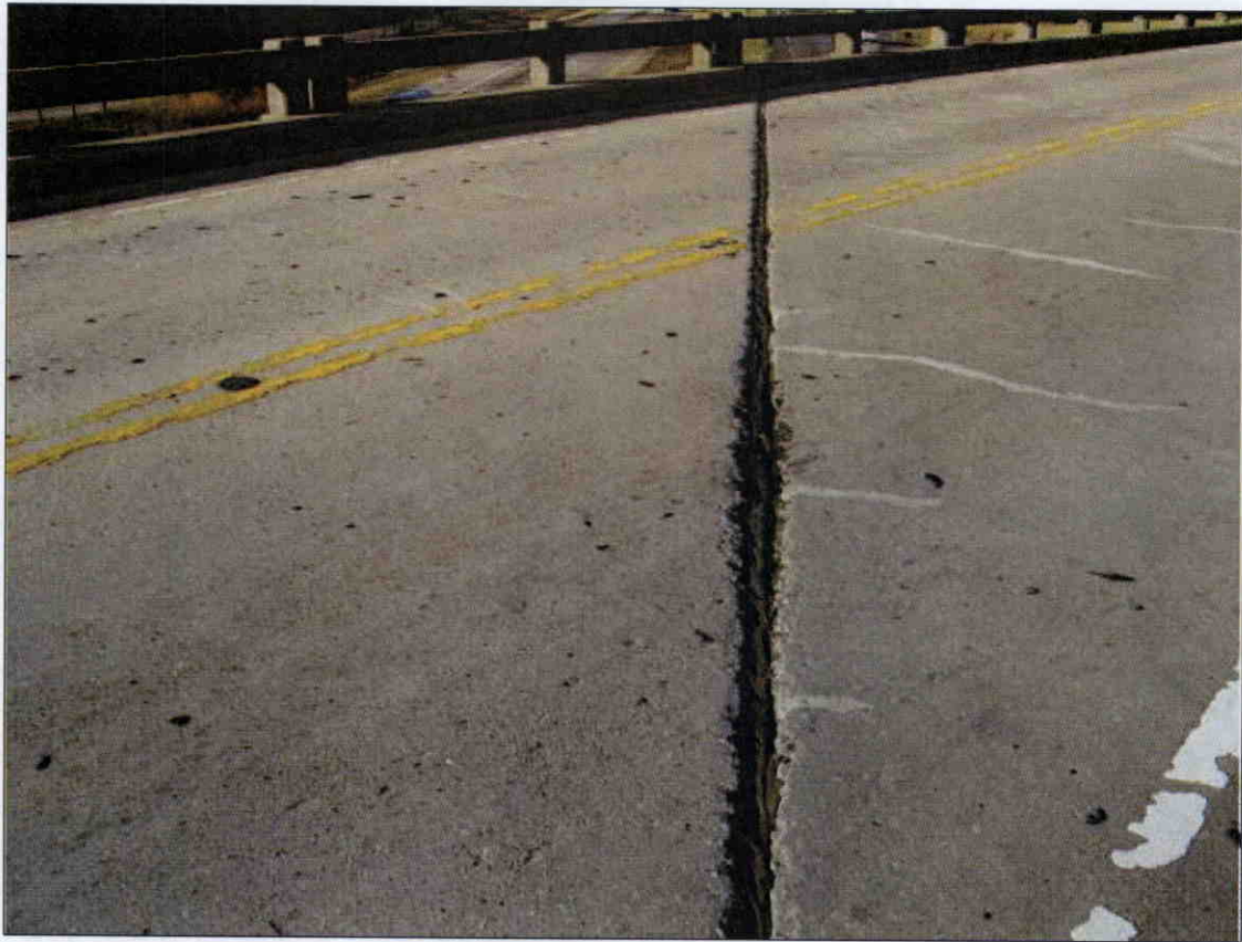
END OF SPANS SPALLING AT BENT 3 EXPANSION JOINT
