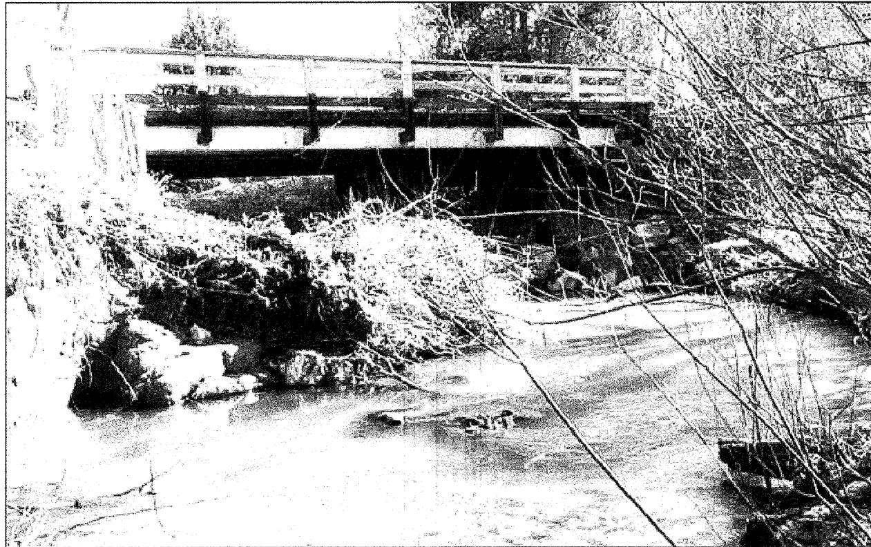
Photo 1: Looking North (Downstream) at bridge. Note scouring of stream bank in lower left-hand portion of photo.
