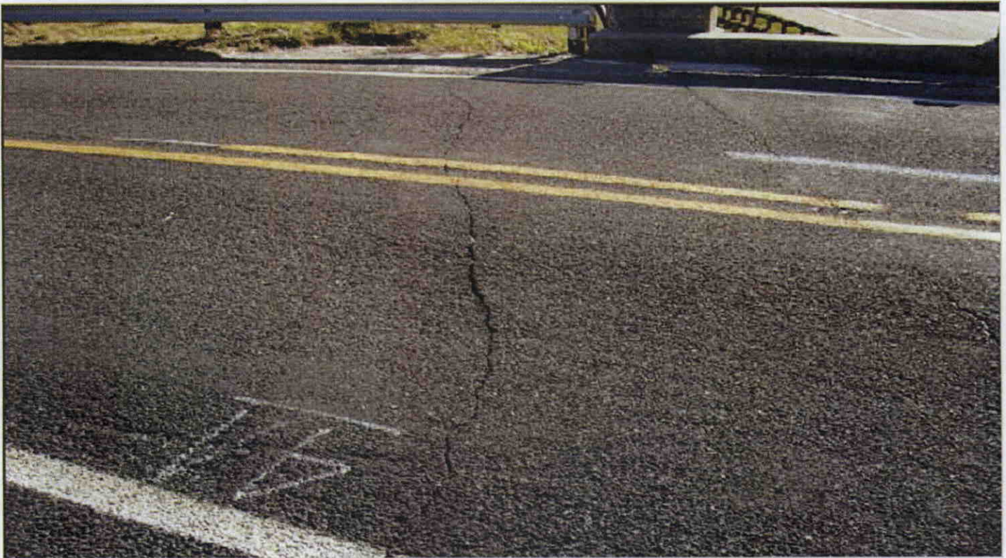
TRANSVERSE CRACK IN ASPHALT WEARING SURFACE EAST APPROACH
