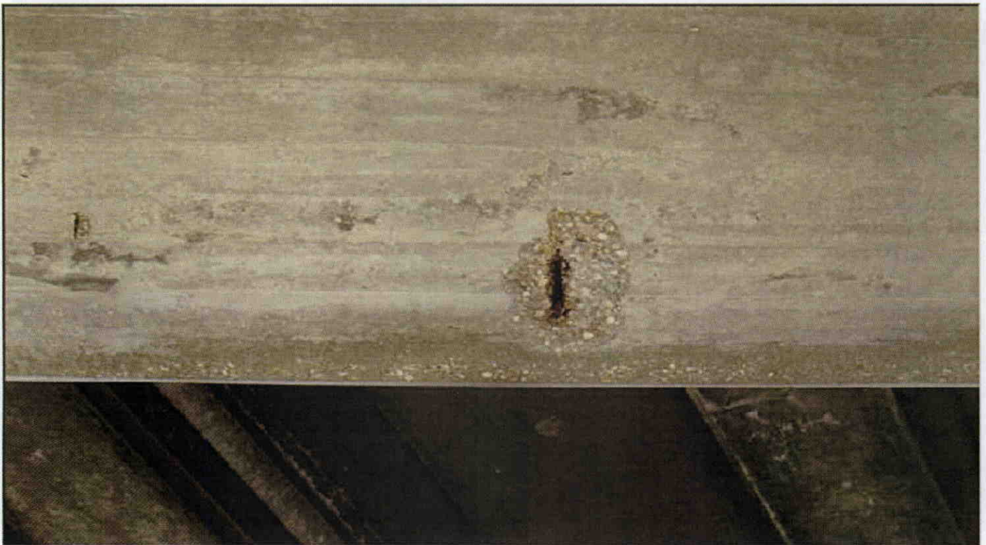
13 IN. X 9 IN. SPALL WITH EXPOSED REBAR ON BOTTOM OF BENT 1 CAP BETWEEN COLUMNS
