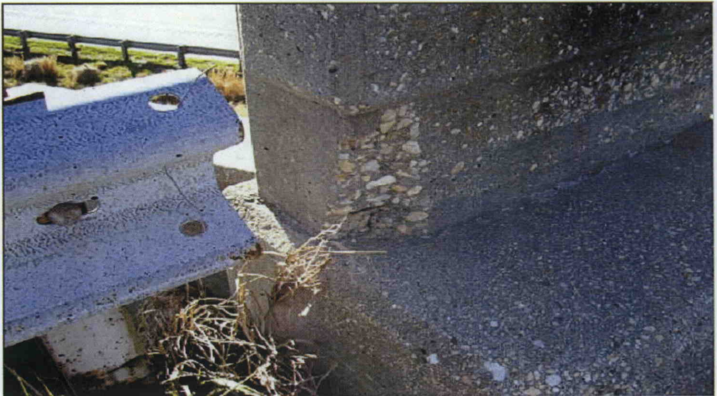
9 IN. X 4 IN. SPALL ON RAIL END POST AT SOUTHEAST CORNER
