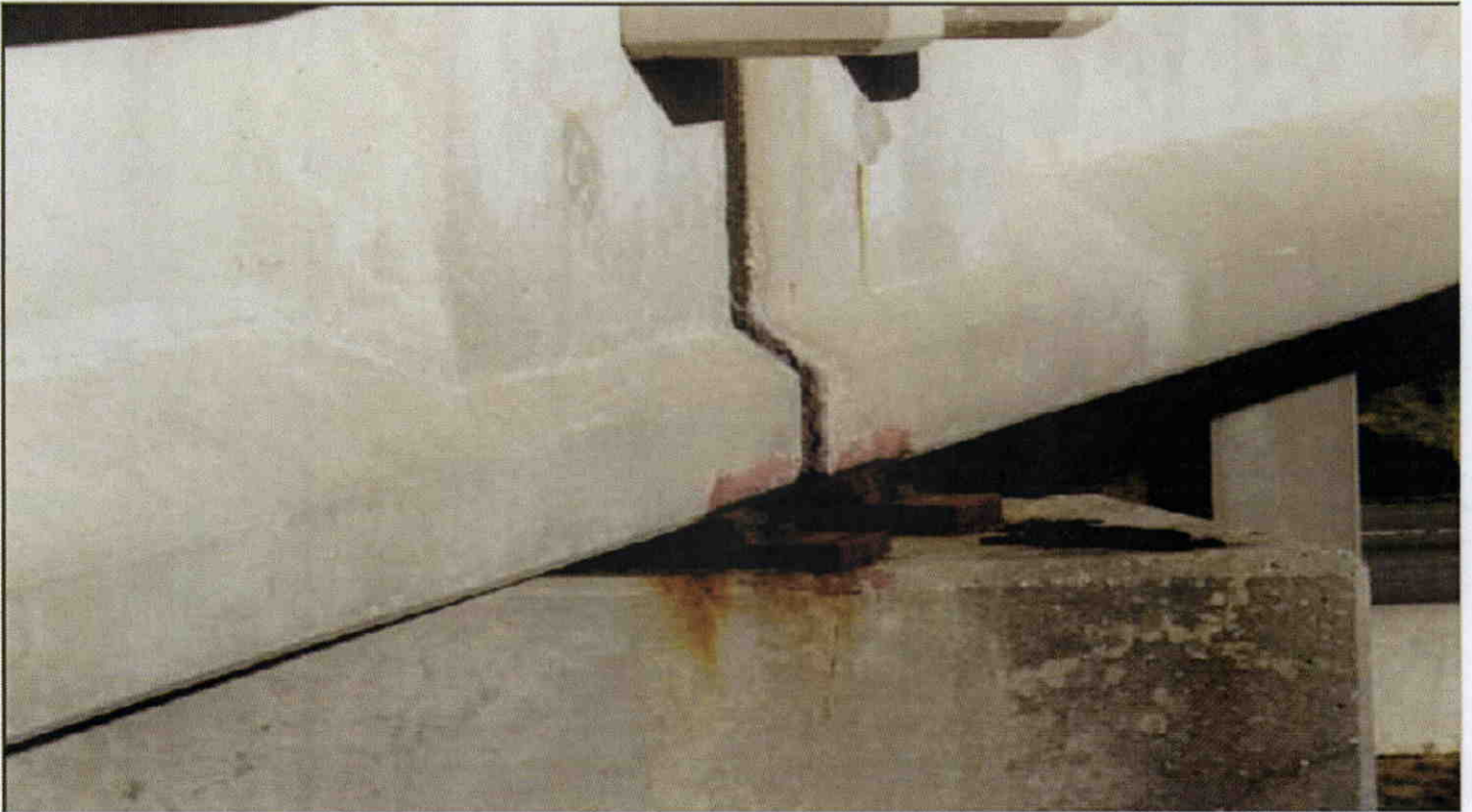
SURFACE RUST ON BEARING PLATES AT INTERIOR BENT 1 AT GIRDER 4
