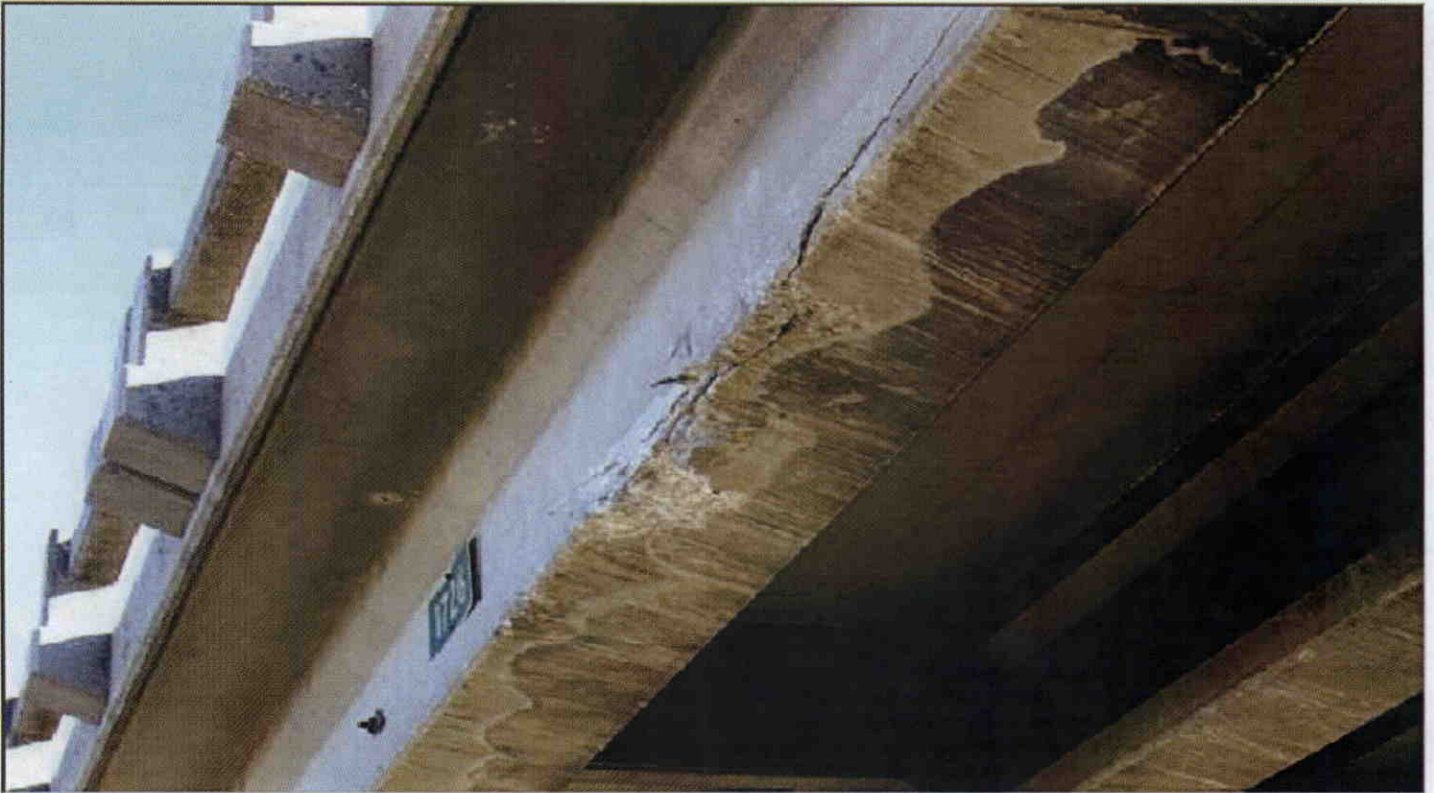
SPALL 2 FT. X 10 IN. X 3 IN. DEEP WITH 2 EXPOSED CABLES WITH SOME STRANDS BROKEN ON BOTTOM FLANGE OF GIRDER 1 OVER 95 SOUTH BOUND. CAUSED BY VEHICULAR
