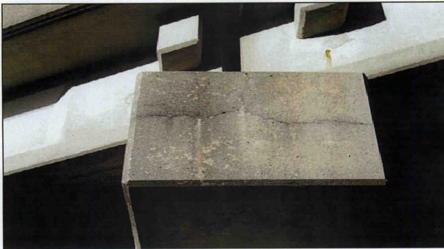
VERTICAL AND HORIZONTAL HAIRLINE TO 1/32 IN. CRACK ON SOUTH END OF BENT 1 CAP
