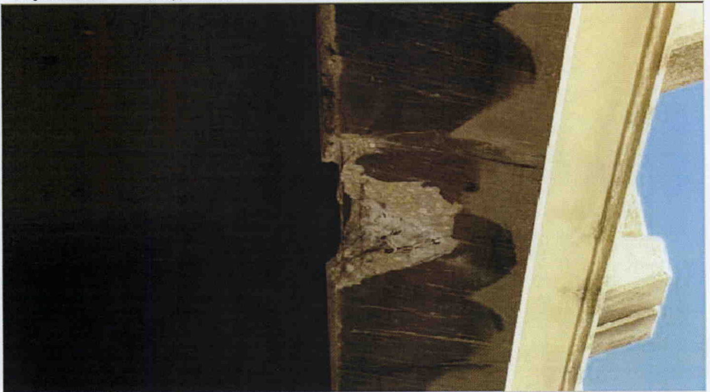
SPALL 14 IN. X 10 IN. X 4 IN. DEEP ON BOTTOM OF GIRDER 4 WITH 5 EXPOSED CABLES. 3 BOTTOM CABLES SHEARED INTO OVER 95 SOUTH BOUND. LONGITUDINAL
