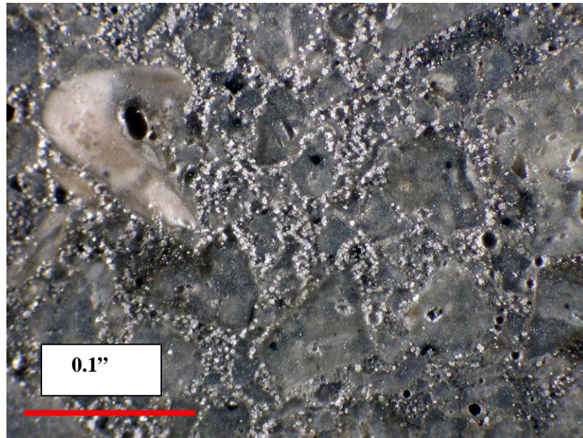
Figure 14. On drying, salt crystals appeared on the lapped concrete surface near the outside end of the core.
