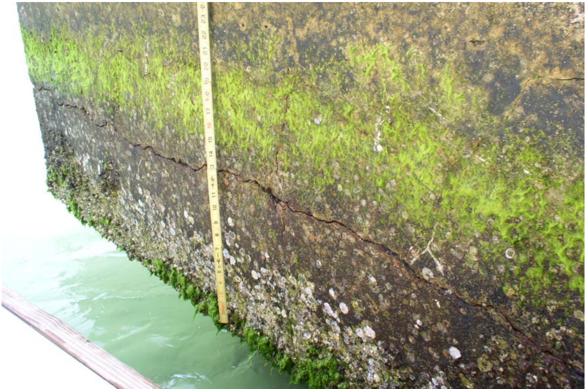
PHOTO 28: CRACKING IN NORTH END OF EAST "NEW" CAP AT BENT 171
