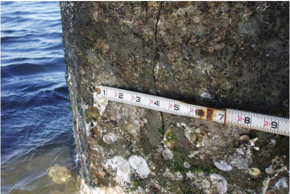
PHOTO 4: TYPICAL VERTICAL CRACKING AT PILE 6 OF BENT 55
