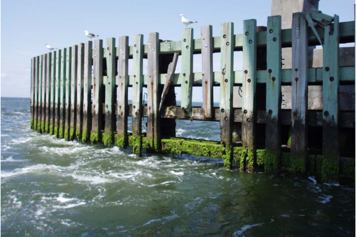
PHOTO 35: DAMAGED TIMBER RUB STRIPS NEAR THE WEST END OF THE NORTH FENDER.
