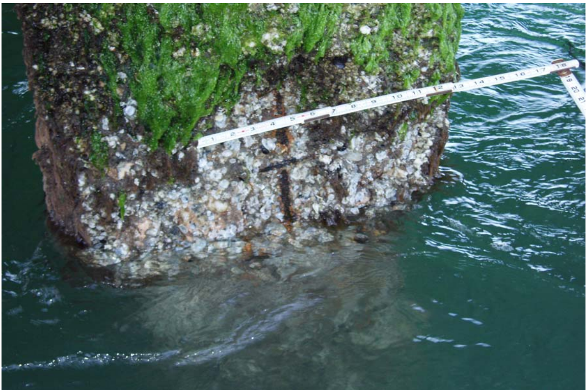
PHOTO 18: SPALLING IN TIDAL ZONE AT PILE 16 OF BENT 146
