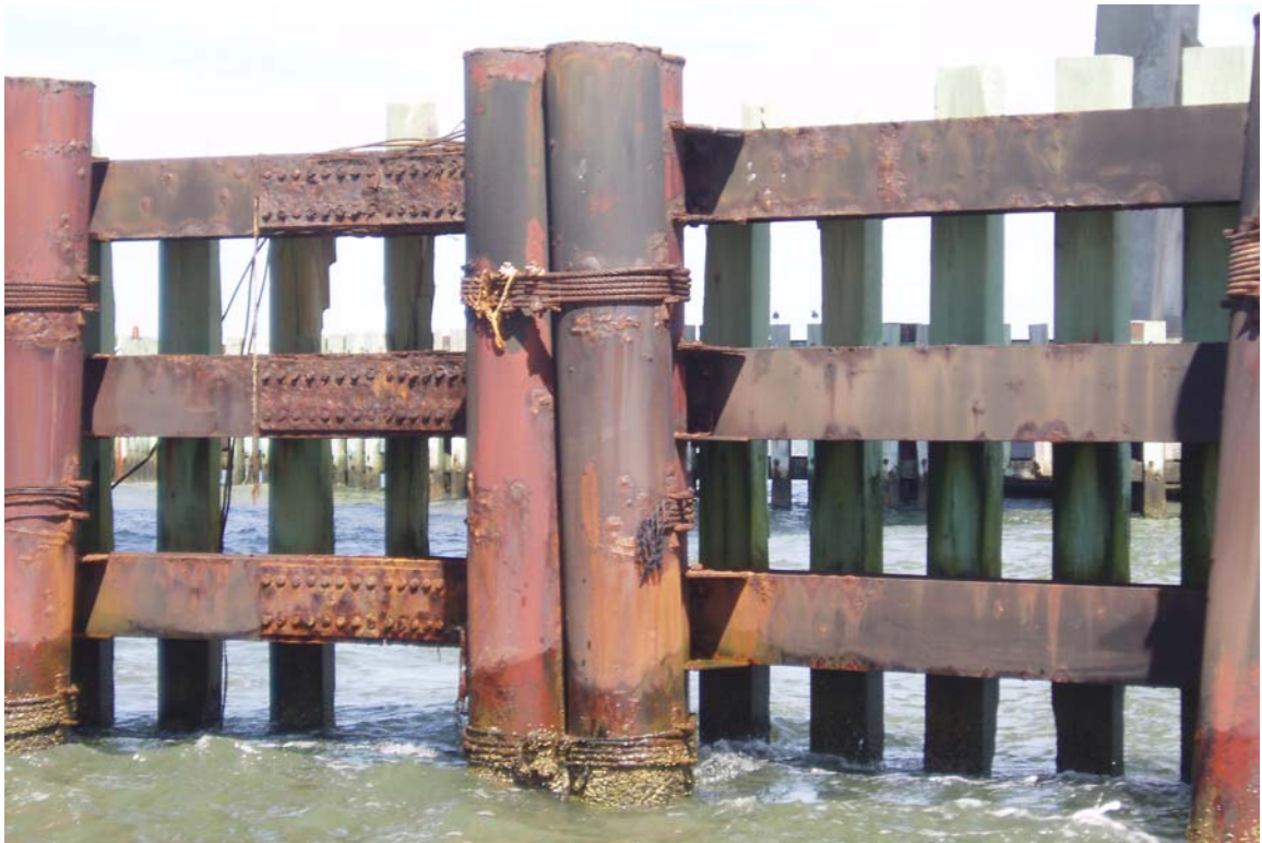
PHOTO 34: TYPICAL CORROSION ON STEEL ELEMENTS OF FENDER SYSTEM ABOVE THE HIGH WATER MARK, SOUTH FENDER SHOWN
