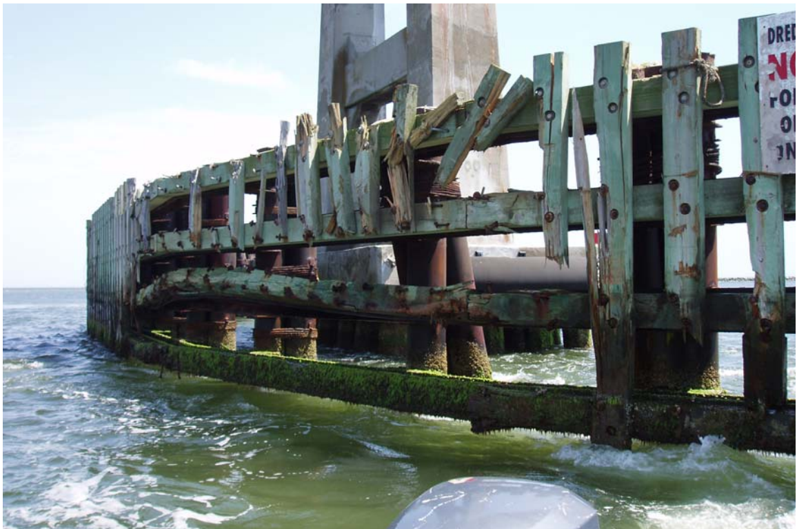
PHOTO 38: IMPACT DAMAGE BETWEEN PILE CLUSTERS 10 AND 13 OF THE SOUTH FENDER
