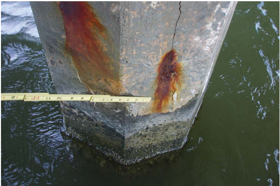
PHOTO 2: CRACKING TO 1/8 IN. WIDE WITH CORROSION STAINS AT PILE 4 OF BENT 95
