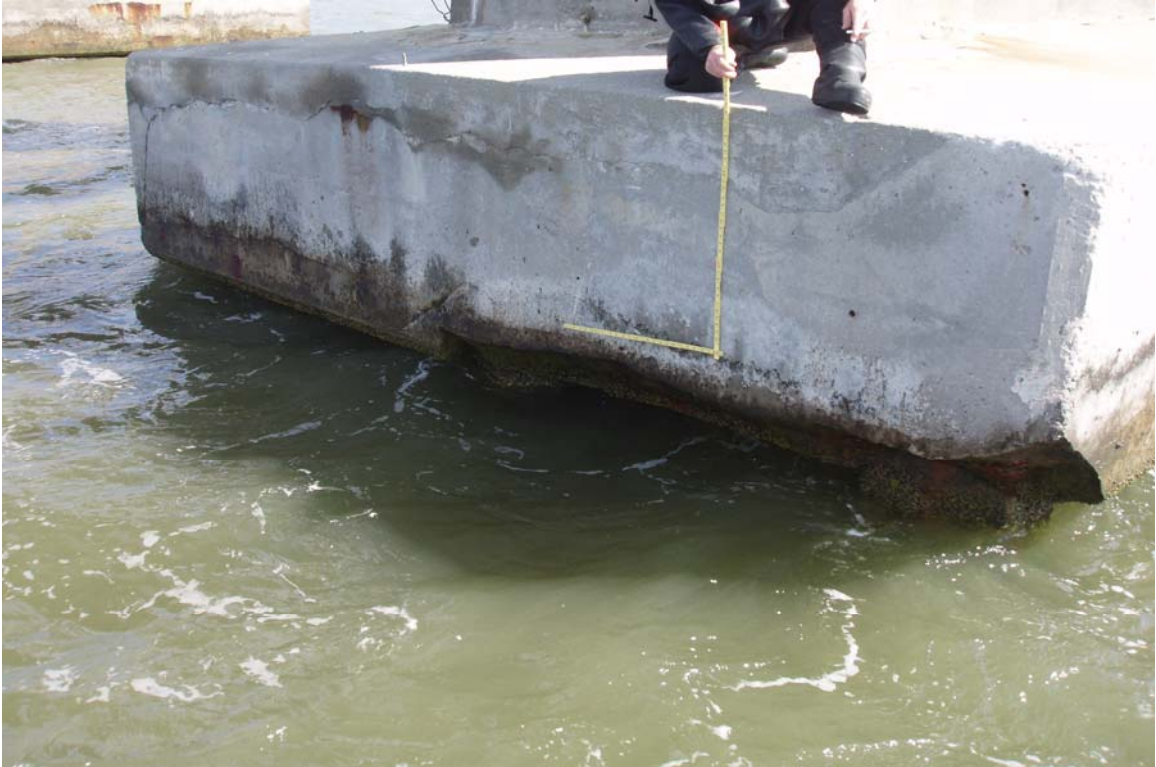
PHOTO 9: SPALL IN LOWER WEST EDGE OF BENT 143
