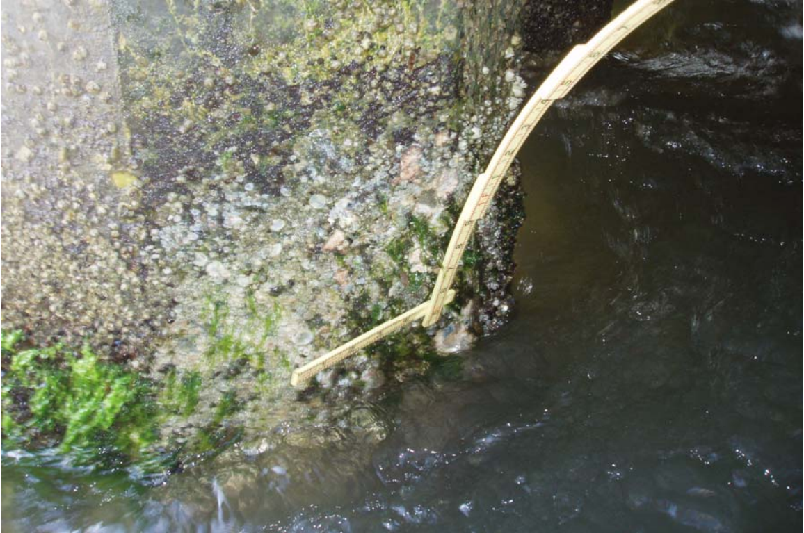
PHOTO 21: SPALL IN TIDAL ZONE AT PILE 9 OF BENT 144
