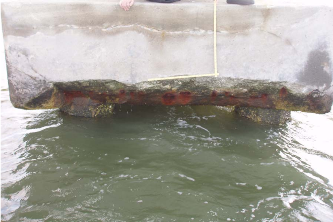
PHOTO 10: SPALL IN LOWER WEST EDGE OF BENT 159
