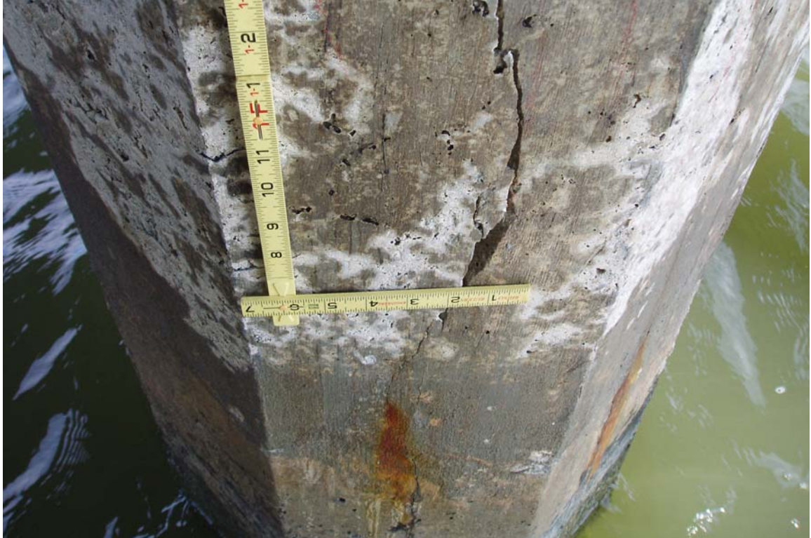
PHOTO 1: CRACKING TO 1/8 IN. WIDE WITH CORROSION STAINS AT PILE 3 OF BENT 95
