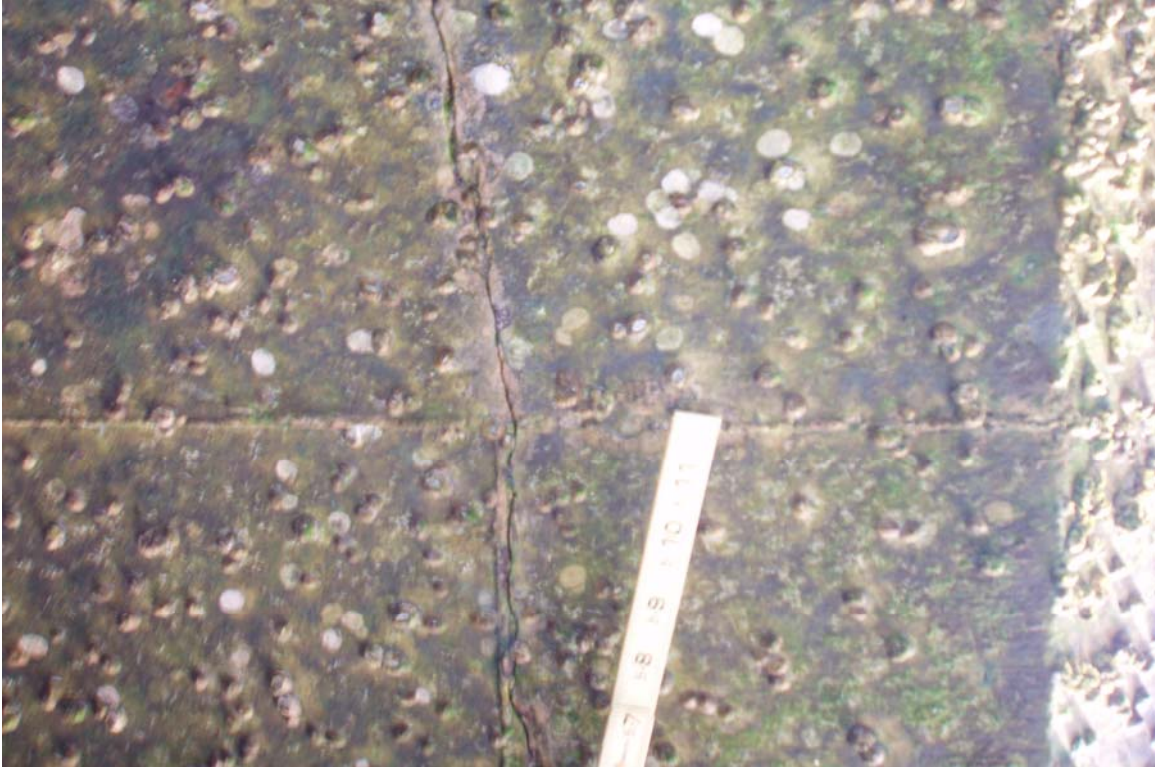
PHOTO 13: CRACKING IN UNDERSIDE OF BENT 147 PILE CAP
