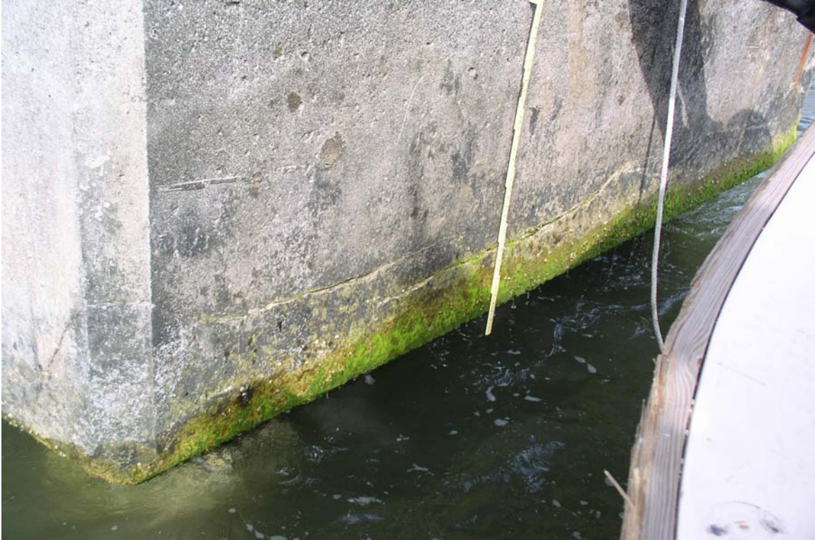
PHOTO 15: HORIZONTAL CRACKING IN LOWER PORTION OF EAST FACE OF BENT 159 PILE CAP, TYPICAL
