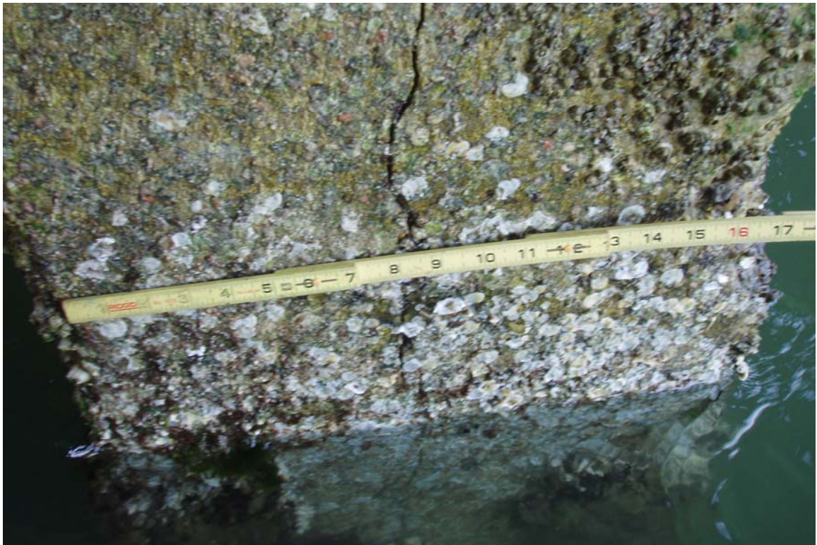
PHOTO 30: CRACK IN FACE 4 (WEST FACE) AT PILE 6 OF BENT 186
