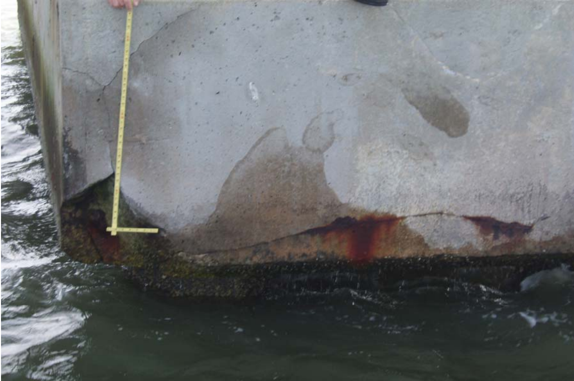
PHOTO 11: SPALL IN LOWER NORTHWEST CORNER OF BENT 164
