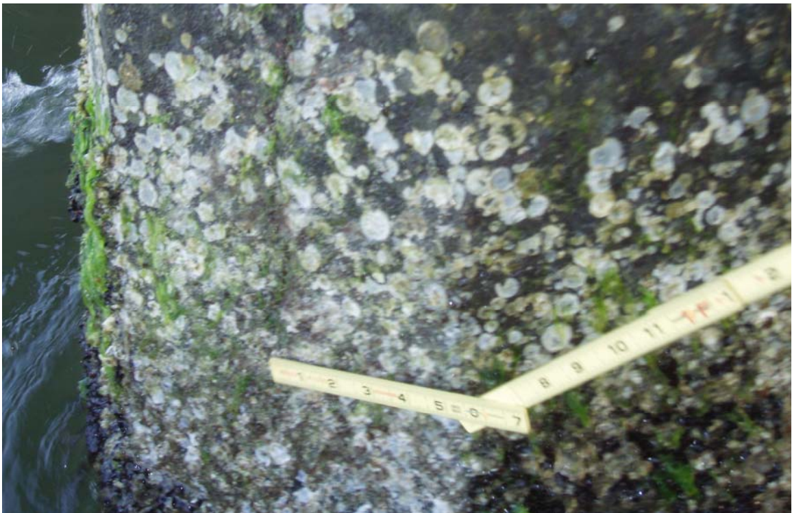
PHOTO 22: VERTICAL CRACKING IN THE TIDAL ZONE AT PILE 10 OF BENT 160
