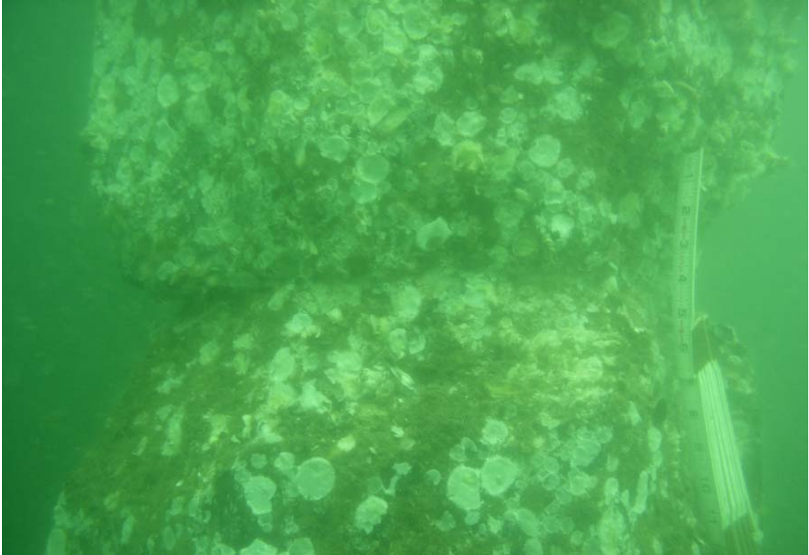
PHOTO 25: DETERIORATED SPLICE IN MID WATER COLUMN AT PILE 7 OF BENT 159
