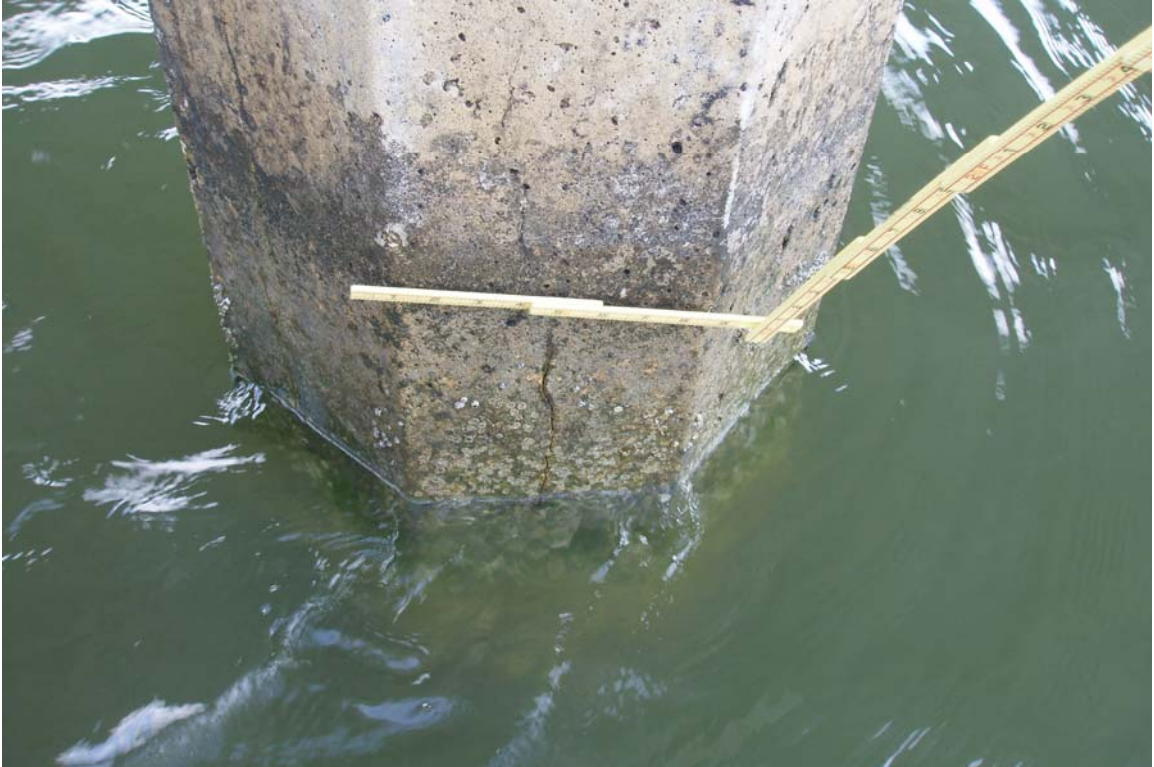
PHOTO 3: TYPICAL VERTICAL CRACKING AT PILE 1 OF BENT 106
