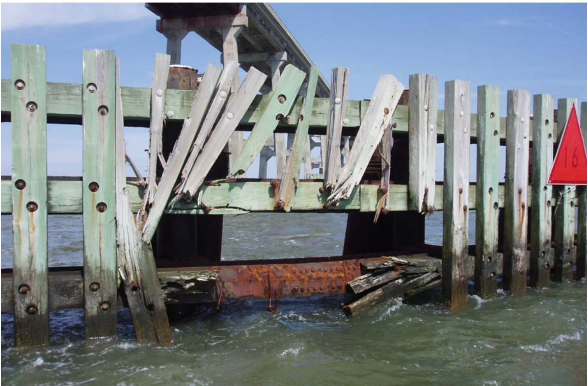
PHOTO 36: DAMAGED TIMBER RUB STRIPS AND BACKING TIMBER, NORTH FENDER SHOWN BETWEEN CLUSTERS 2 & 3
