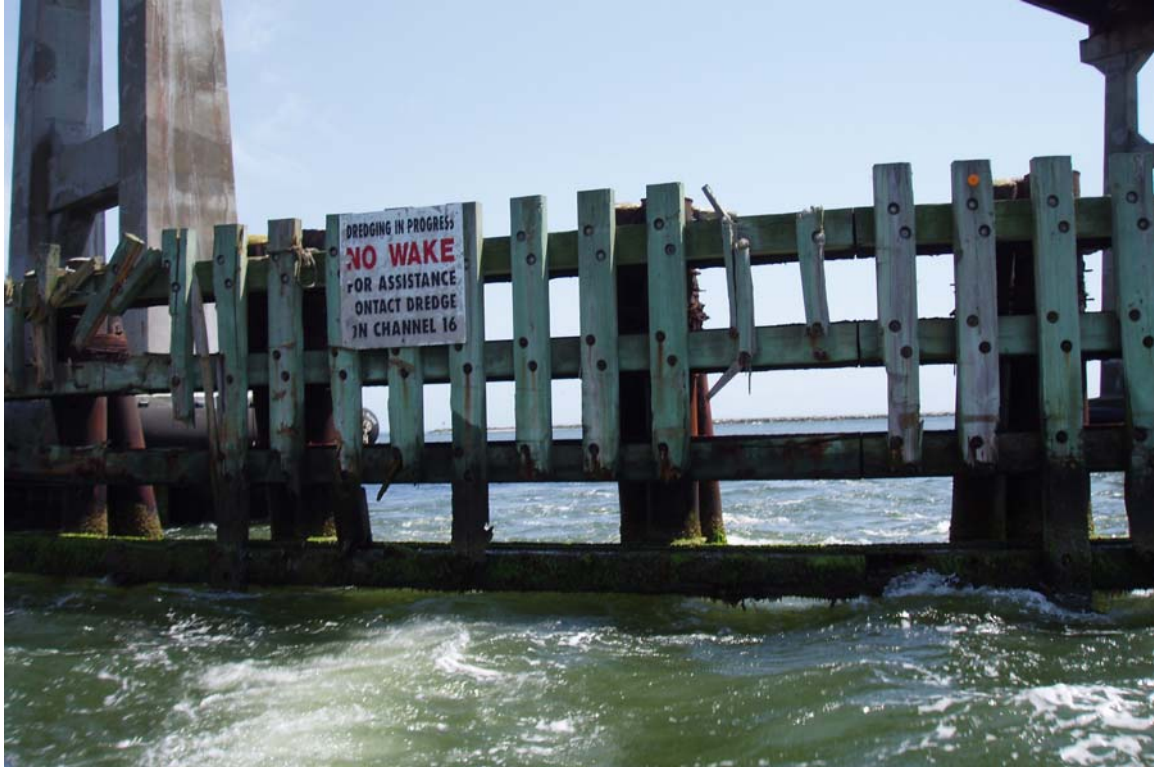
PHOTO 39: DAMAGED/MISSING TIMBER RUB STRIPS IN THE WEST END OF THE SOUTH FENDER
