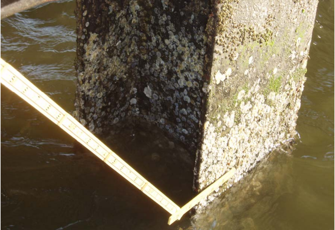
PHOTO 7: TYPICAL CONDITION OF STEEL H-PILE IN TIDAL ZONE (PILE I OF BENT 115 SHOWN)
