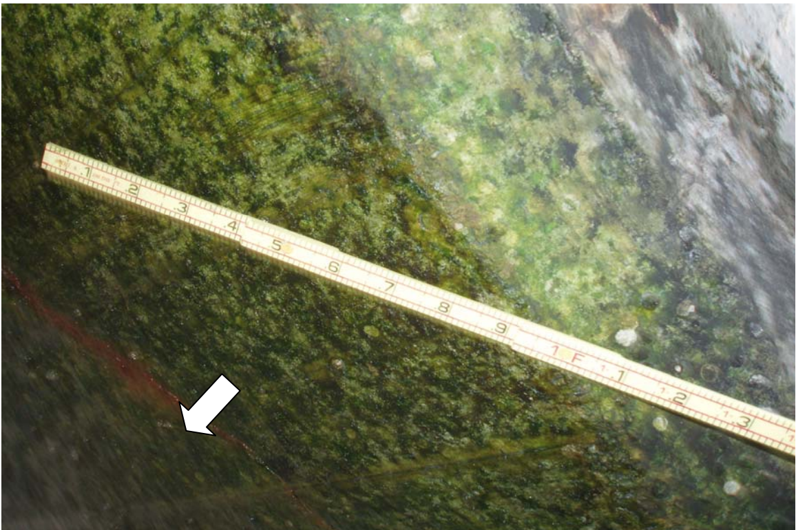
PHOTO 14: CRACKING IN UNDERSIDE OF BENT 160 PILE CAP
