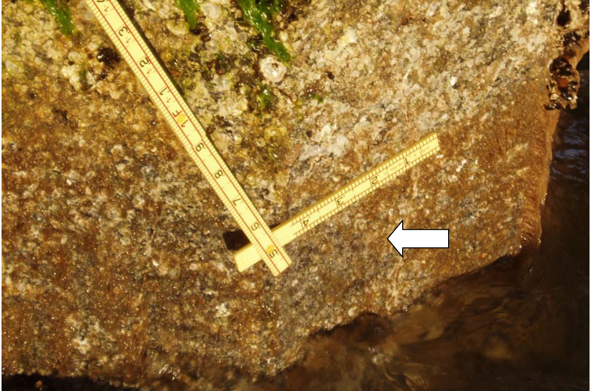
PHOTO 23: VERTICAL CRACKING IN THE TIDAL ZONE AT PILE 9 OF BENT 163
