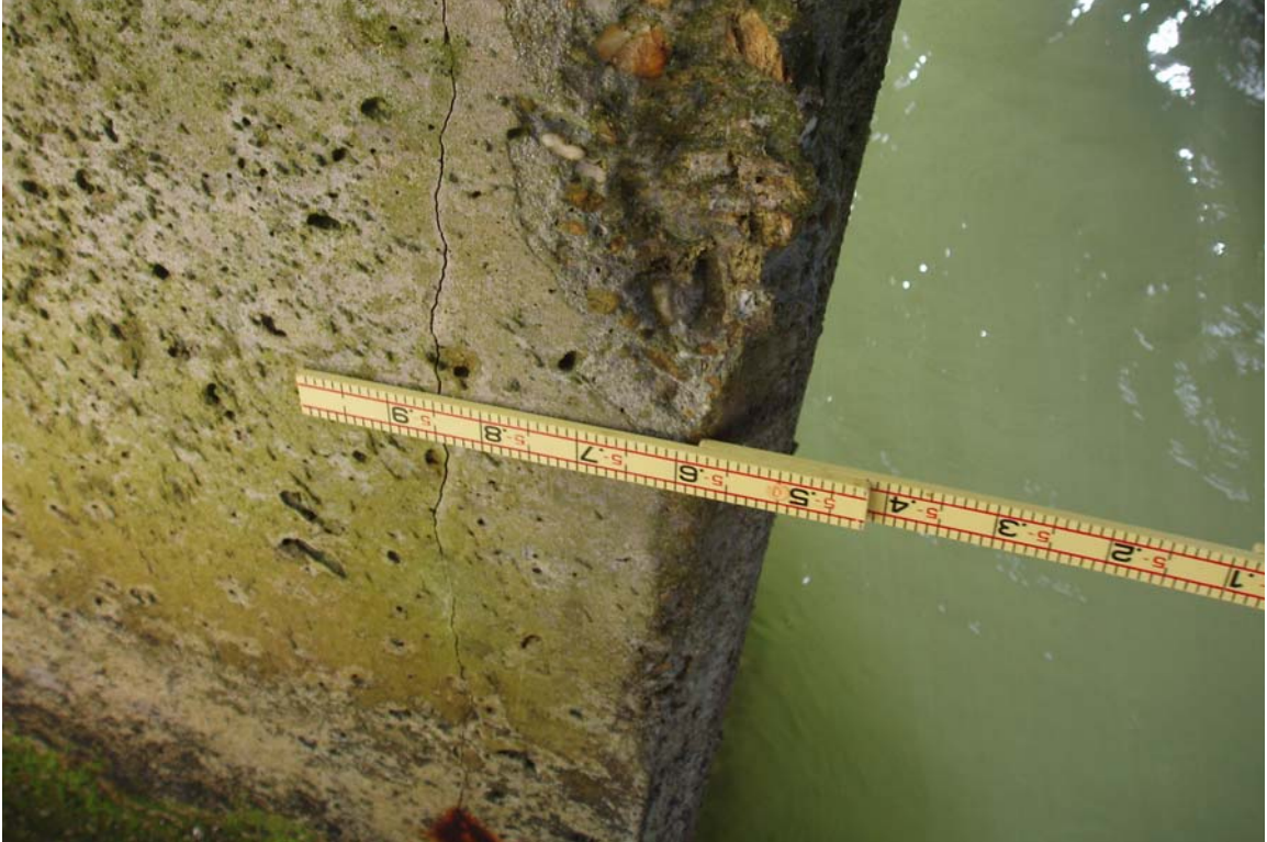
PHOTO 31: DELAMINATED SOUTHWEST EDGE AT PILE 1 OF BENT 174
