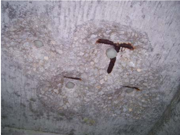
Span 129-130, spall & ER at North end
