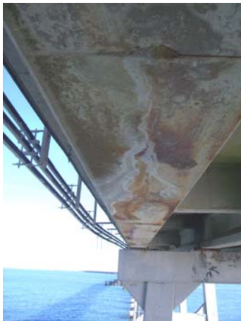
Span 131-132; CSagg along Girder bottom, typ.
