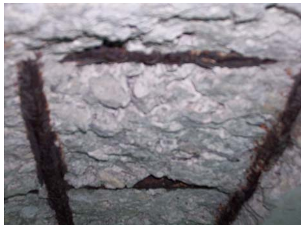
Span 134-135; SP & ER at soffit South end
