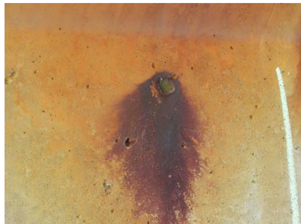
Span 131-132, Corroded Aggregate in girder
