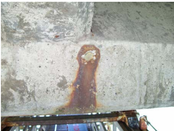
Span 149-150; CS agg on Girder #2, East side,
