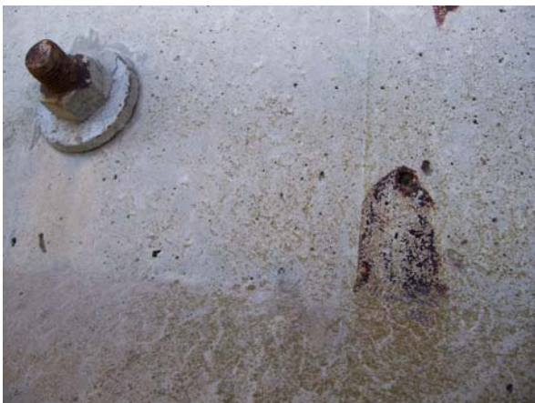
Span 139-140; CSagg on Girder #1, East side,
