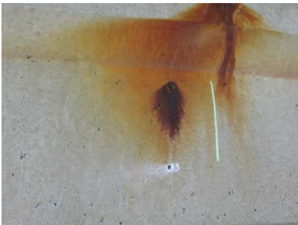
Span 131-132, Corroded Aggregate in girder
