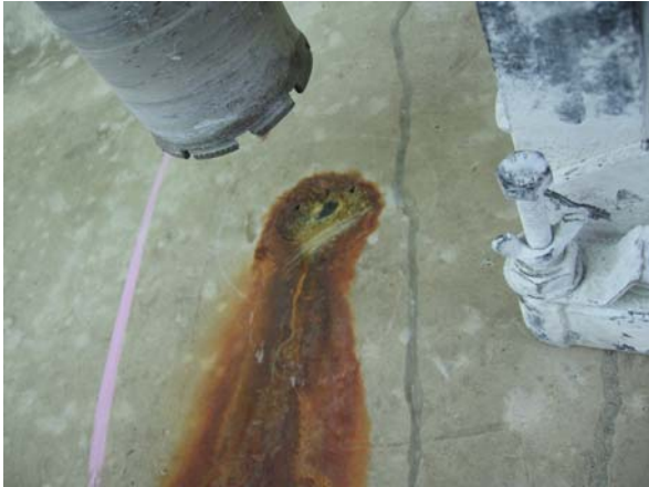
Span 161-162, Girder #3 corroded aggregate
