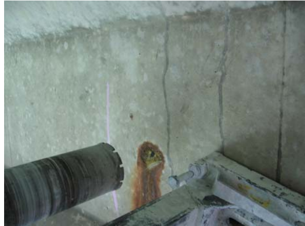
Span 161-162, Girder #3 corroded aggregate
