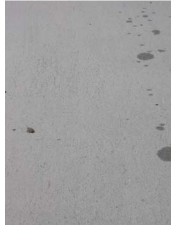
Span 129-130: mapped cracking south end
