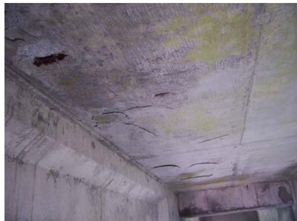
Span 149-150; ER on soffit, West bay, North
