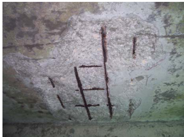
Span 134-135; SP & ER at soffit South end
