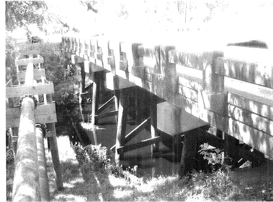
Photograph No. 7: This photograph was taken from the right side of the -EL- alignment, looking northwest, along the right side of the existing bridge.
