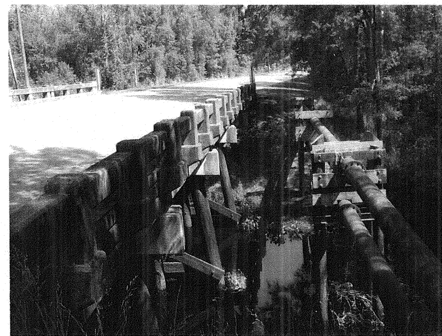
Photograph No. 4: This photograph was taken from the right side of the -EL- alignment, looking southeast, along the right side of the existing bridge.
