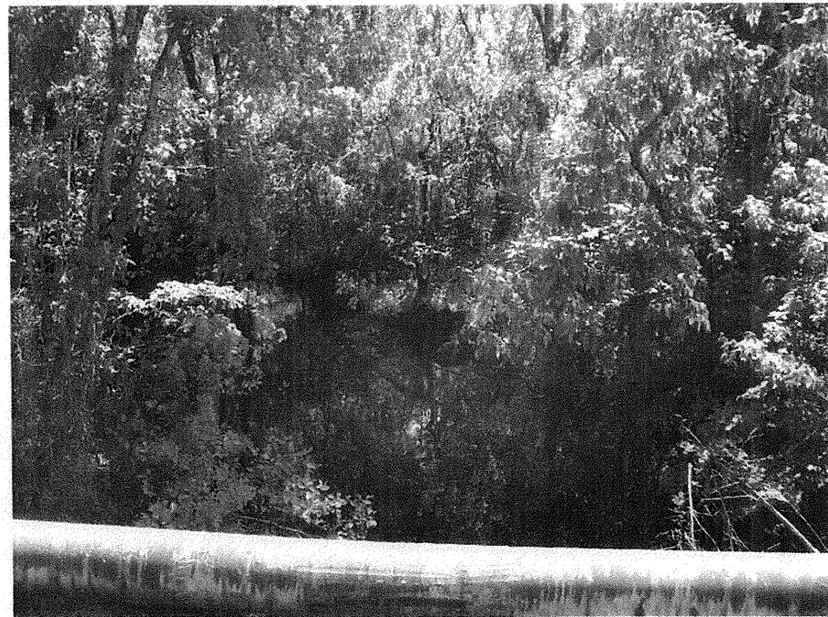
Photograph No. 6: This photograph was taken from the existing bridge, looking southwest (upstream).
