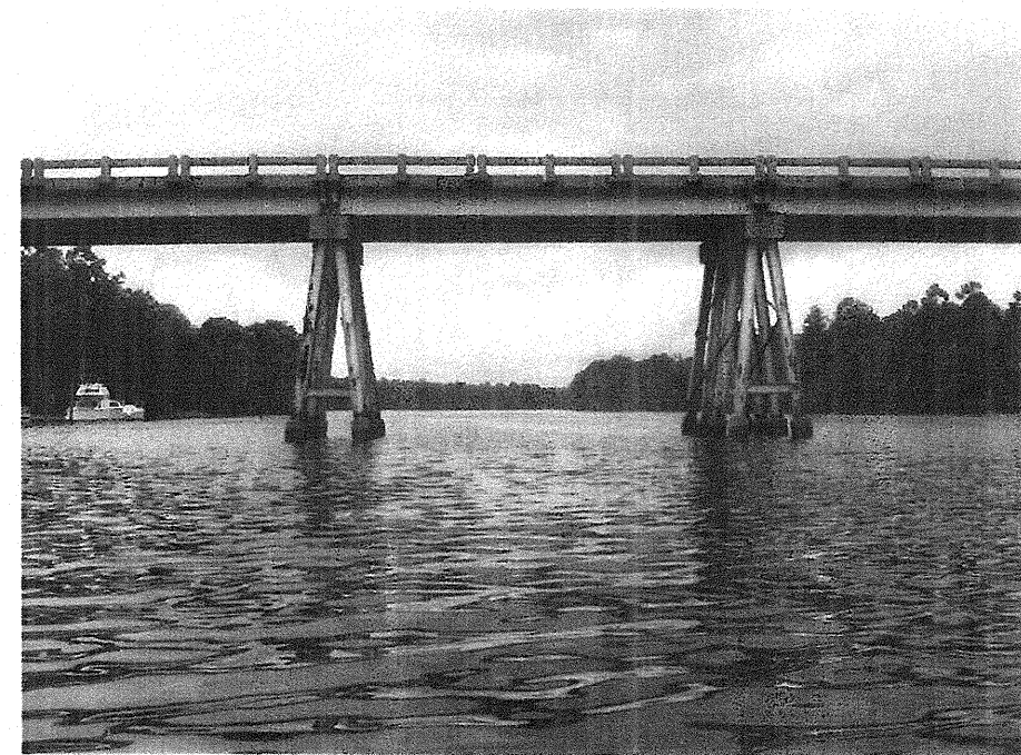
Photograph No. 8: This photograph was taken from the right side of the -L- alignment, looking north, across proposed Interior Bent No. 3.
