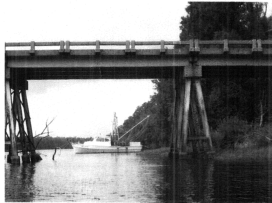
Photograph No. 11: This photograph was taken from the right side of the -L- alignment, looking north, across proposed Interior Bent No. 6.
