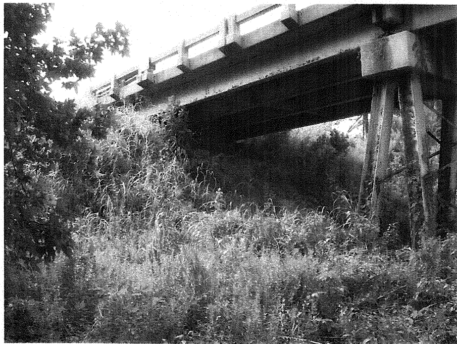
Photograph No. 6: This photograph was taken from the right side of the -L- alignment, looking north, across proposed Interior Bent No. 1.
