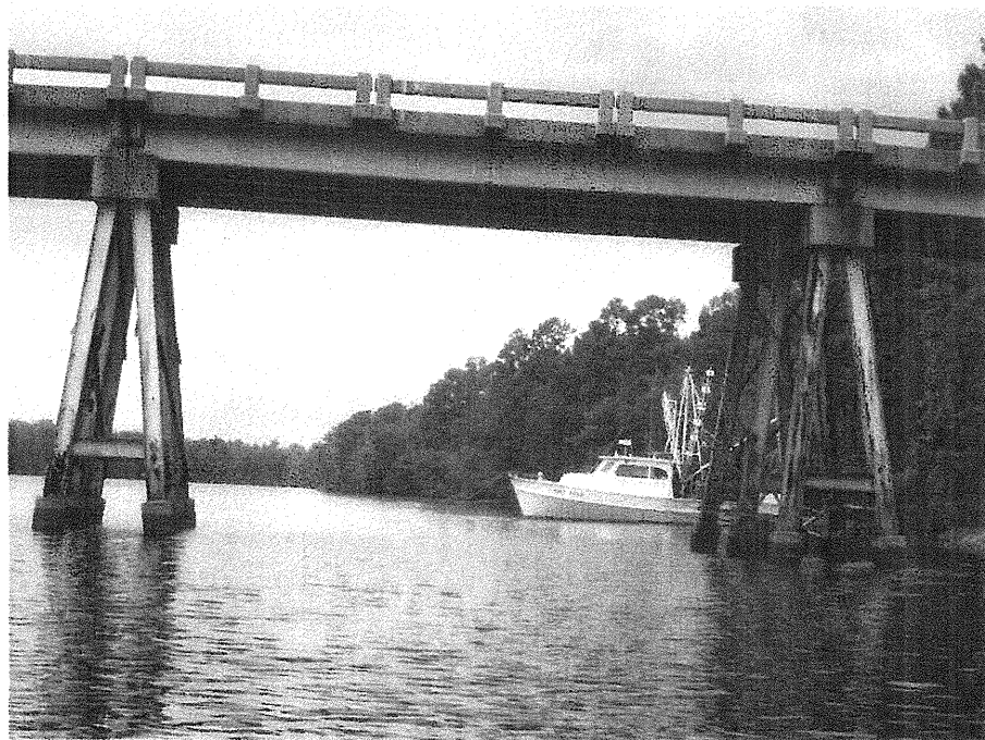
Photograph No. 10: This photograph was taken from the right side of the -L- alignment, looking north, across proposed Interior Bent No. 5.
