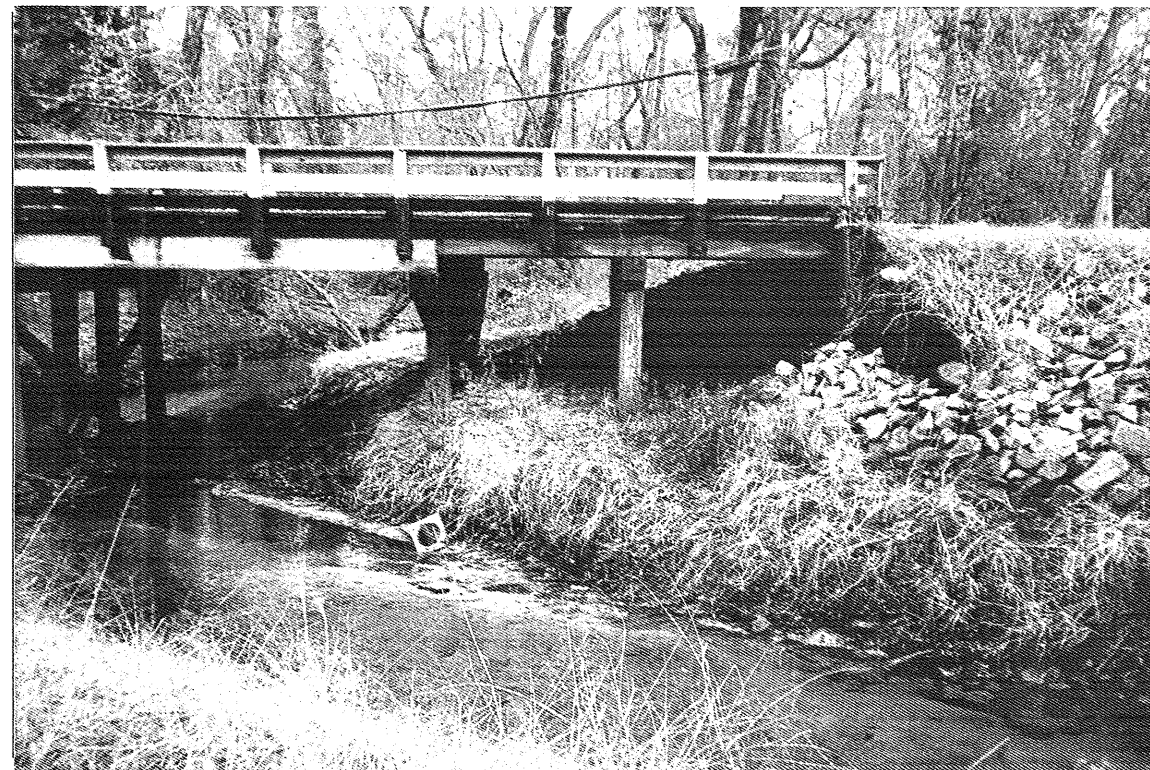
Photograph No. 6: Looking north along bent 2, located at the third guardrail post from right.
