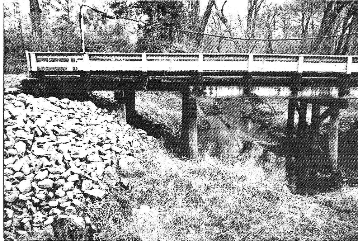
Photograph No. 5: Looking north along bent 1, located at the third guardrail post from left.
