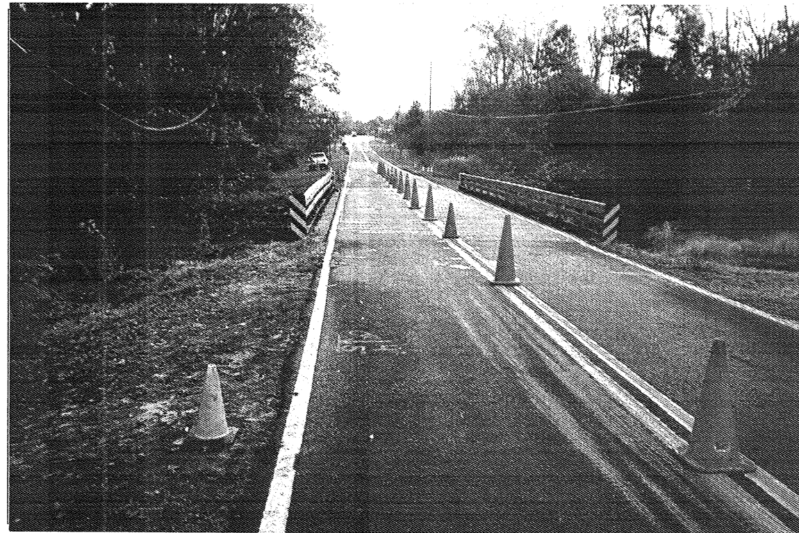
Photograph No. 2: Looking east toward Hookerton along SR 1438. End bent 1 at first cone in foreground.
