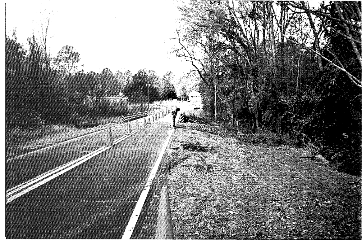
Photograph No. 3: Looking west along SR 1438. End bent 2 at first cone in center of road. People standing at bent 3.
