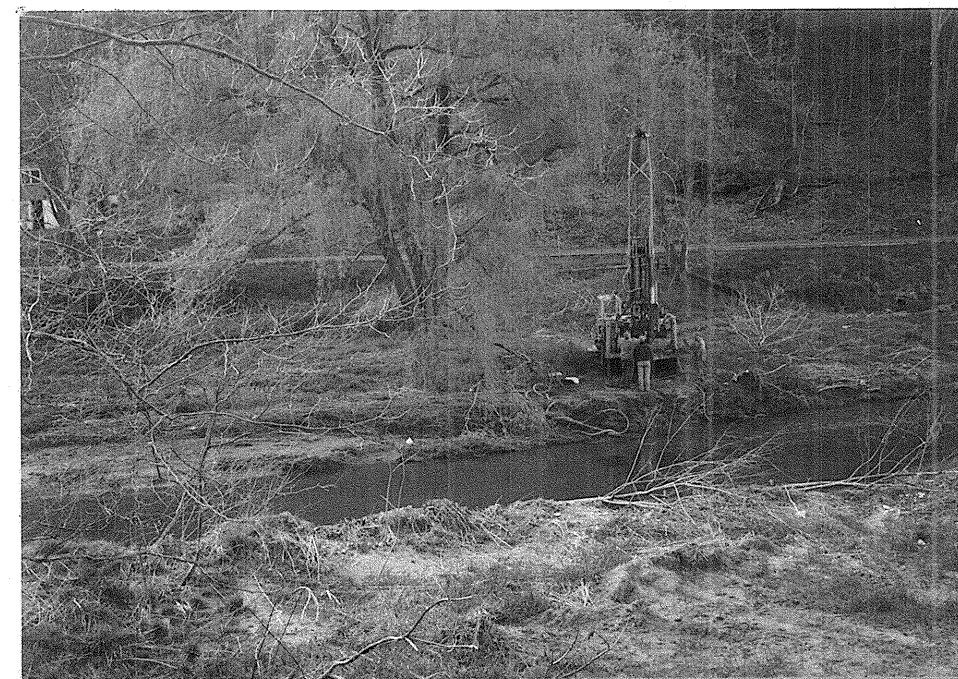
Figure 3. Drilling on B1-A. View looking back along -L- from shoulder of US 321.
