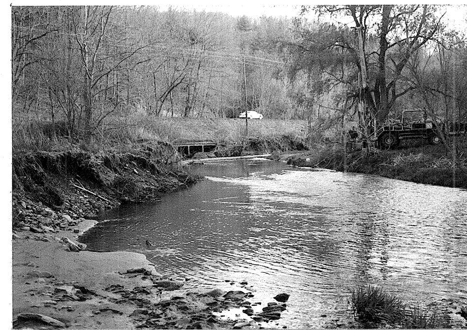
Figure 4. View looking upstream across -L-. Drilling on B1-A. Note fresh erosion on stream bank at B2 and at base of US 321 embankment.
