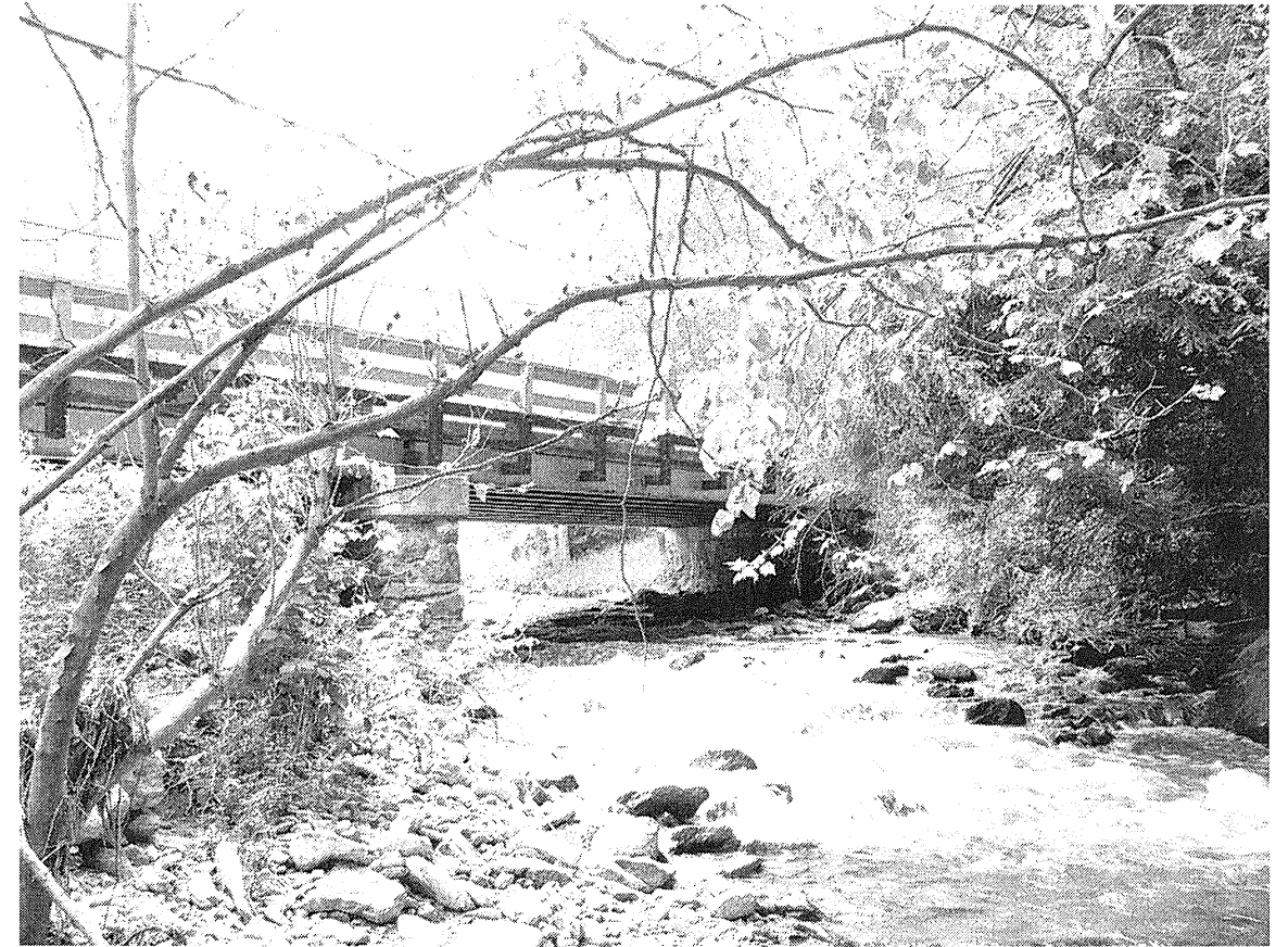
DOWNSTREAM FACE, INTERIOR BENT AND SOUTH END BENT. MADISON COUNTY BRIDGE NUMBER 30, NC-209 OVER SPRING CREEK
