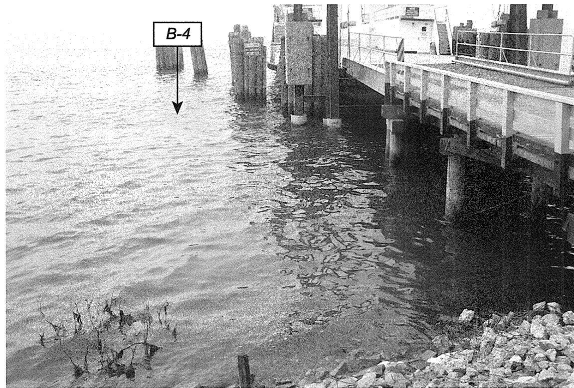
Photograph 6: View to Southwest showing approximate location of boring B-4 at the Knotts Island Ferry Dock site.
