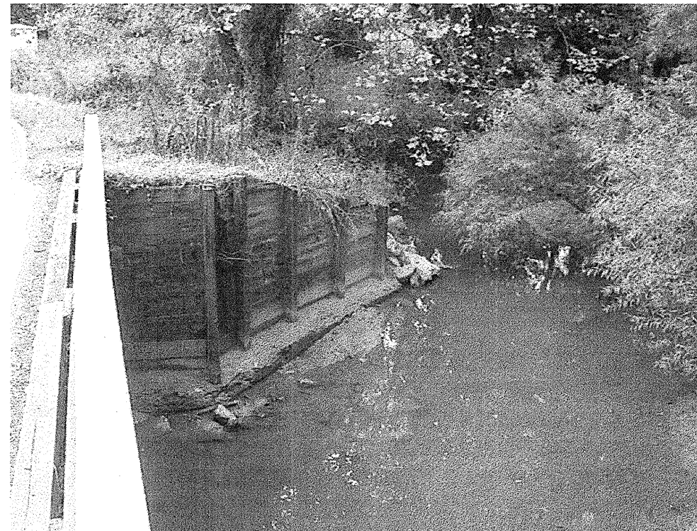
UPSTREAM VIEW SHOWING LONG WING WALL AND BOULDER BACKFILL ON SW CORNER OF BRIDGE
