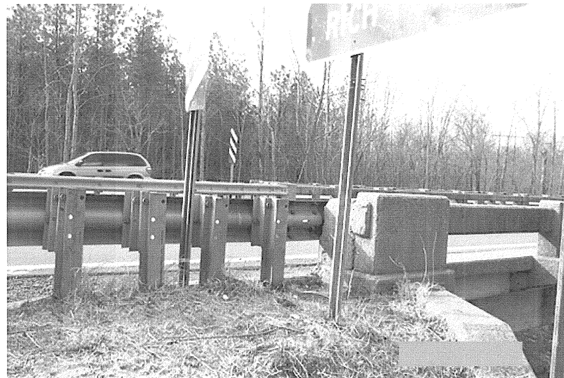
Photograph 6: View Along End Bent-2 From Left to Right From Top of Embankment
