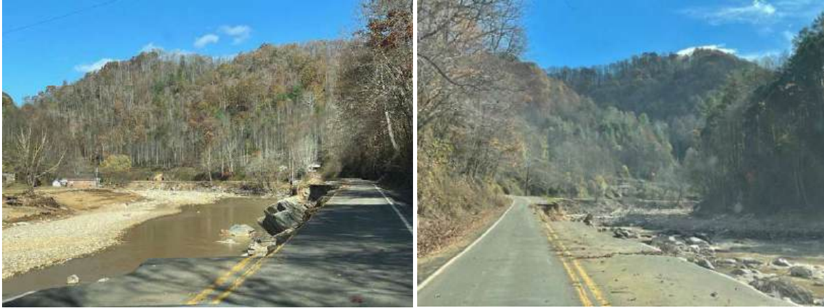
Figures 2-4. October 31, 2024 images of damaged portions of US 19W along Cane River within action area
