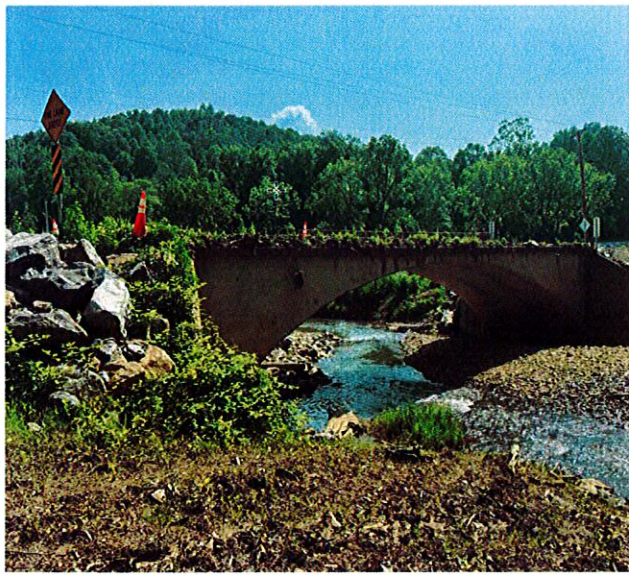
Bridge 171 (YC0250)- Post-Helene Photographs
