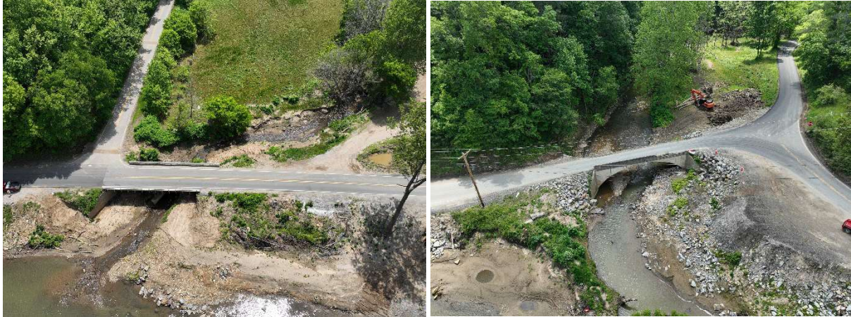
Figures 2-4. 2025 Images of temporarily repaired portions of NC 197 within action area. Photos courtesy of Dave McHenry and NCDOT.
