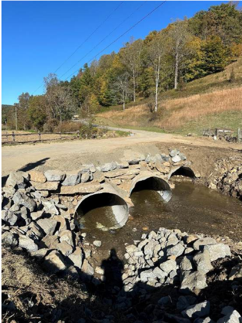
Figure 5. Damage to Culvert 449 from Hurricane Helene. South side of culvert, looking north. Note debris has been removed and temporary road repair has occurred. NCDOT Hurricane Helene All Imagery/Drone Map, December 30, 2024.
