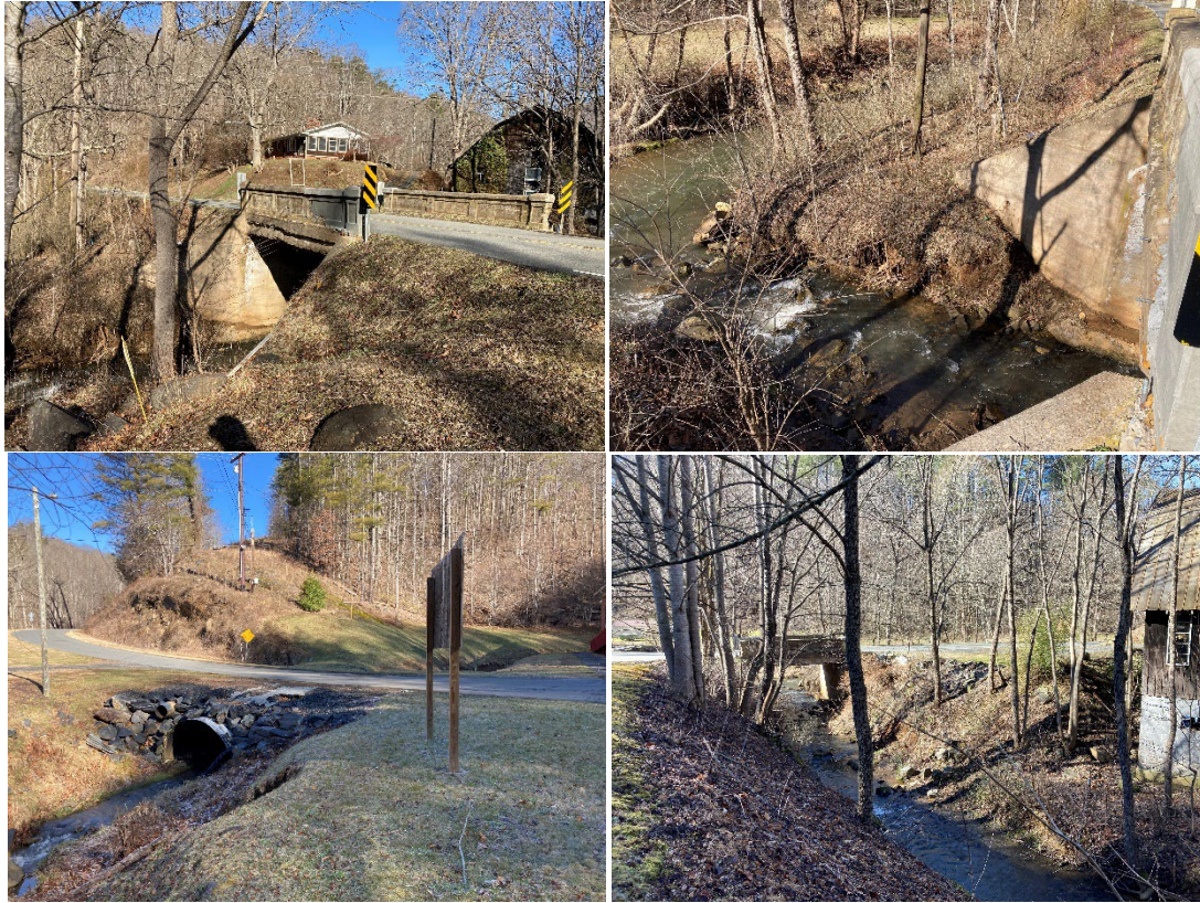
Figure 1. Photos of the Action Area. Bridge 19 over Cub Creek, the confluence of Cub and Cane Creek, the Sweet Creek Road culvert, and Cub Creek and trees that will be removed upstream of Bridge 19.
