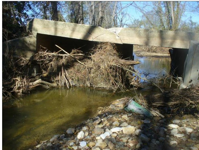
PAR: CULVERT HAS COLLAPSED
