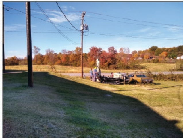
Photo 4. Carolina Soil Investigations using the Geoprobe to drill boring B-5 in the PUE along Little Mountain Road.
