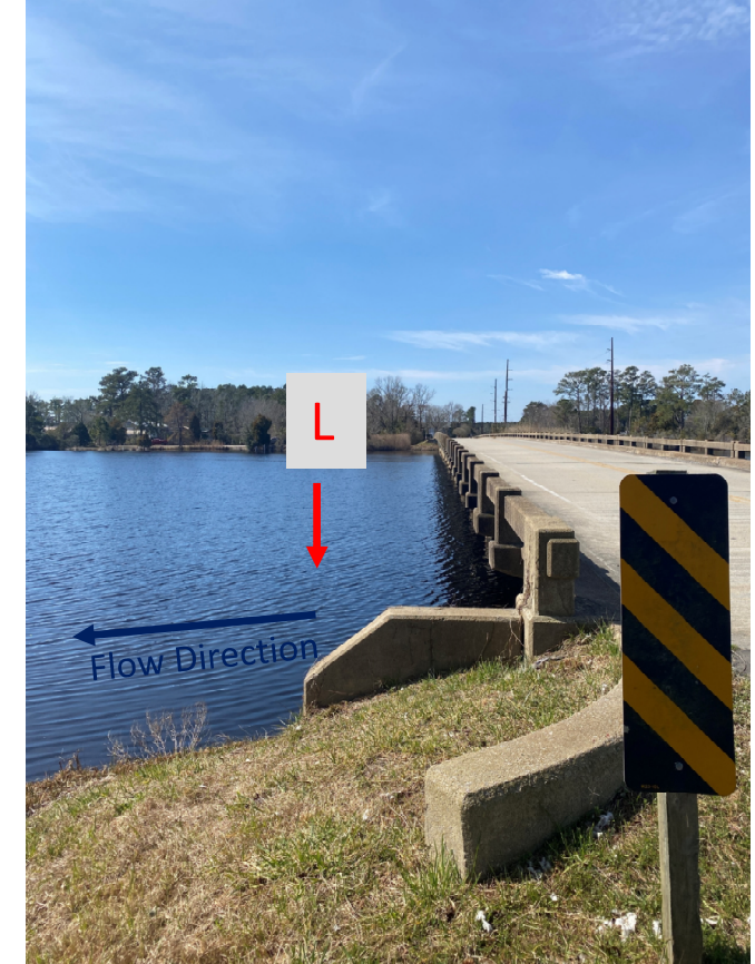
-EB2 facing downstation-
