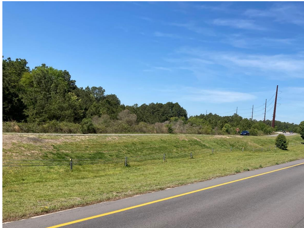
A. Photograph of median showing differential settlement as evident by variation in guardrail height, looking west from northbound lanes.
