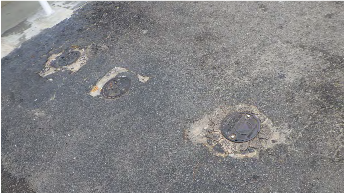
Multiple monitoring wells
