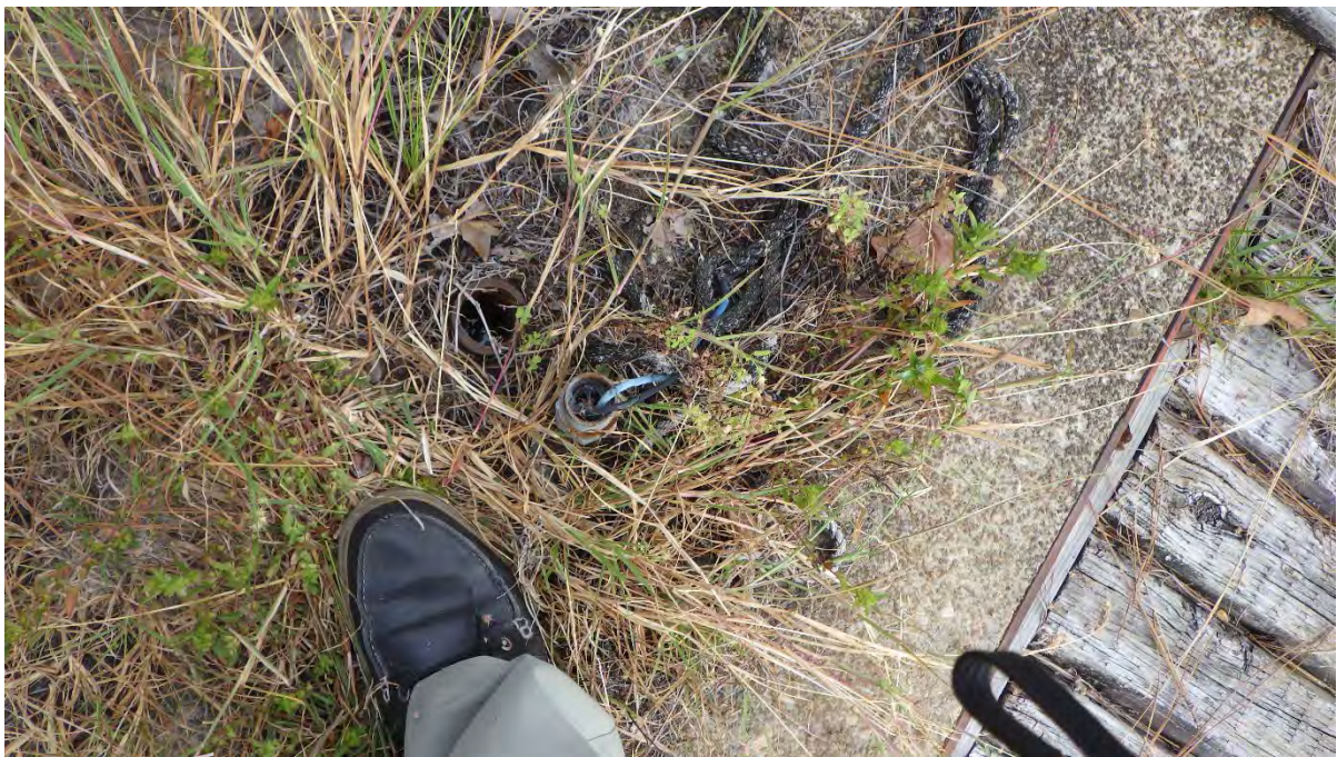
Possible abandoned UST product line/pipe
