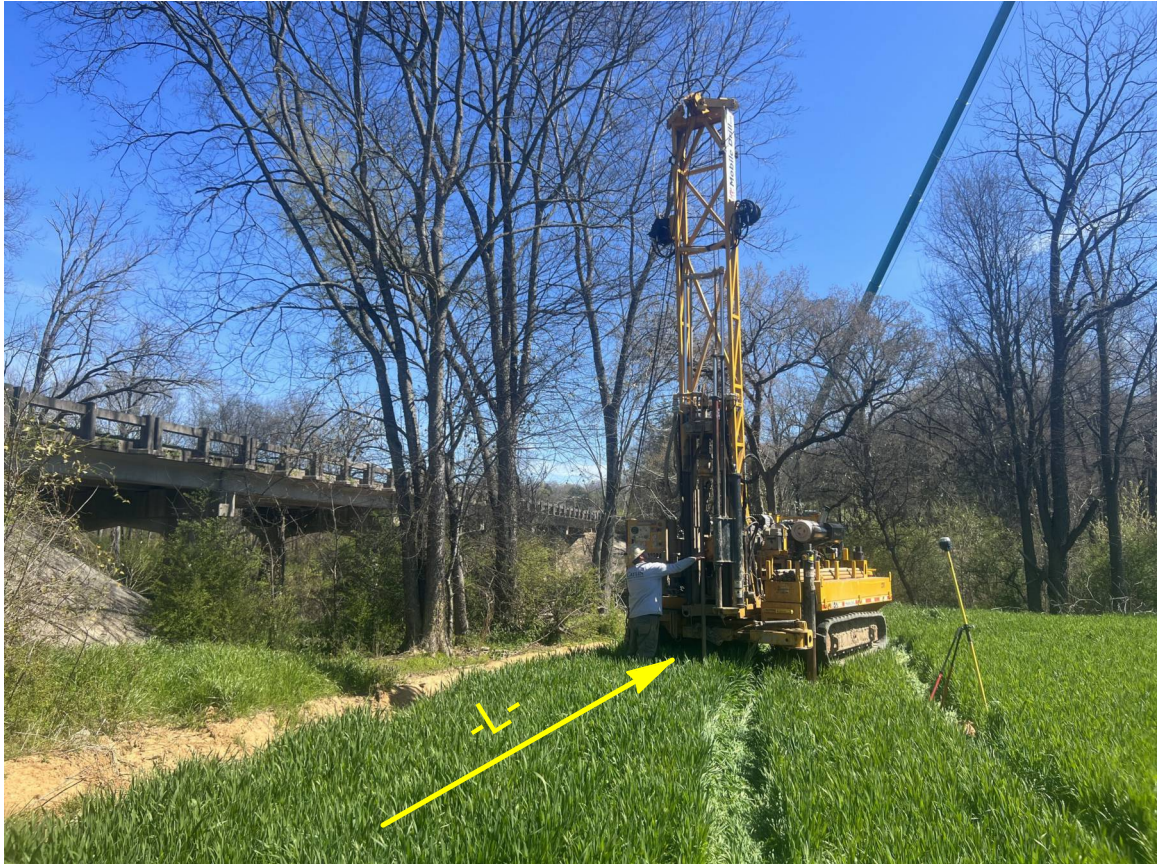
RIG ON EB1-C FACING UP STATION
