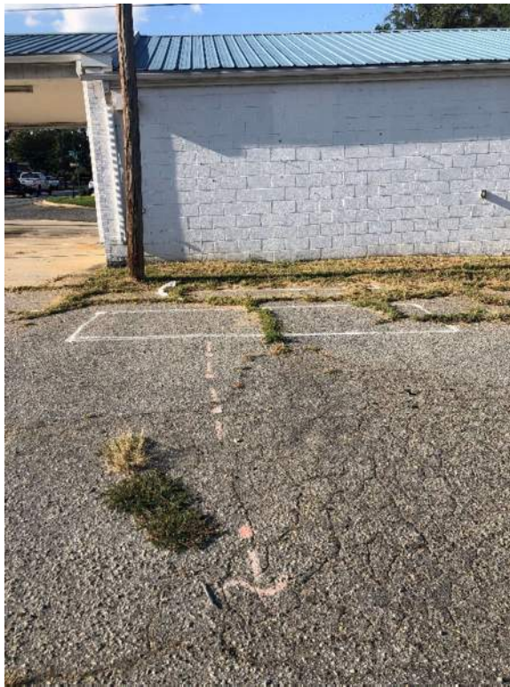
View of the two (2) probable orphan USTs located southwest of the vacant building on Parcel 22.
