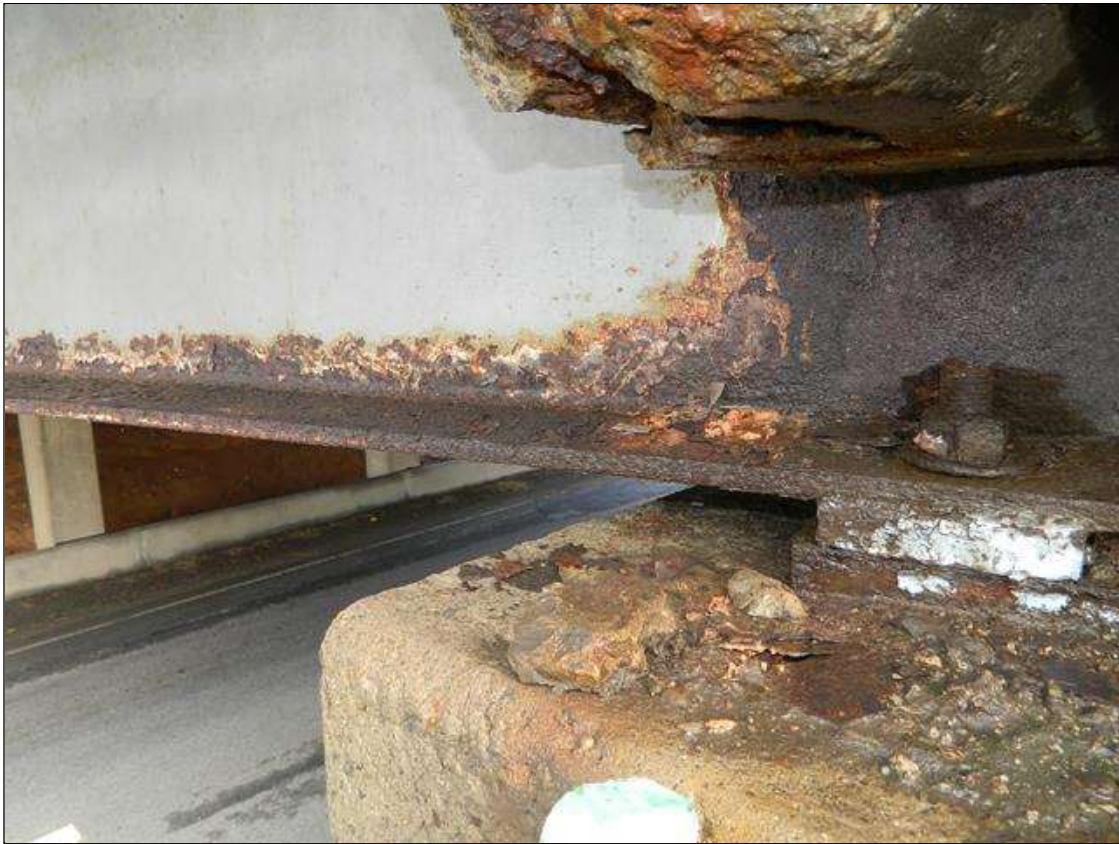
Span 2 Beam 10: THE FULL WIDTH OF THE BOTTOM FLANGE IS REDUCED TO 5/8" FOR 4' BEGINNING AT THE FAR END OF THE BEAM. THE LOWER 9" OF THE WEB IS REDUCED TO 3/8" - 7/16" FOR 1' BEGINNING AT THE FAR END OF THE BEAM. UPPER PORTION OF THE WEB IS NOT VISIBLE DUE TO END DIAPHRAGMS. ORIGINAL 11/16" FLANGE AND 1/2" WEB THICKNESSES. A PRIORITY MAINTENANCE IS REQUESTED.
