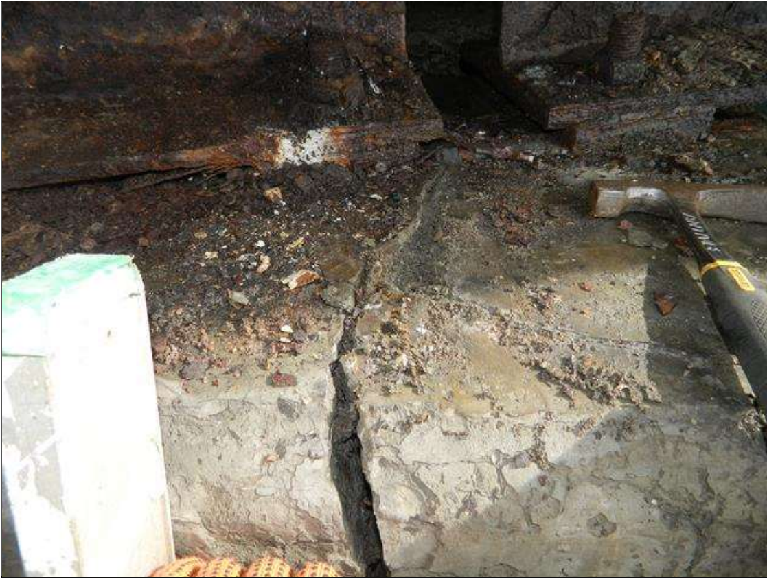
Bent 1 Cap 1: PATCH ON THE RIGHT END OF THE CAP HAS MULTIPLE CRACKS UP TO 1/2" WIDE THROUGHOUT ALL FACES AND THE END. THE PATCH IS DULL SOUNDING TO THE HAMMER, AND COULD EASILY BE KNOCKED LOOSE FROM THE CAP. LARGE PIECES OF THE PATCH HAVE ALREADY FALLEN OUT. A PRIORITY MAINTENANCE IS REQUESTED.
