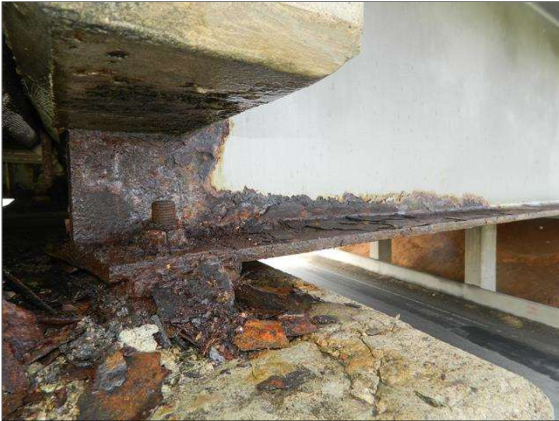
Span 2 Beam 1: THE FULL WIDTH OF THE BOTTOM FLANGE IS REDUCED TO 5/8" FOR 4' BEGINNING AT THE FAR END OF THE BEAM. THE LOWER 9" OF THE WEB IS REDUCED TO 3/8" - 7/16" FOR 1' BEGINNING AT THE FAR END OF THE BEAM. UPPER PORTION OF THE WEB IS NOT VISIBLE DUE TO END DIAPHRAGMS. ORIGINAL 11/16" FLANGE AND 1/2" WEB THICKNESSES. A PRIORITY MAINTENANCE IS REQUESTED.
