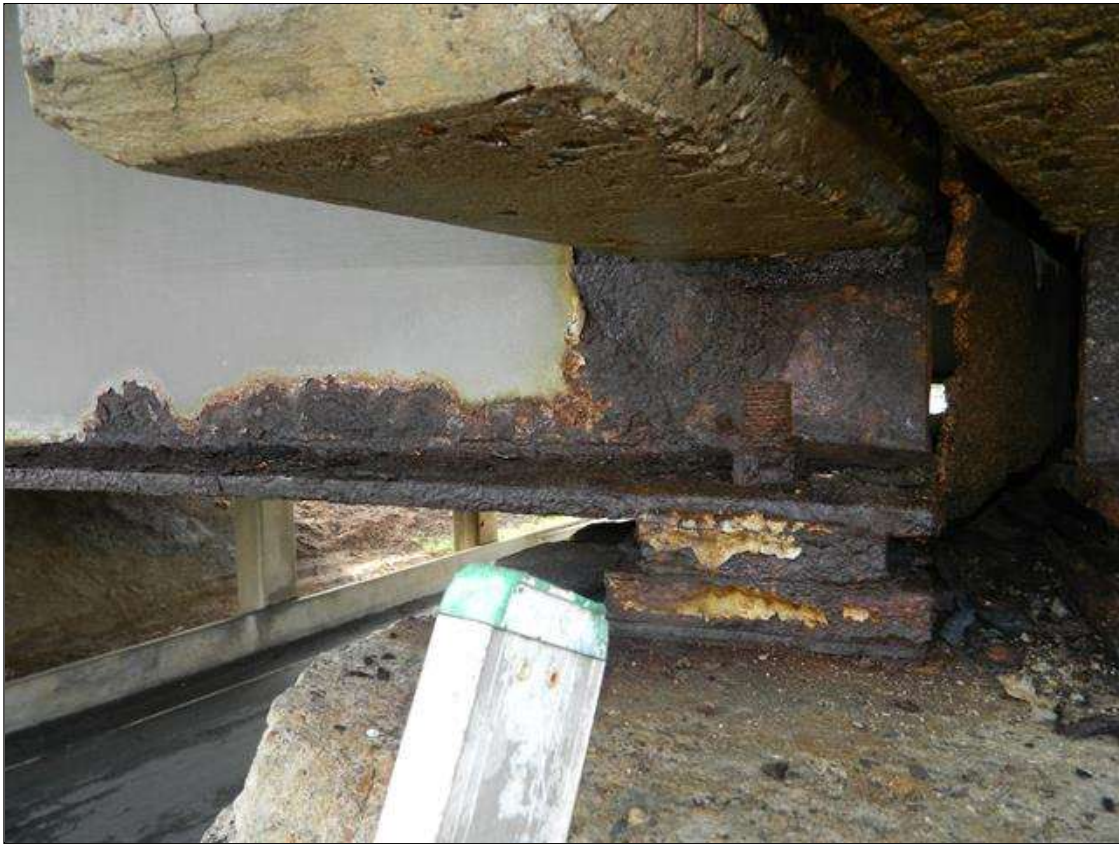
Span 2 Beam 1: THE FULL WIDTH OF THE BOTTOM FLANGE IS REDUCED TO 5/8" FOR 4' BEGINNING AT THE NEAR END OF THE BEAM. THE LOWER 9" OF THE WEB IS REDUCED TO 3/8" - 7/16" FOR 1' BEGINNING AT THE NEAR END OF THE BEAM. UPPER PORTION OF THE WEB IS NOT VISIBLE DUE TO END DIAPHRAGMS. ORIGINAL 11/16" FLANGE AND 1/2" WEB THICKNESSES. A PRIORITY MAINTENANCE IS REQUESTED.
