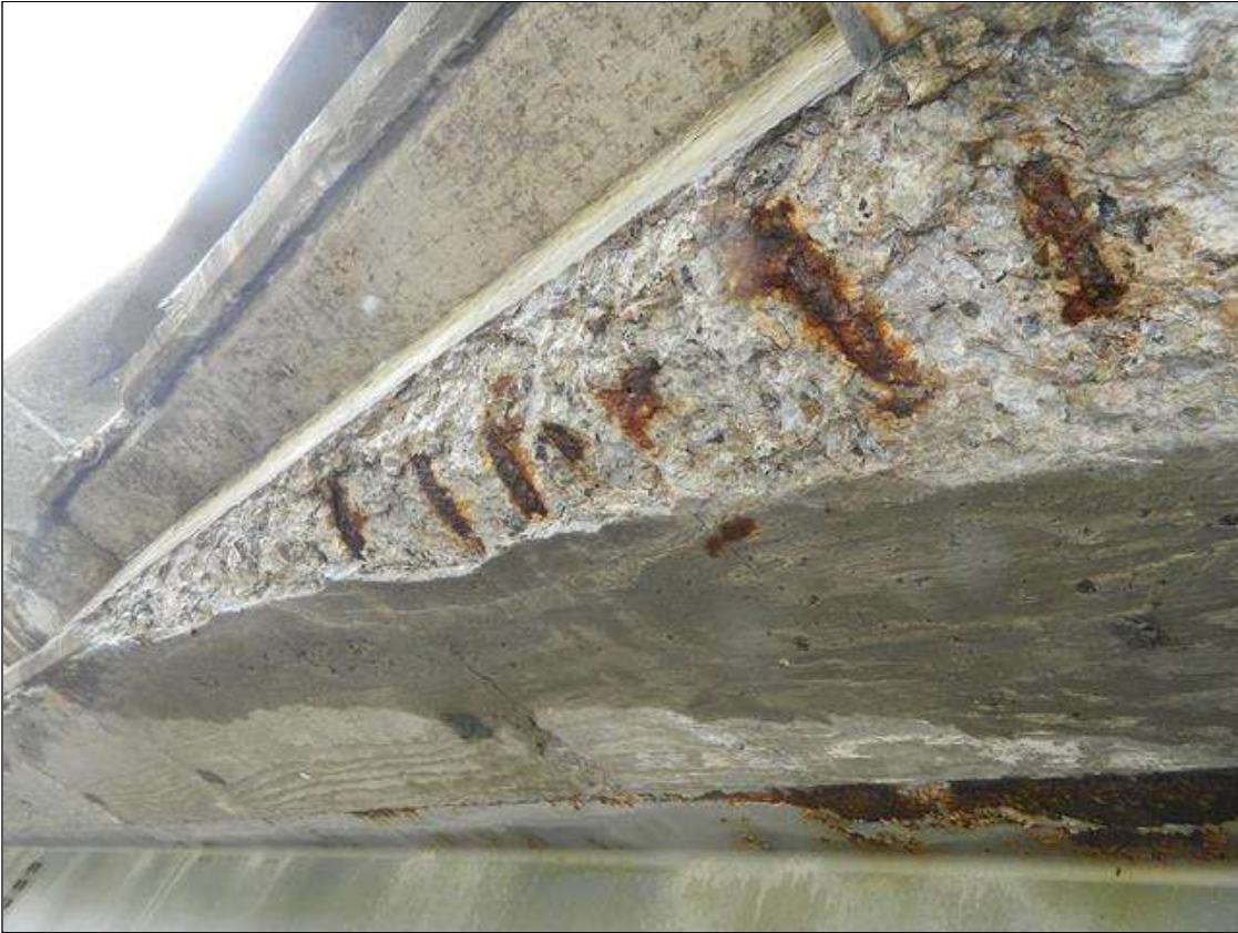
Span 3 Deck: 7' LONG X 1.5' WIDE X 2.5" DEEP DELAMINATION IN THE LEFT OVERHANG WITH EXPOSED AND CORRODING REINFORCING STEEL BEGINNING AT THE NEAR END OF THE SPAN. THE CURB, BEGINNING AT THE SAME AREA HAS 15' LONG FULL WIDTH X FULL HEIGHT X UP TO 3" DEEP DELAMINATION WITH EXPOSED AND CORRODING REINFORCING STEEL. A PRIORITY MAINTENANCE IS REQUESTED.
