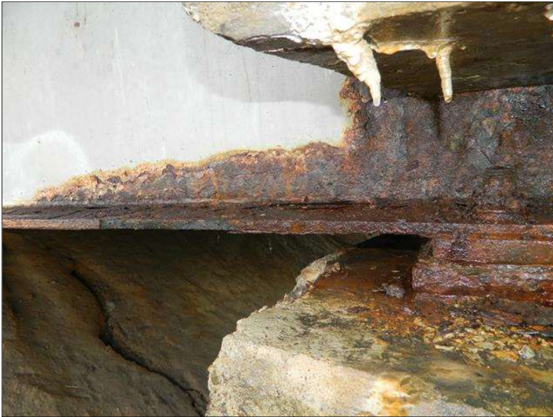
Span 3 Beam 1: THE FULL WIDTH OF THE BOTTOM FLANGE IS REDUCED TO 5/8" FOR 3' BEGINNING AT THE NEAR END OF THE BEAM. THE LOWER 9" OF THE WEB IS REDUCED TO 7/16" - 3/8" FOR 12" BEGINNING AT THE NEAR END OF THE BEAM. UPPER PORTION OF THE WEB IS NOT VISIBLE DUE TO END DIAPHRAGMS. ORIGINAL 11/16" FLANGE AND 1/2" WEB THICKNESSES. A PRIORITY MAINTENANCE IS REQUESTED.
