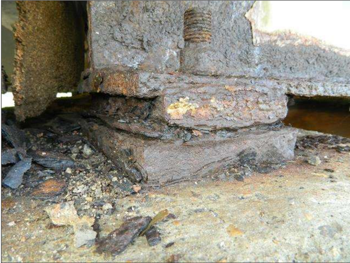
Span 1 Beam 1 Near Bearing: BEARING DEVICE CORRODED WITH 1/16" - 1/8" SCALE SECTION LOSS TO BOTH THE MASONRY AND SOLE PLATES. THE ANCHOR NUTS HAVE UP TO 75 PERCENT LOSS.
