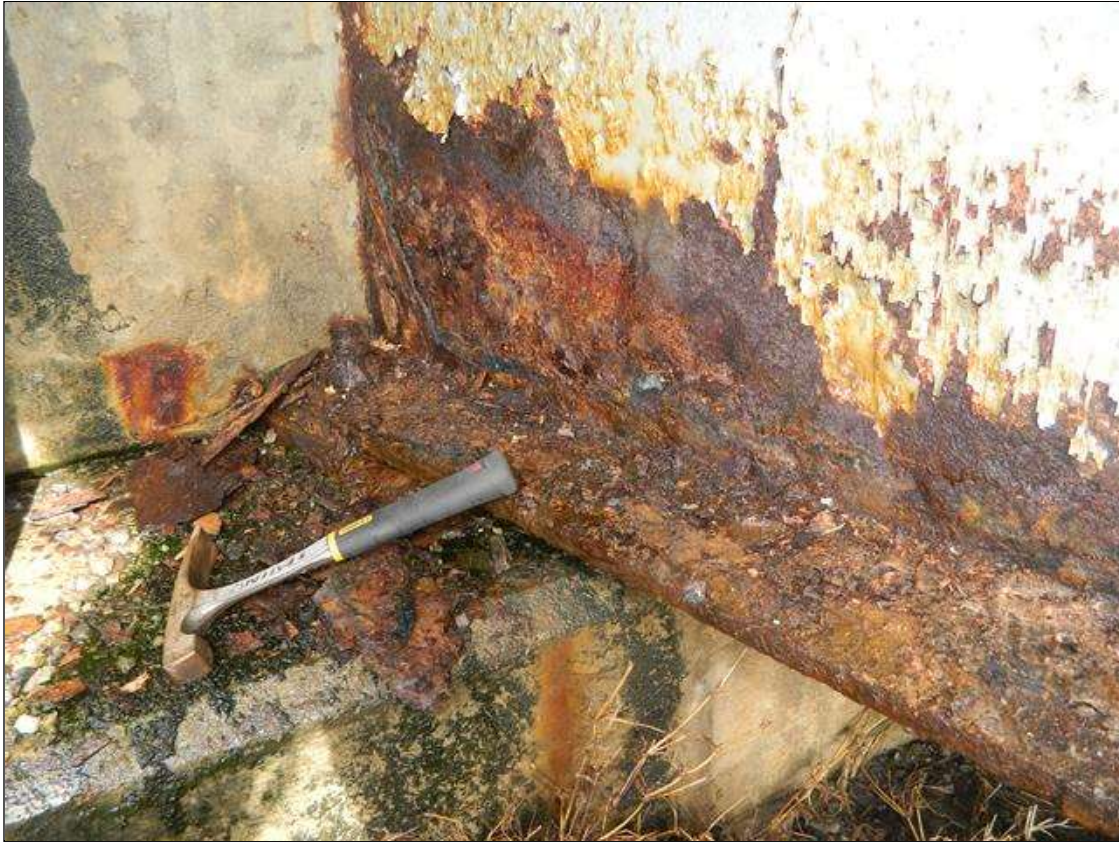
Span 1 Beam 10: THE FULL WIDTH OF THE BOTTOM FLANGE IS REDUCED TO 9/16'' - 5/8'' FOR 4' BEGINNING AT THE NEAR END OF THE BEAM. THE LOWER 16" OF THE WEB IS REDUCED TO 1/4'' - 5/16'' FOR 2' BEGINNING AT THE NEAR END OF THE BEAM. ORIGINAL 11/16'' FLANGE AND 1/2'' WEB THICKNESSES. A PRIORITY MAINTENANCE IS REQUESTED.
