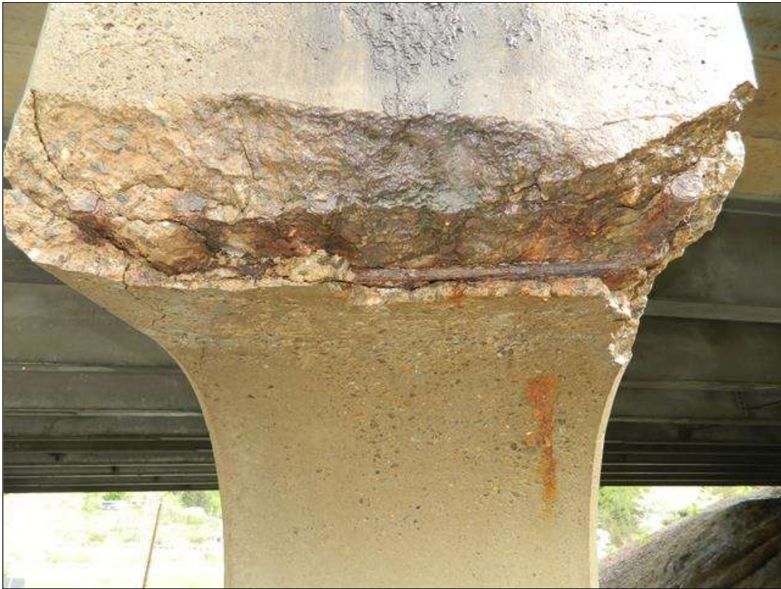
Bent 2 Cap 1: THE RIGHT END OF THE CAP HAS A FULL WIDTH X 3' LONG SPALL UP TO 3" DEEP WITH EXPOSED AND CORRODING REINFORCING STEEL TO THE UNDERSIDE OF THE CAP AND THE END OF THE CAP. MULTIPLE CRACKS UP TO 1/2" WIDE IN THE TOP FACE OF THE CAP, AND ALONG THE TOP EDGE OF THE CAP IN THE EAST FACE EXTENDING UNDERNEATH BEAM 10, AND UP TO BEAM 9. A PRIORITY MAINTENANCE IS REQUESTED.
