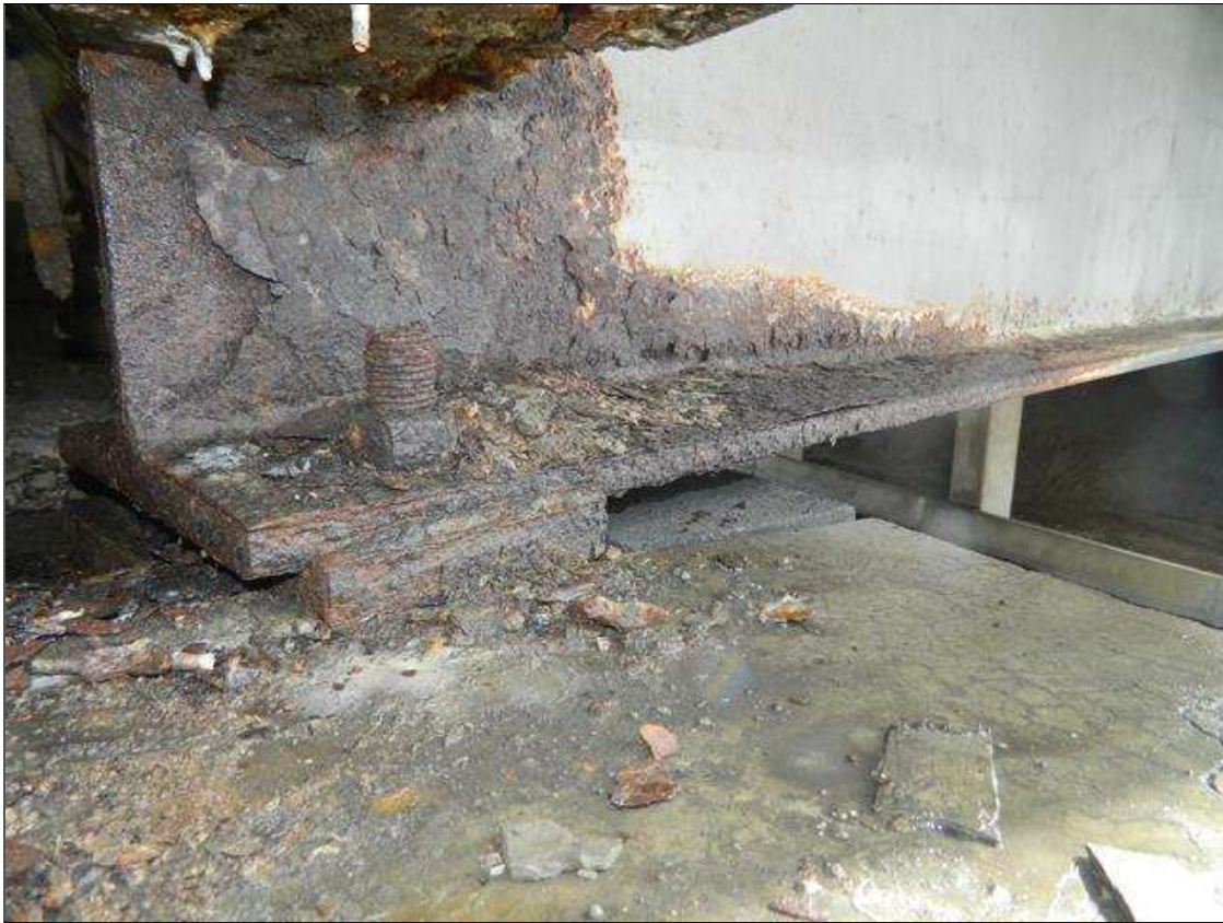
Span 2 Beam 10: THE FULL WIDTH OF THE BOTTOM FLANGE IS REDUCED TO 5/8" FOR 3.5' BEGINNING AT THE NEAR END OF THE BEAM. THE LOWER 9" OF THE WEB IS REDUCED TO 3/8" - 7/16" FOR 1' BEGINNING AT THE NEAR END OF THE BEAM. UPPER PORTION OF THE WEB IS NOT VISIBLE DUE TO END DIAPHRAGMS. ORIGINAL 11/16" FLANGE AND 1/2" WEB THICKNESSES. A PRIORITY MAINTENANCE IS REQUESTED.
