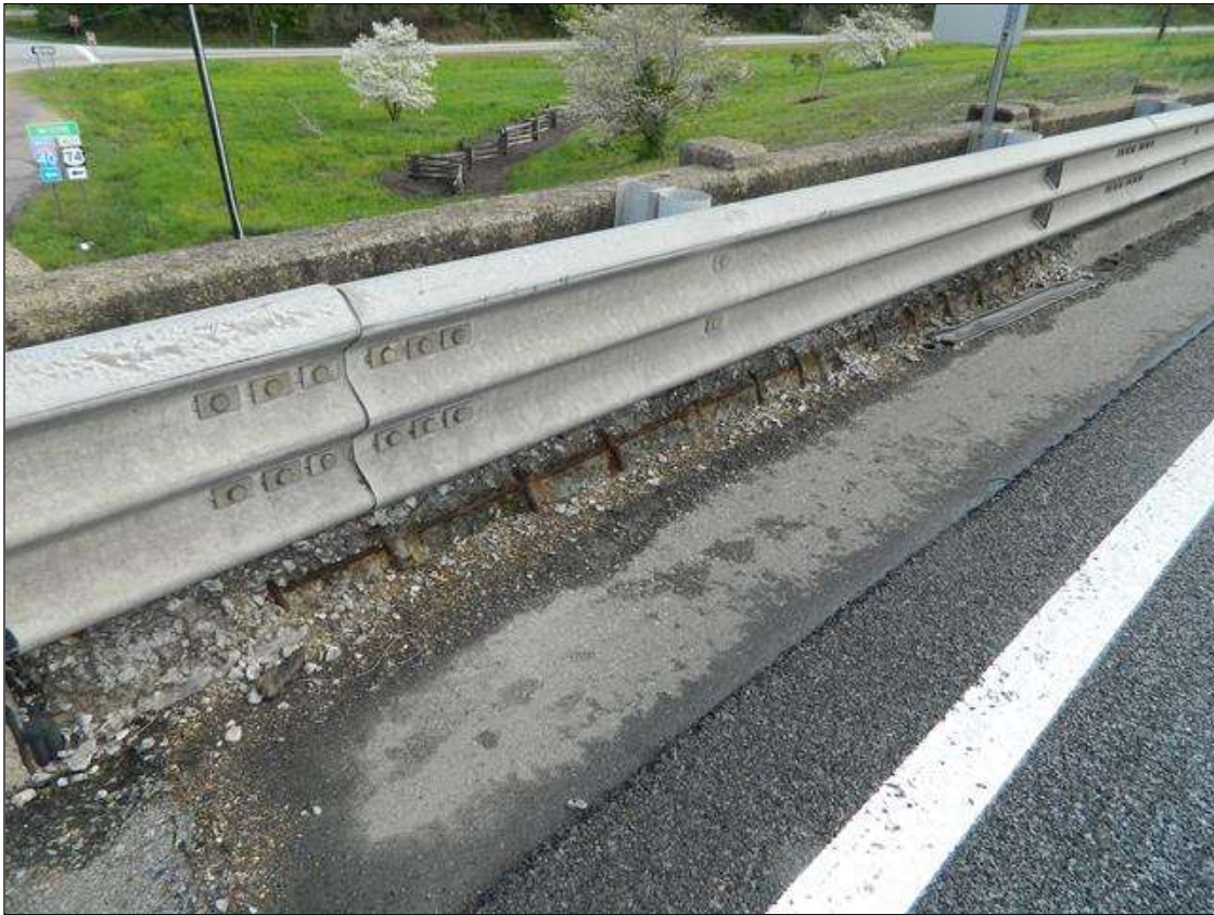
Span 3 Deck: 7' LONG X 1.5' WIDE X 2.5" DEEP DELAMINATION IN THE LEFT OVERHANG WITH EXPOSED AND CORRODING REINFORCING STEEL BEGINNING AT THE NEAR END OF THE SPAN. THE CURB, BEGINNING AT THE SAME AREA HAS 15' LONG FULL WIDTH X FULL HEIGHT X UP TO 3" DEEP DELAMINATION WITH EXPOSED AND CORRODING REINFORCING STEEL. A PRIORITY MAINTENANCE IS REQUESTED.
