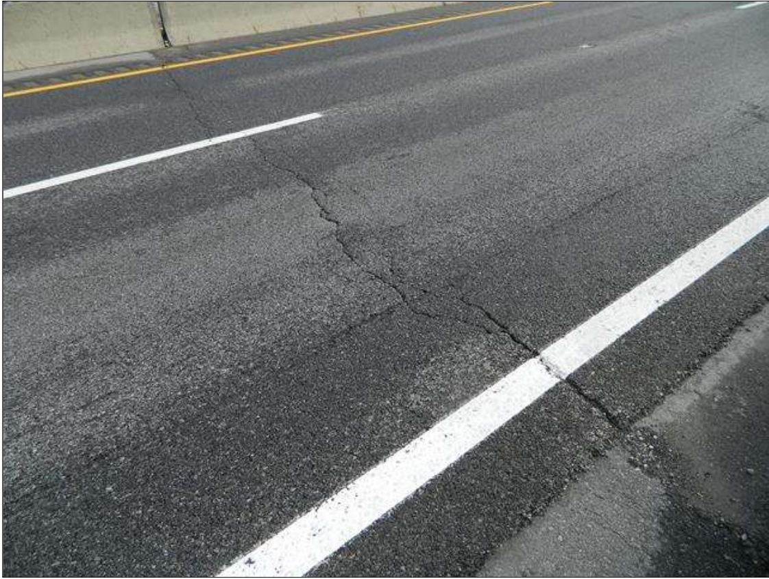
Span 1 Wearing Surface: 1/4" - 1/2" WIDE TRANSVERSE CRACKS AT THE EXPANSION JOINTS.
