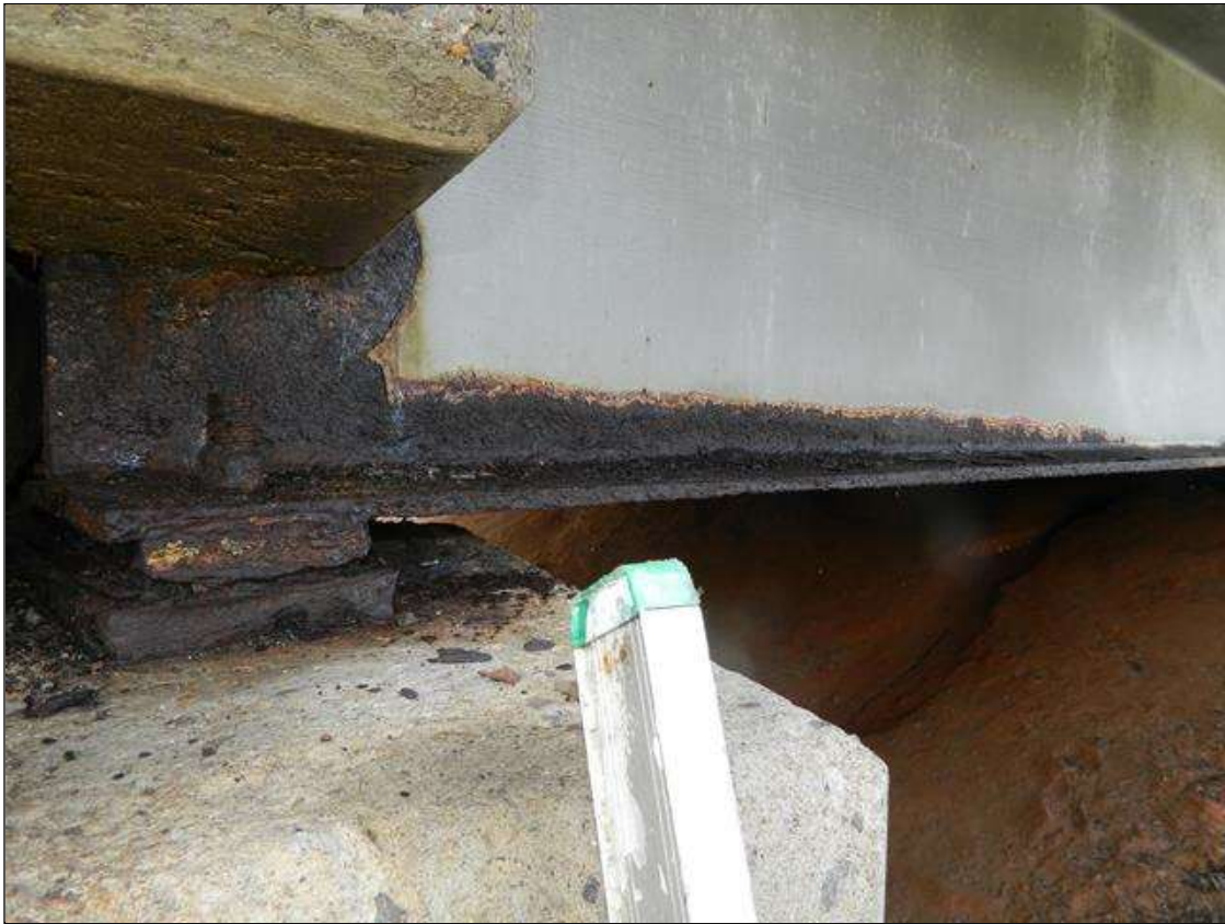
Span 1 Beam 1: THE FULL WIDTH OF THE BOTTOM FLANGE IS REDUCED TO 1/2" FOR 4' BEGINNING AT THE FAR END OF THE BEAM, AND 5/8" FOR 1' ADJACENT TO PREVIOUS LOSS. THE LOWER 9" OF THE WEB IS REDUCED TO 3/8" FOR 1.5' BEGINNING AT THE FAR END OF THE BEAM. UPPER PORTION OF THE WEB IS NOT VISIBLE DUE TO END DIAPHRAGMS. ORIGINAL 11/16" FLANGE AND 1/2" WEB THICKNESSES. A PRIORITY MAINTENANCE IS REQUESTED.
