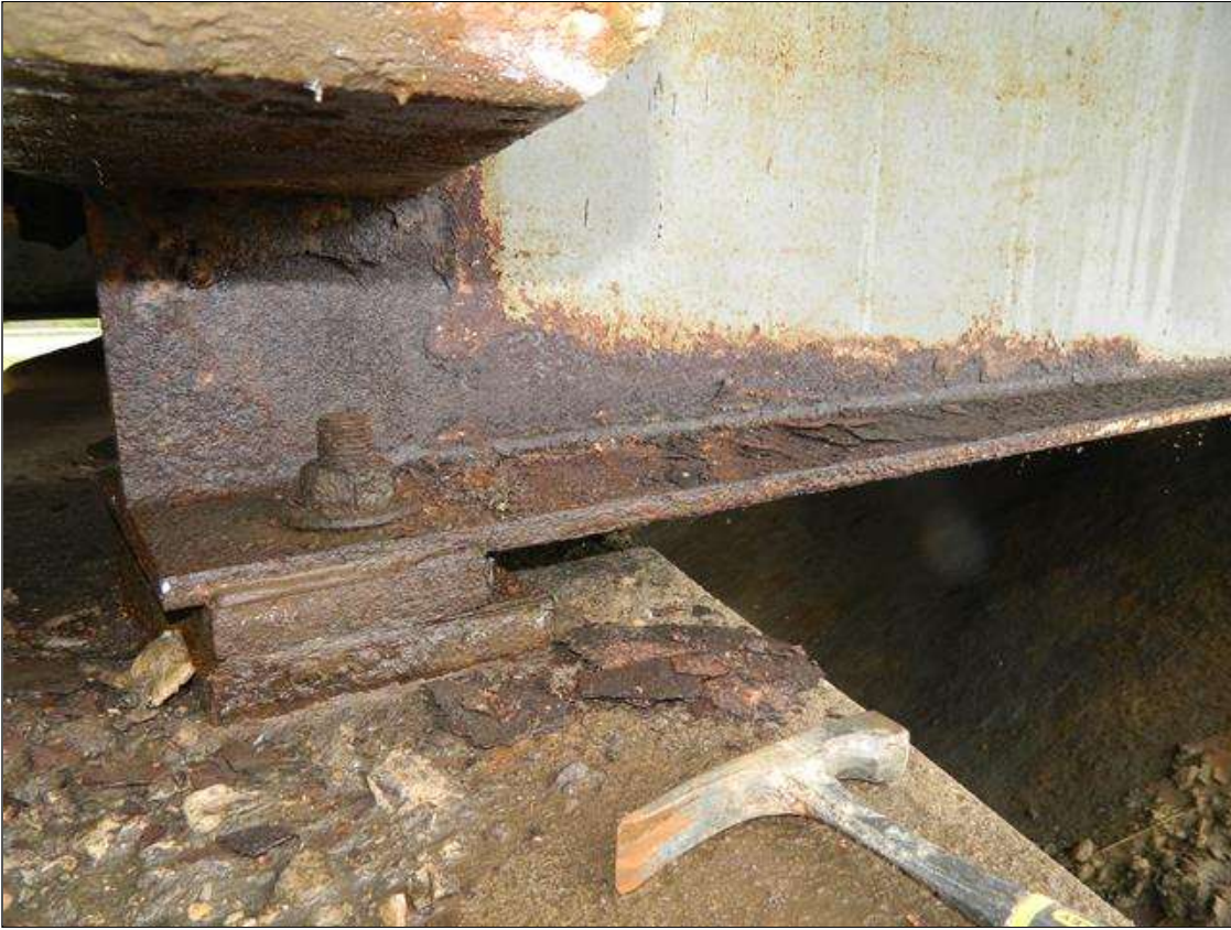
Span 3 Beam 10: THE FULL WIDTH OF THE BOTTOM FLANGE IS REDUCED TO 5/8" FOR 3' BEGINNING AT THE NEAR END OF THE BEAM. THE LOWER 9" OF THE WEB IS REDUCED TO 7/16" - 3/8" FOR 12" BEGINNING AT THE NEAR END OF THE BEAM. UPPER PORTION OF THE WEB IS NOT VISIBLE DUE TO END DIAPHRAGMS. ORIGINAL 11/16" FLANGE AND 1/2" WEB THICKNESSES. A PRIORITY MAINTENANCE IS REQUESTED.
