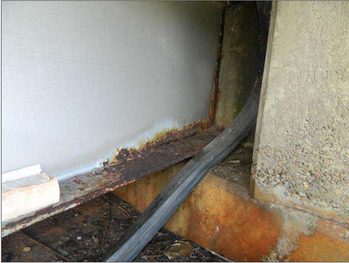
Span 1 Beam 1: THE FULL WIDTH OF THE BOTTOM FLANGE IS REDUCED TO 5/8" FOR 4' BEGINNING AT THE NEAR END OF THE BEAM. THE LOWER 6" OF THE WEB IS REDUCED TO 3/8" - 7/16" FOR 1' BEGINNING AT THE NEAR END OF THE BEAM. ORIGINAL 11/16" FLANGE AND 1/2" WEB THICKNESSES. A PRIORITY MAINTENANCE IS REQUESTED.
